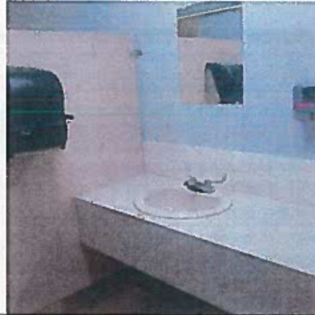
Washroom finishes are tired and are not accessible.
