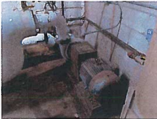
Many of the ice plant components appear to be very old and should be reviewed.
