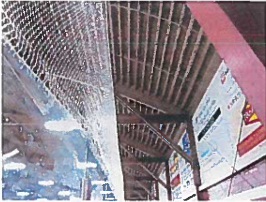
The existing wood beams and purlins appear to be in good condition.
