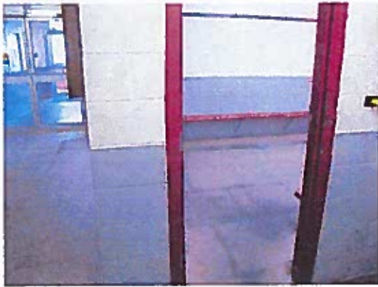
Doorways are narrow and not compliant with current OBC standards.
