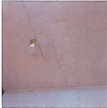
Ceiling tiles in the community hall are damaged, either the result of a roofing problem or the result of condensation.
