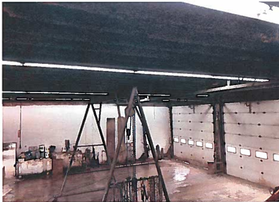
Photo 6: View from Second Floor Looking into Garage, Gantry Crane in View, Coated Double Tees at Roof Level. Wall in Background Separates the Existing from Garage Addition
