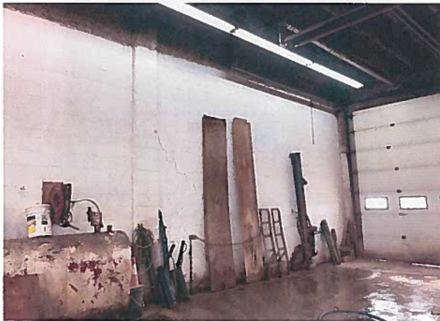
Photo 12: Crack in Concrete Block Wall Near Central Pier
