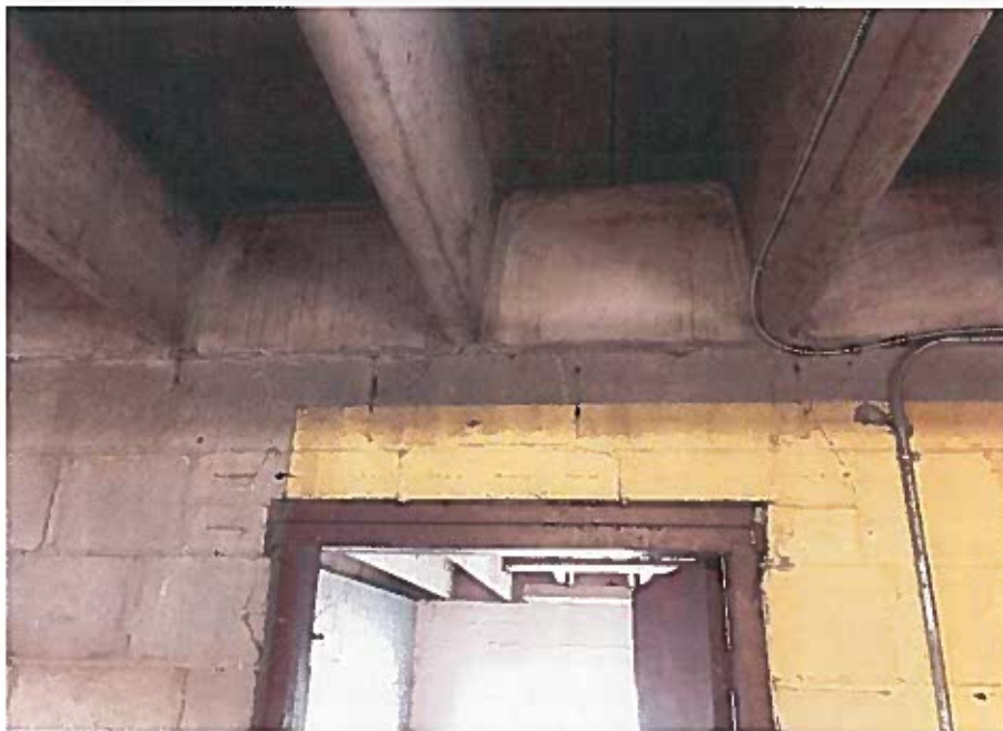
Photo 8: Cracks Through Block Lintel Above Second Floor Door
