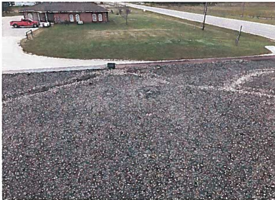
Photo 20: Minor “Trenching” or Roof Gravel to Direct Water to Edge Scupper, Likely to Reduce Water Ponding
