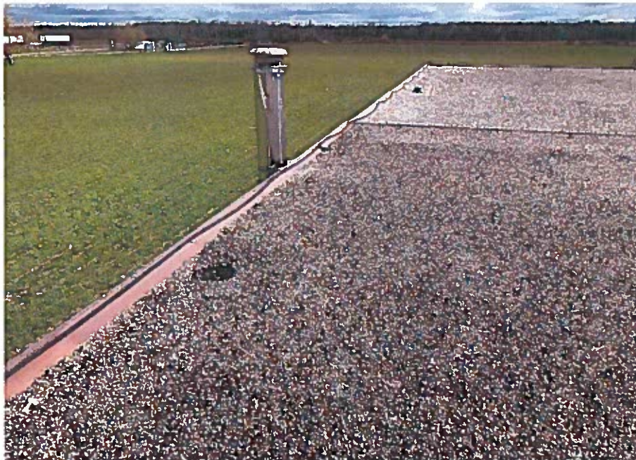
Photo 18: Roof Drain with Missing Filter Basket
