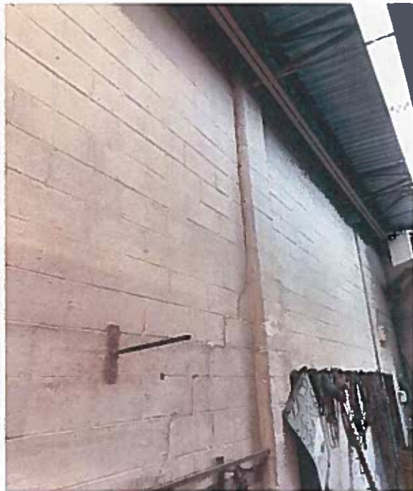
Photo 16: Crack in Concrete Block Wall on Addition Side. Joists Parallel to Wall, Block Wall Carries Little Vertical Weight
