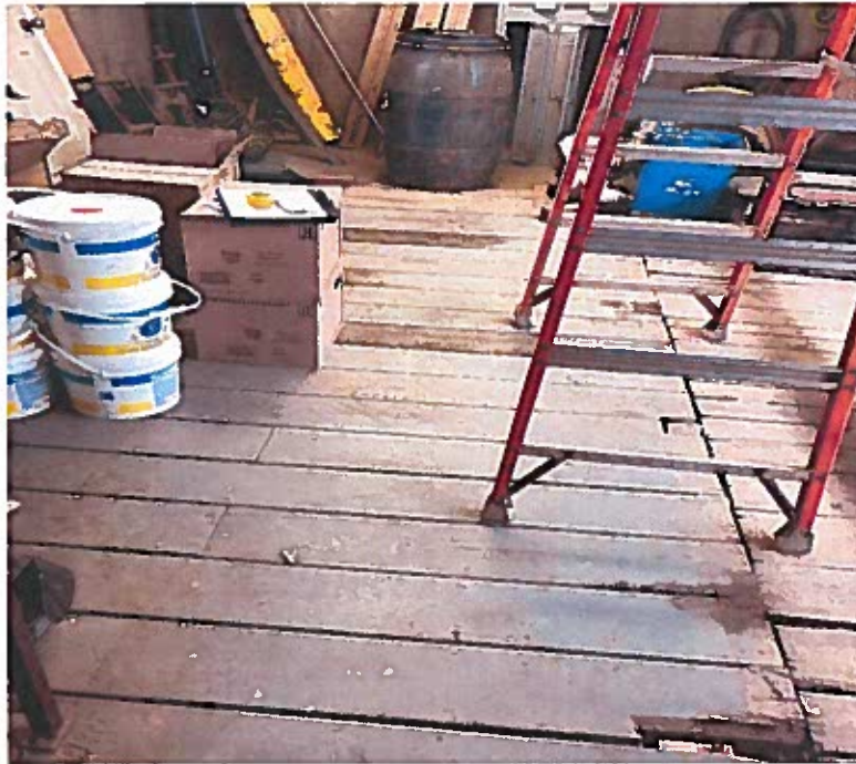
Photo 10: Wood Decking Second Floor in Fair Condition
