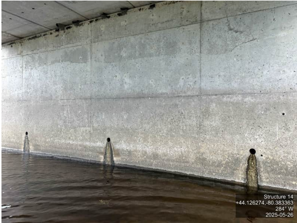
ABUTMENT WALLS – SOUTH – COLD JOINT
