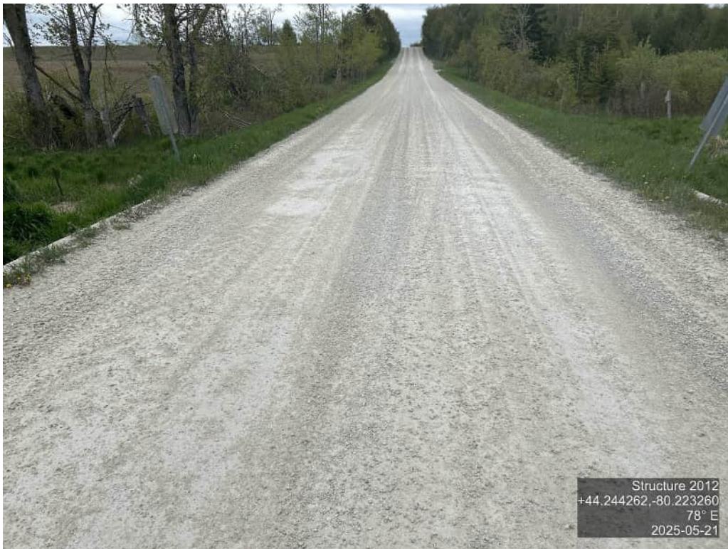
DECK WEARING SURFACE – EAST – MODERATE POTHOLES
