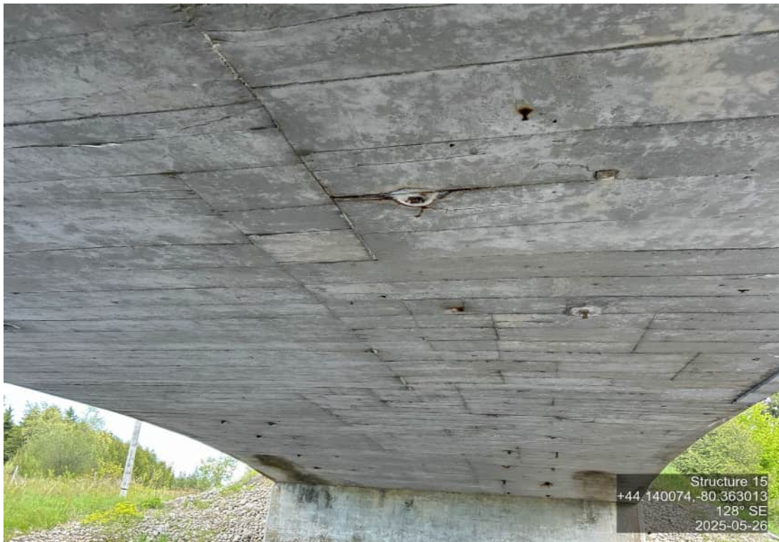
SOFFIT- INTERIOR - LIGHT DELAMINATIONS
