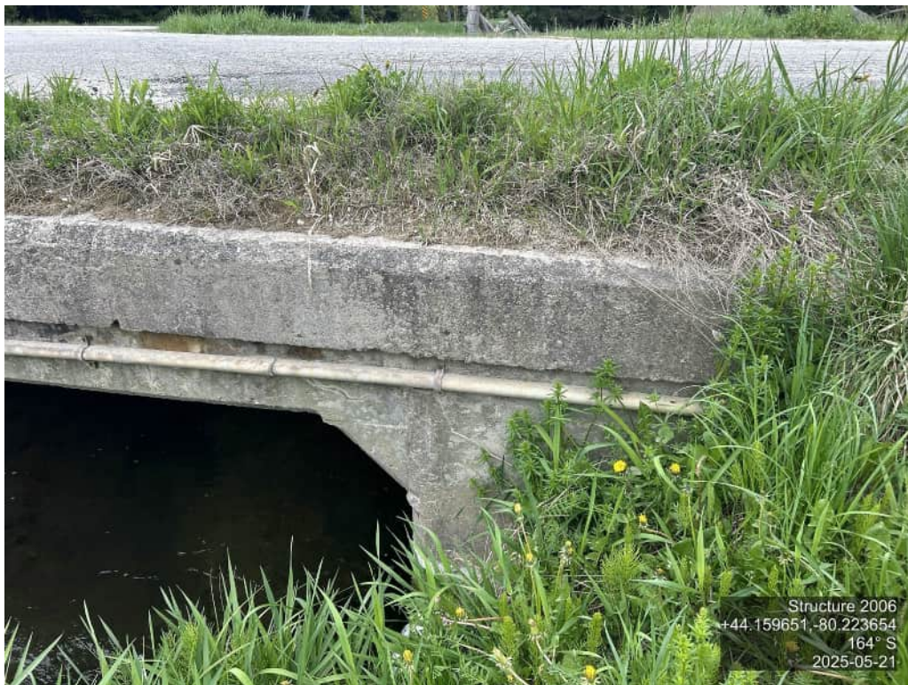
WINGWALL – SOUTH – NARROW STAINED CRACKS
