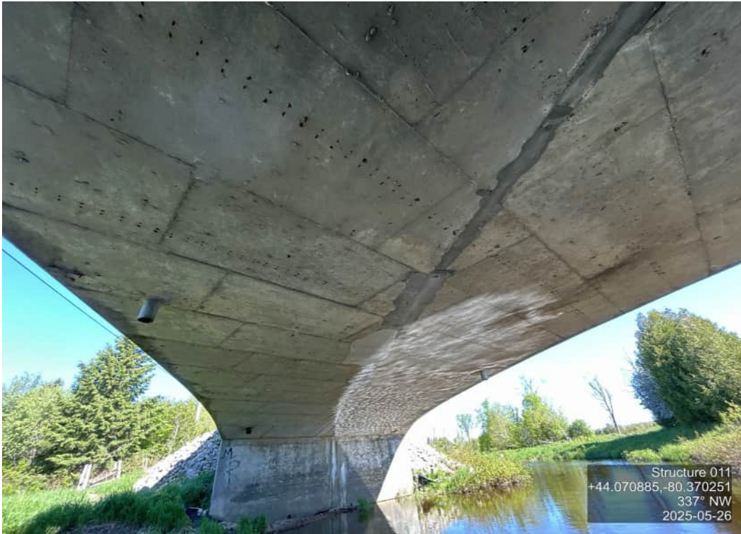
SOFFIT INTERIOR – NORTHWEST – WIDE CRACK PATCHED IN 2022 REHAB
