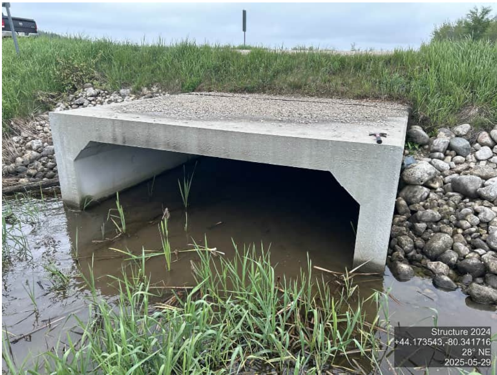
INLET – EAST – HAIRLINE STAINED CRACKS
