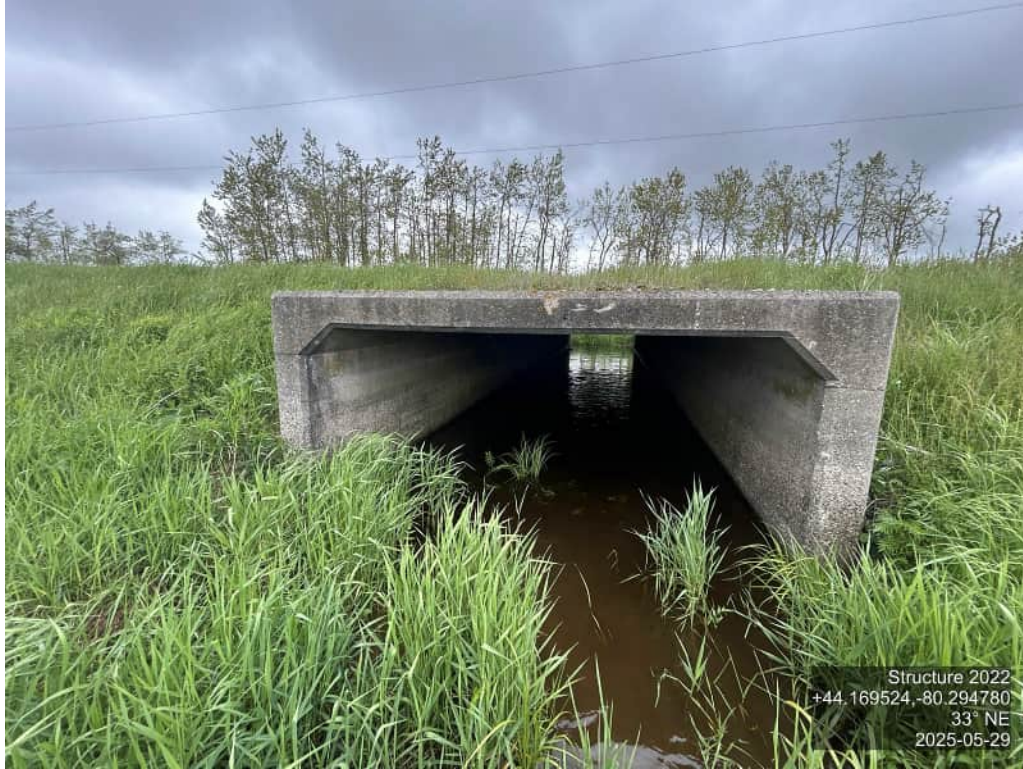
OUTLET – SOUTH – SCALING AND HAIRLINE CRACKS
