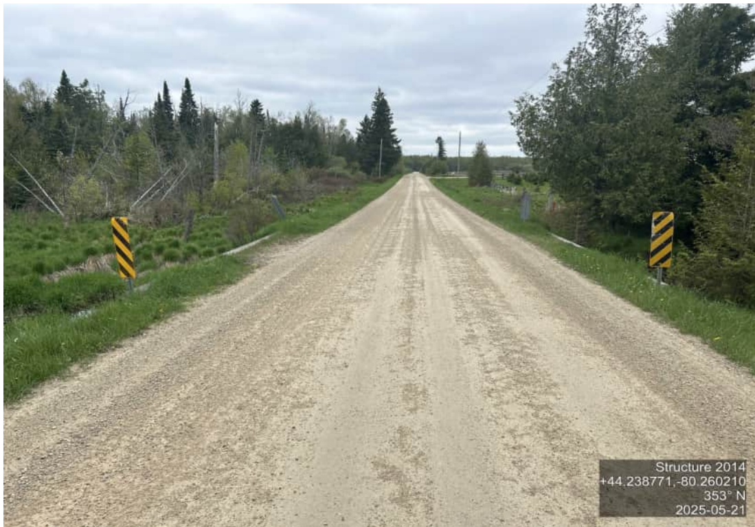
DECK WEARING SURFACE – NORTH – SMALL POTHOLES
