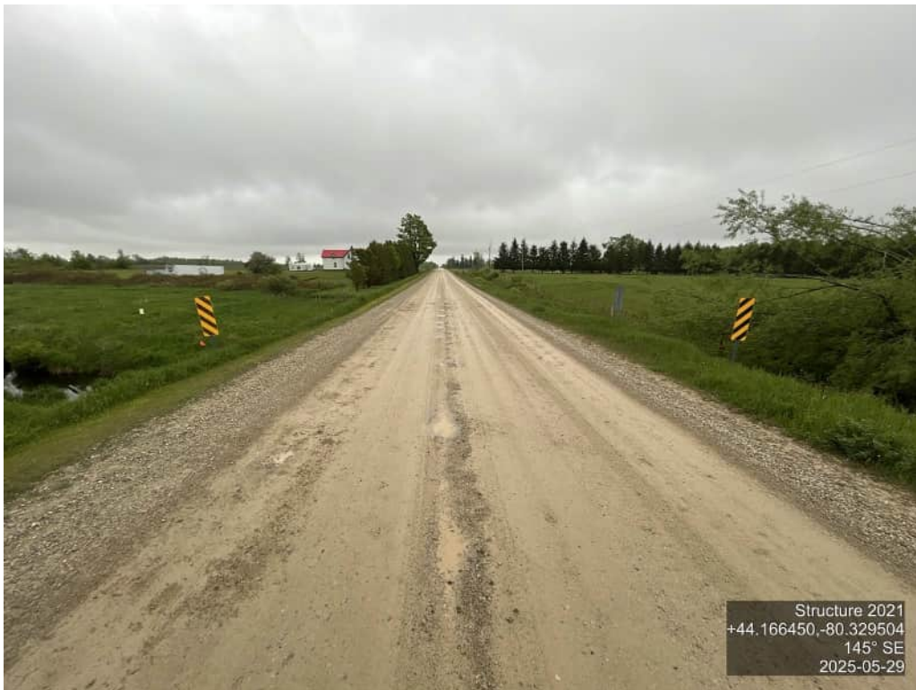
DECK WEARING SURFACE – NORTH – SMALL POTHoles AND MINOR RUTTING
