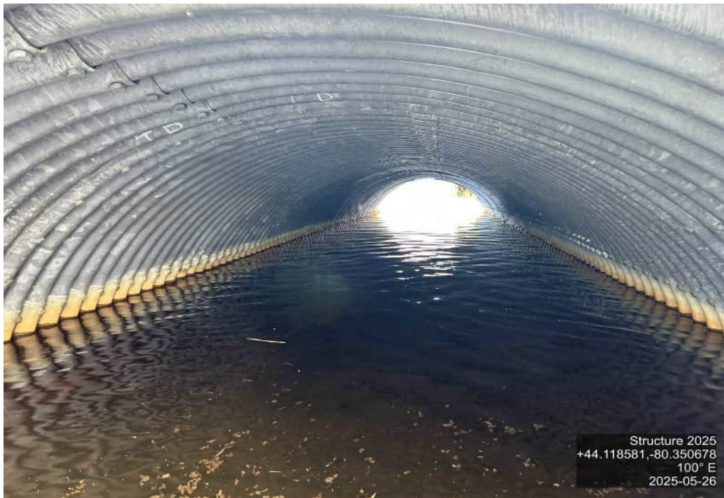
BARREL – SOUTH – MODERATE TO SEVERE CORROSION UP TO SPRING LINE, PERFORATIONS ON CULVERT FLOOR AND SECTION LOSS ALONG ENTIRE FLOOR
