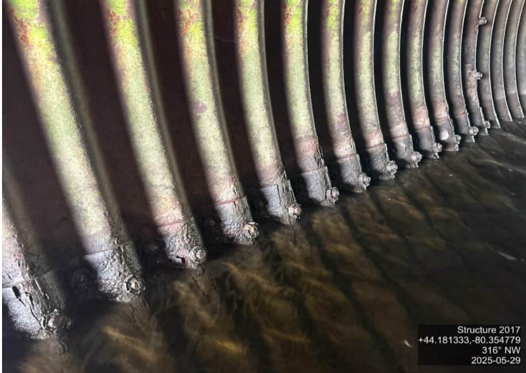
BARREL – NORTHWEST – SEVERE CORROSION, FLAKING AND SECTION LOSS ALONG WATERLINE
