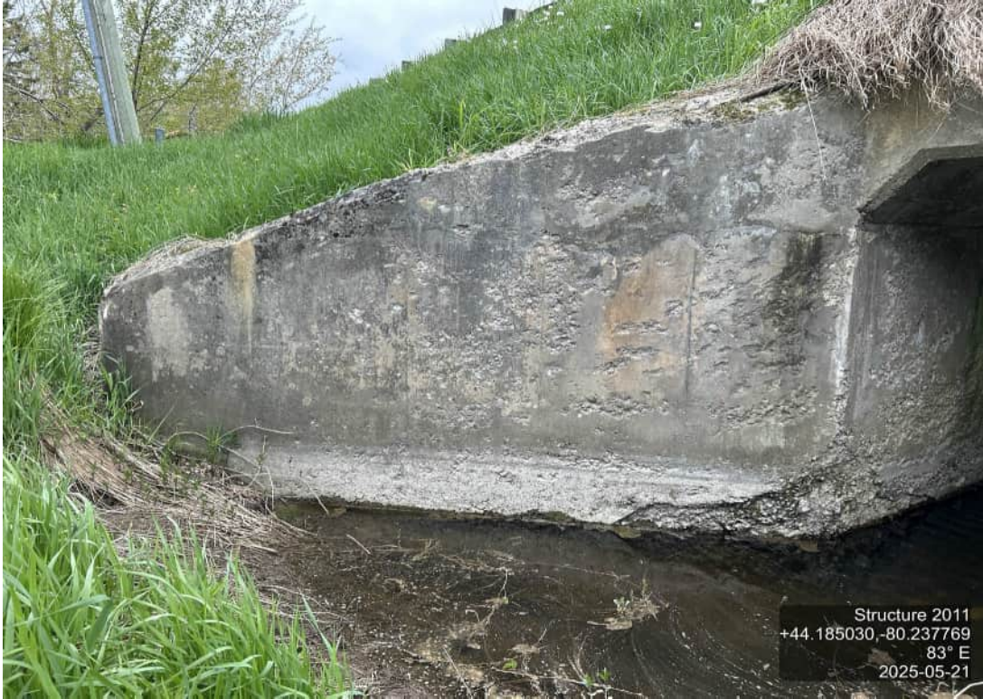
WINGWALL – SOUTHEAST – SEVERE SCALING, DELAMINATIONS AND SPALL WITH EXPOSED CORRODED REBAR
