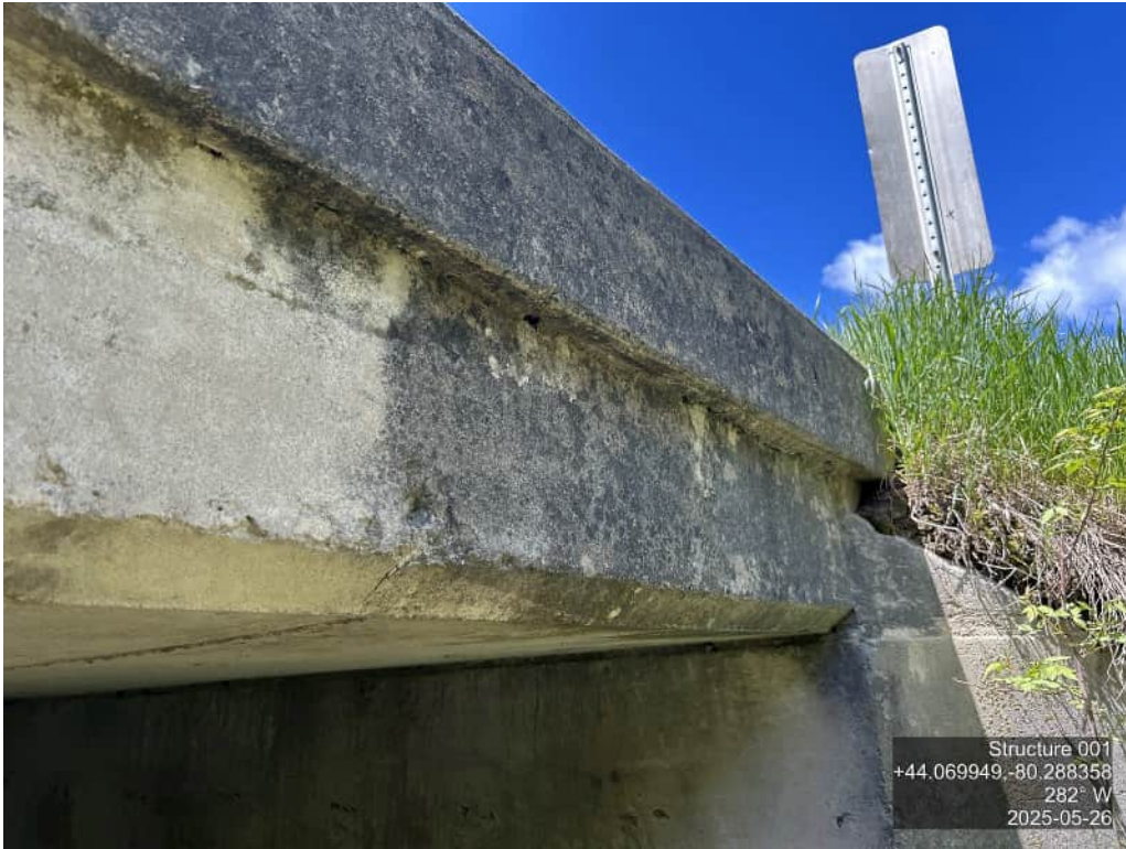
SOFFIT EXTERIOR – EAST – EFFLORESCENCE STAINED CRACKING
