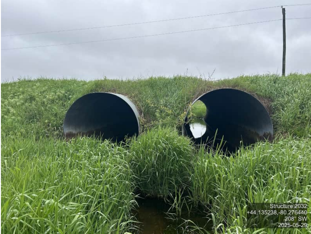
STREAM – EAST – AGGRADATION PARTIALLY BLOCKING NORTH BARREL
