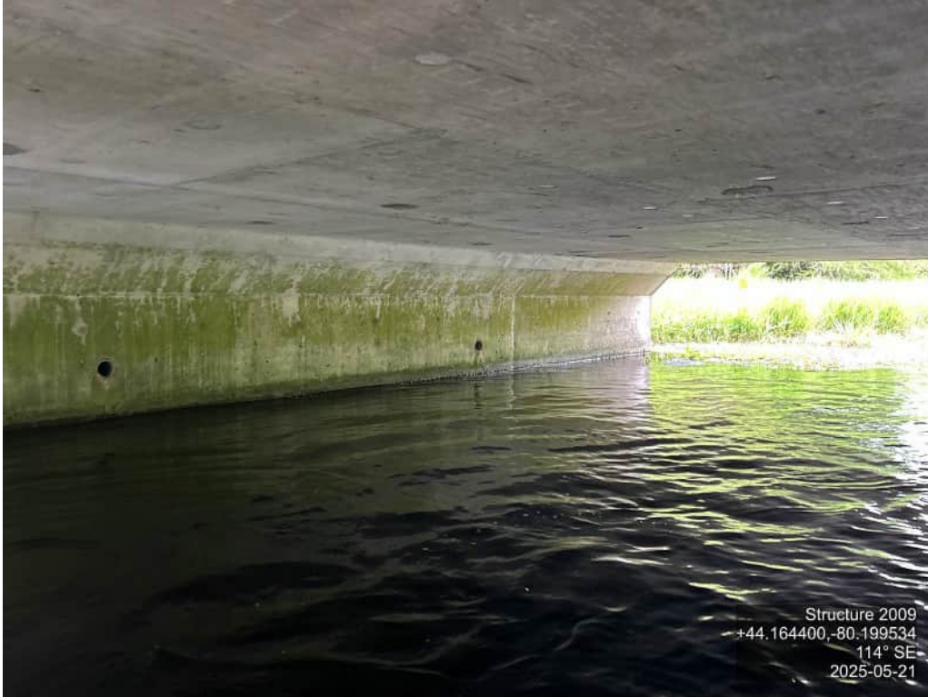
BARREL – INTERIOR – DAMPNESS NOTED
