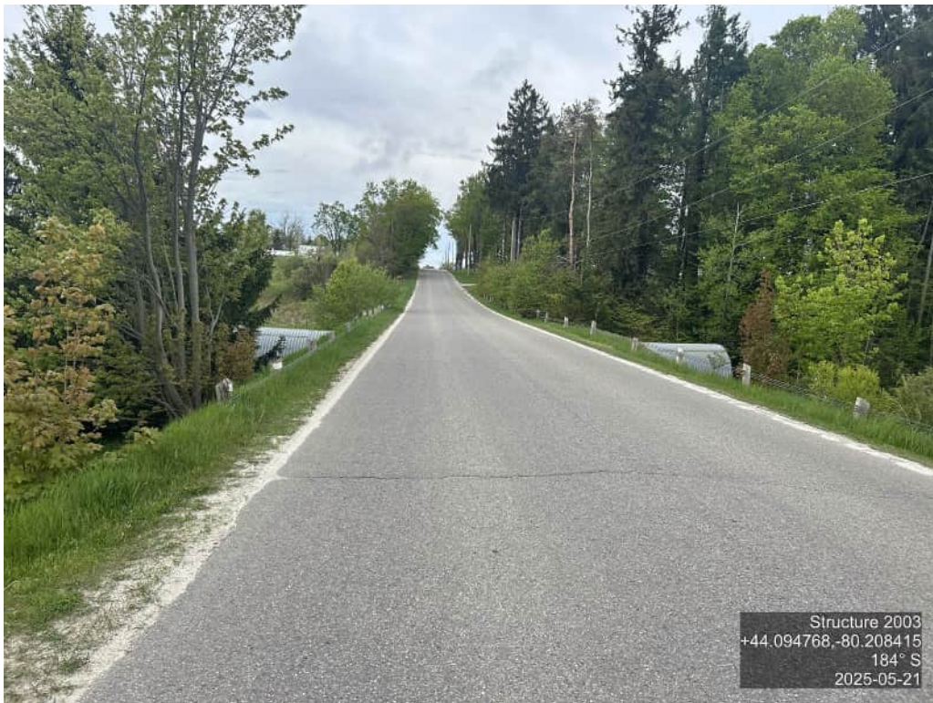
DECK WEARING SURFACE – NORTH – NARROW FULL WIDTH TRANSVERSE CRACK
