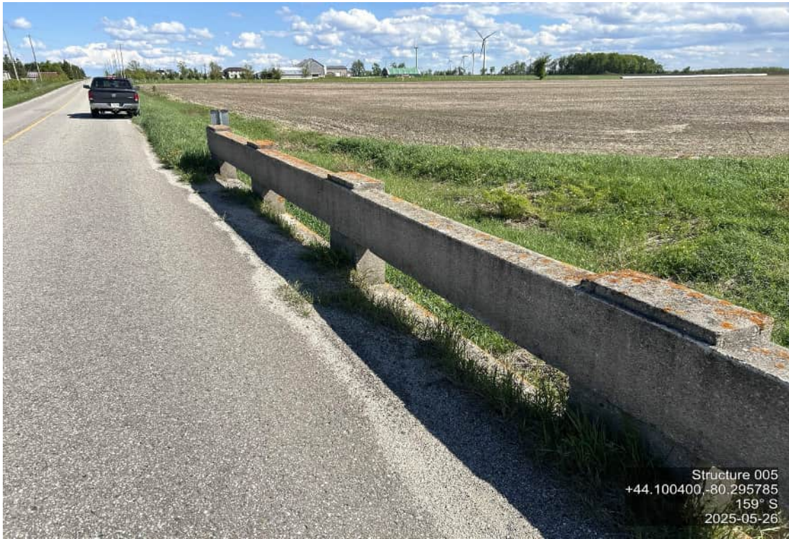
RAILING SYSTEM – EAST – APPEARS TO BE TOO LOW
