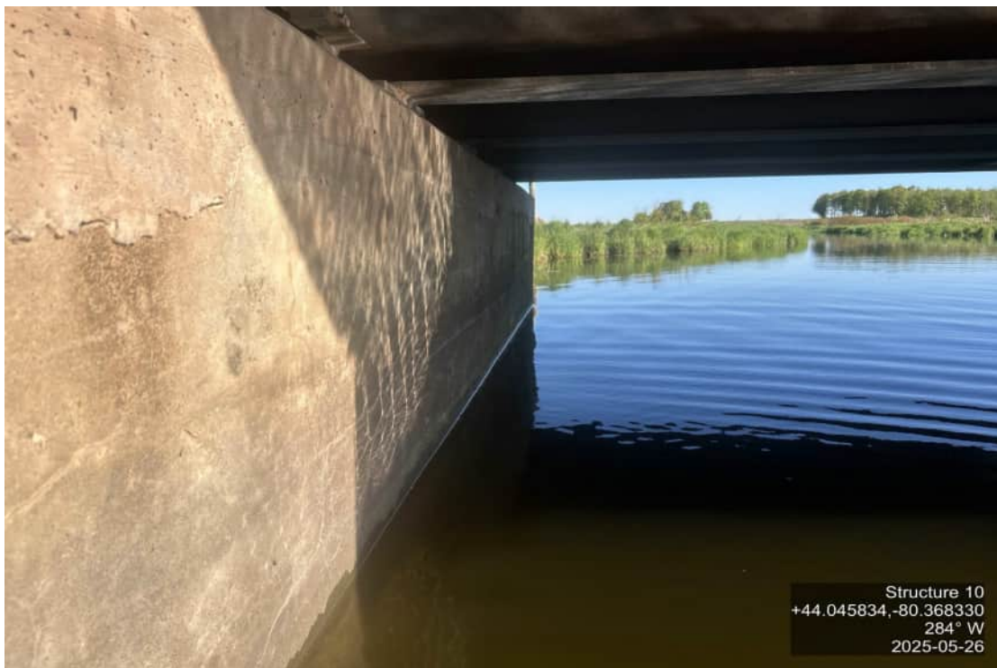
ABUTMENT WALLS – WEST – HAIRLINE TO MEDIUM CRACKING THROUGHOUT
