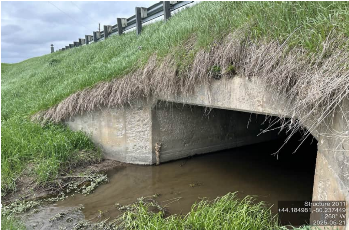
SOFFIT – EXTERIOR – SPALLING WITH EXPOSED CORRODED REBAR AND DELAMINATIONS
