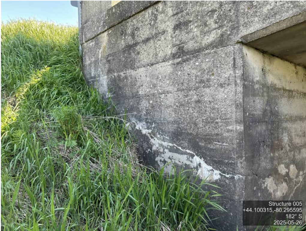
WINGWALLS – SOUTHEAST – EFFLORESCENCE STAINING
