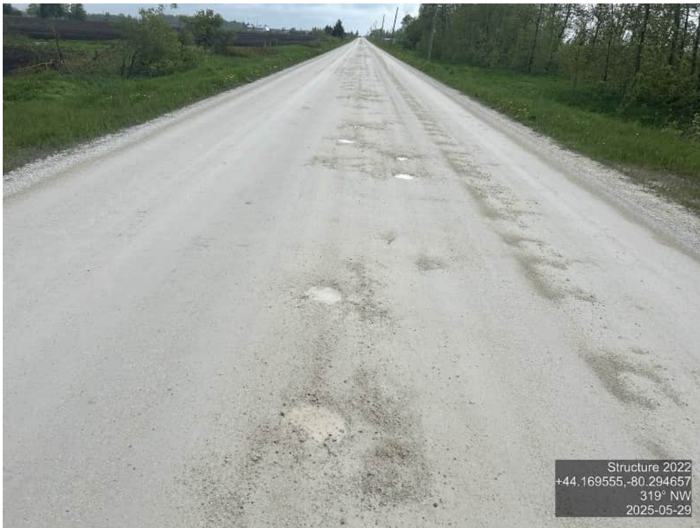
DECK WEARING SURFACE – NORTH – SMALL POTHoles
