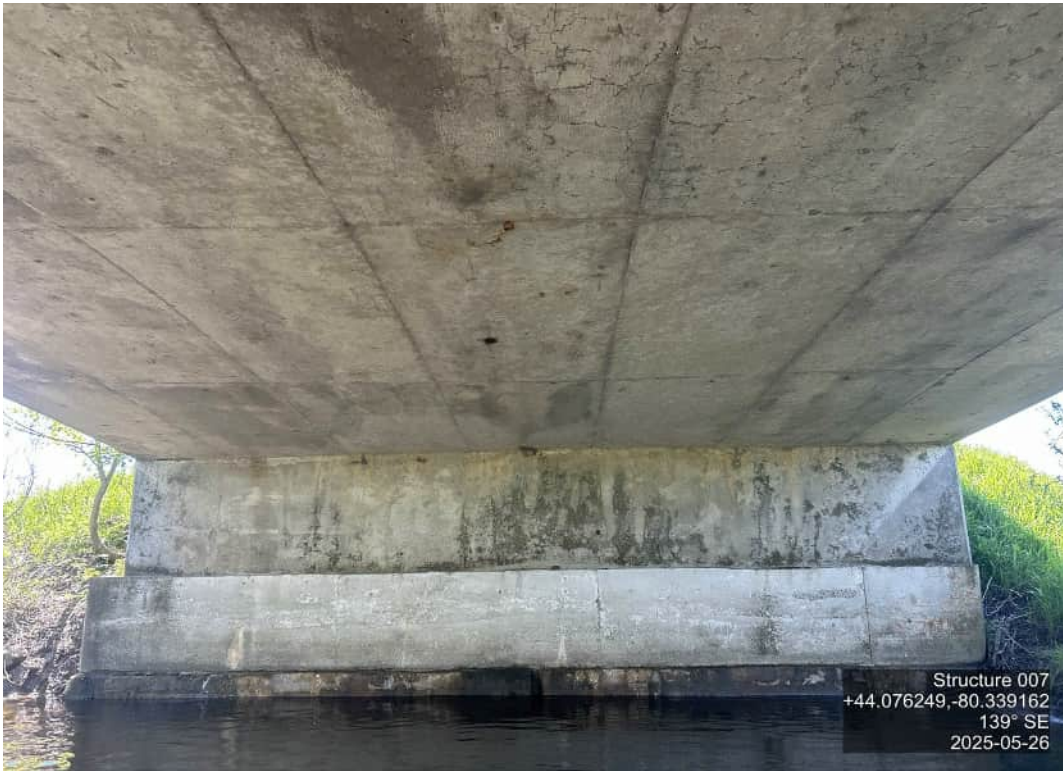
SOFFIT INTERIOR – INTERIOR – PATTERN CRACKING AND FULL SPAN WIDE CRACK IN CENTER
