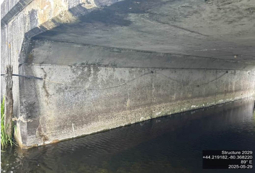
ABUTMENT WALLS – INSIDE WALLS – TWO VERTICAL SHRINKAGE CRACKS IN EACH WALL AND HONEYCOMBING
