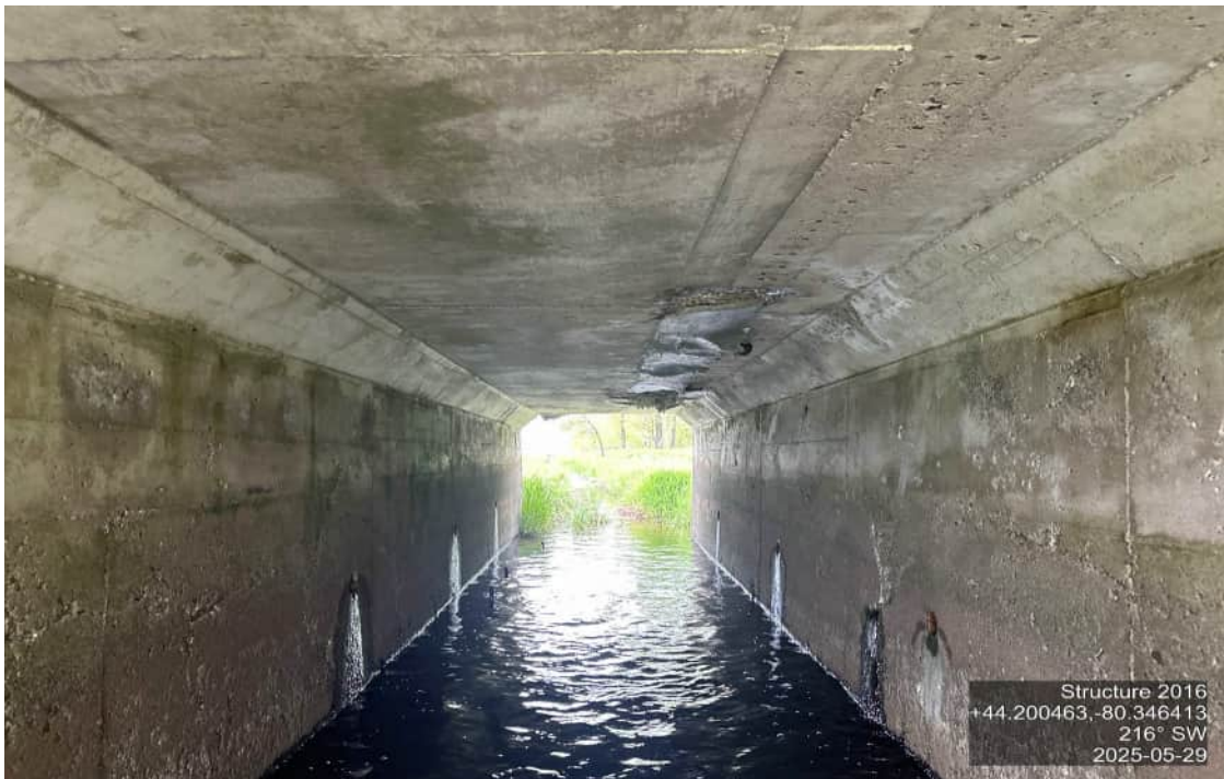
ABUTMENT WALLS – INTERIOR – SPALLS WITH EXPOSED CORRODED REBAR AND COLD JOINTS ON BOTH WALLS
