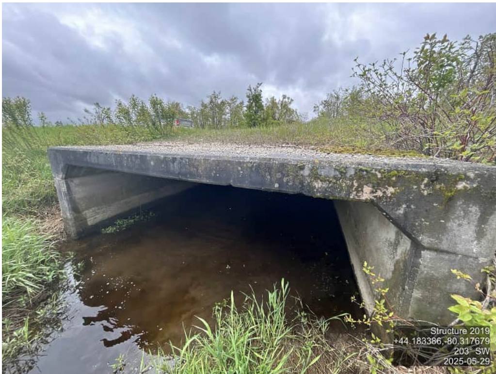
INLET – NORTH – SMALL SPALL AND WATER STAINING
