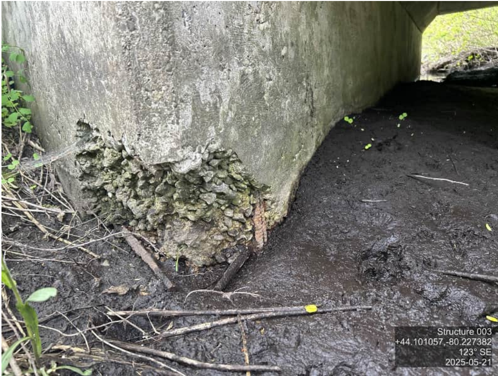
ABUTMENT – EAST – SCOUR AT CORNER
