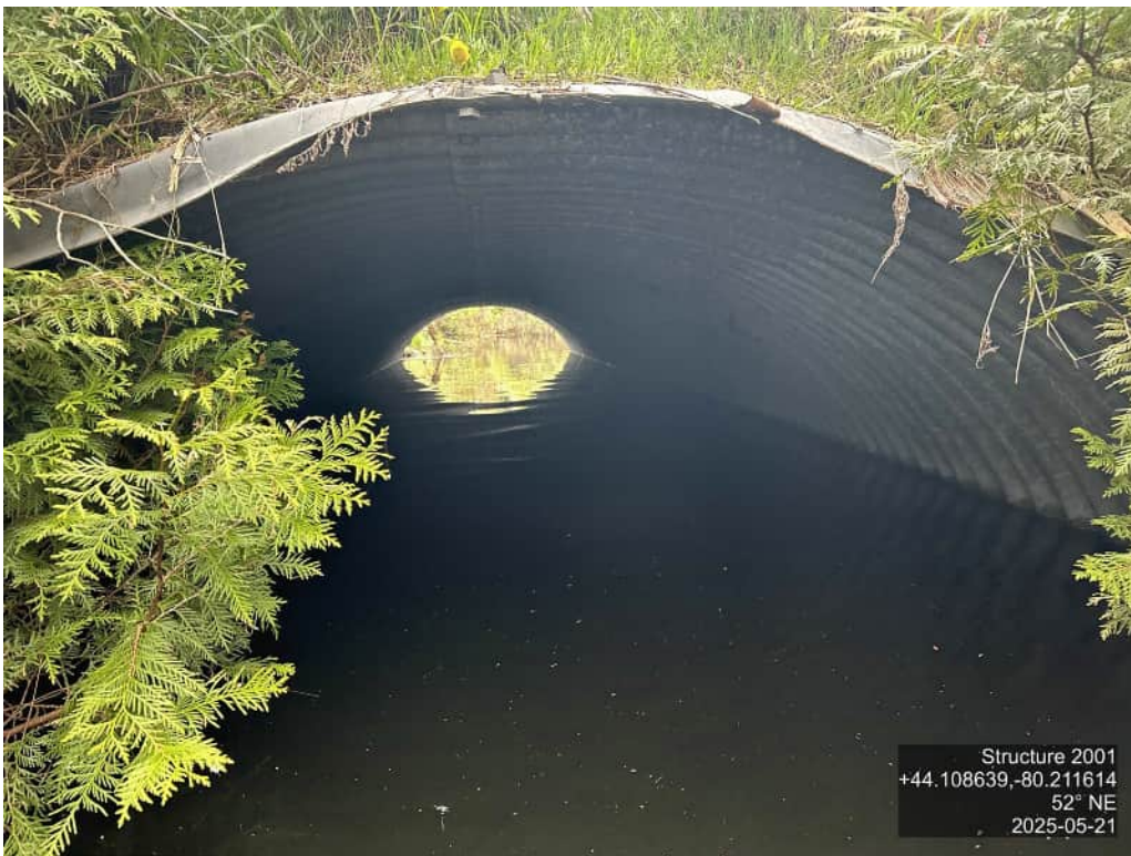
BARREL – INSIDE WALLS – LIGHT CORROSION, FLAKING AND LIGHT BULGING
