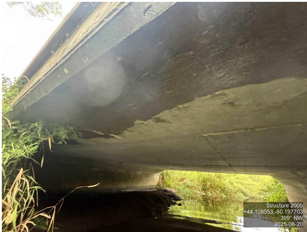
SOFFIT EXTERIOR – EAST – DAMPNESS NOTED
