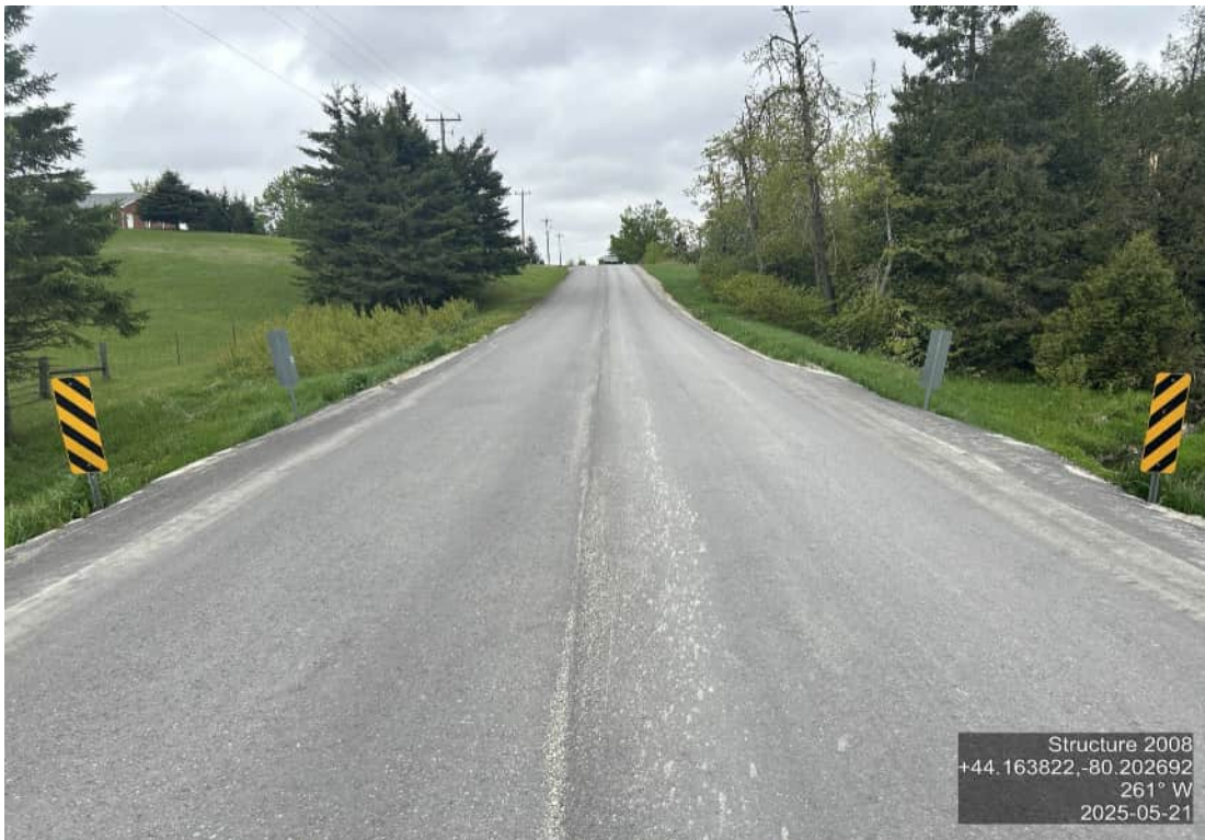
DECK WEARING SURFACE – EAST – LONGITUDINAL CRACKS
