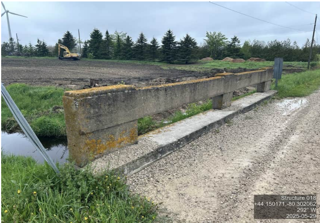
RAILING SYSTEM – SOUTHWEST – LOCALIZED AREAS OF DISINTEGRATION
