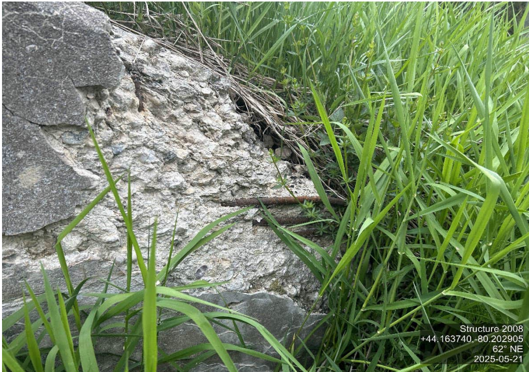
WINGWALL – SOUTHWEST – DISINTEGRATION AND SPALLS WITH EXPOSED CORRODED REBAR
