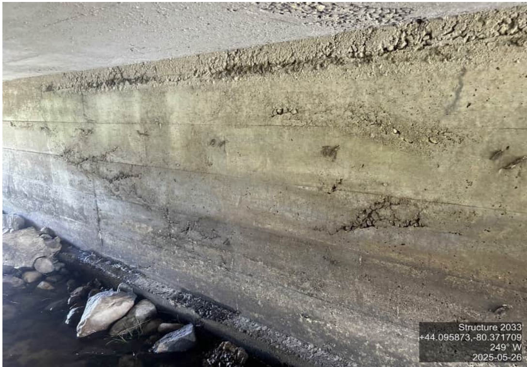
BARREL – INTERIOR – HONEYCOMBING THROUGHOUT AND COLD JOINT PRESENT
