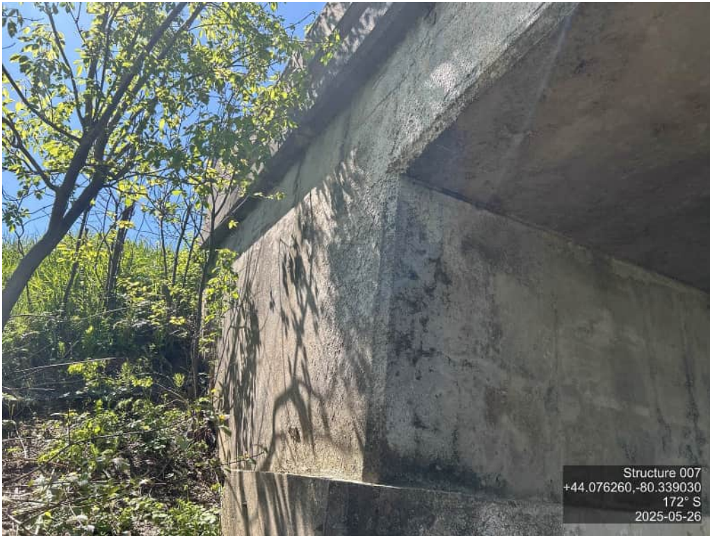
SOFFIT EXTERIOR – EAST – HONEYCOMBING AND EFFLORESCENCE STAINING
