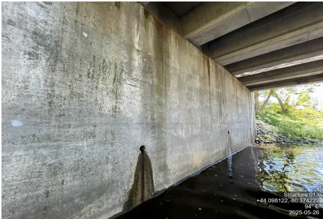
ABUTMENT WALLS – EAST – WIDE VERTICAL CRACK IN CENTER
