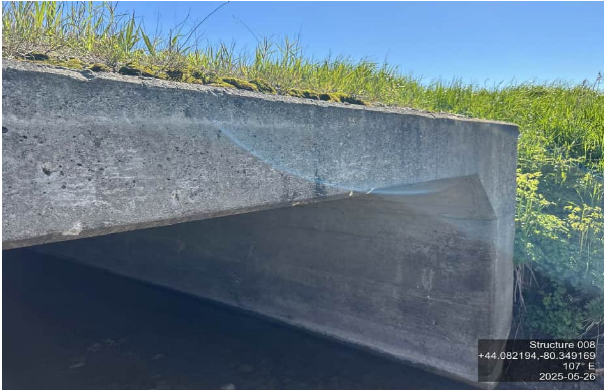
OUTLET – WEST – LIGHT SCALING AND POPOUTS
