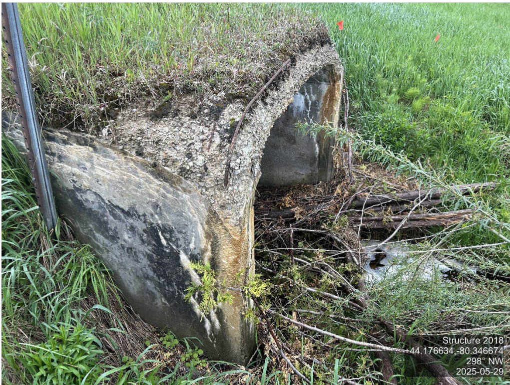
DECK TOP – EAST – SEVERE DISINTEGRATION
