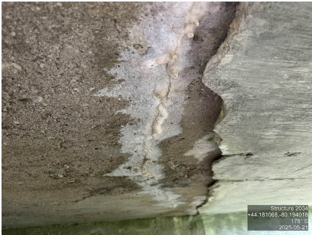
SOFFIT- WEST – EFFLOURESCENCE STAINED CRACKS
