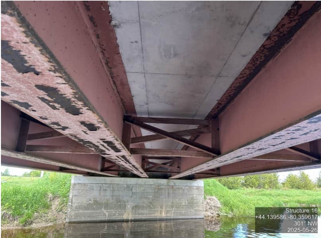
GIRDERS – MIDDLE – MODERATE SURFACE CORROSION
