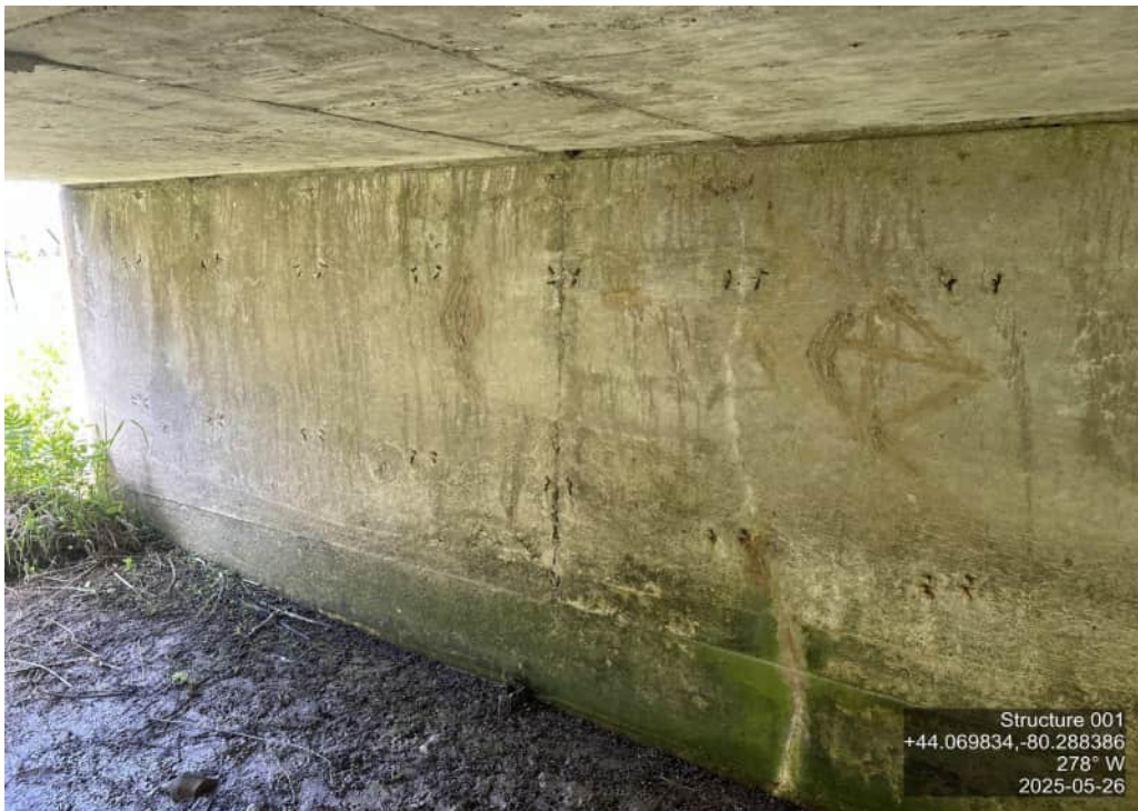
ABUTMENT WALLS – NORTH – FULL HEIGHT CRACK ON EACH WALL
