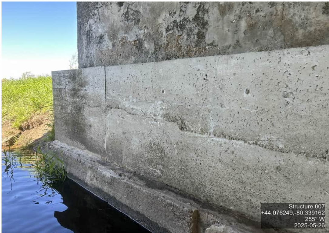
ABUTMENT WALLS – NORTH – COLD JOINTS, HONEYCOMBING AND SEVERAL VERTICAL CRACKS
