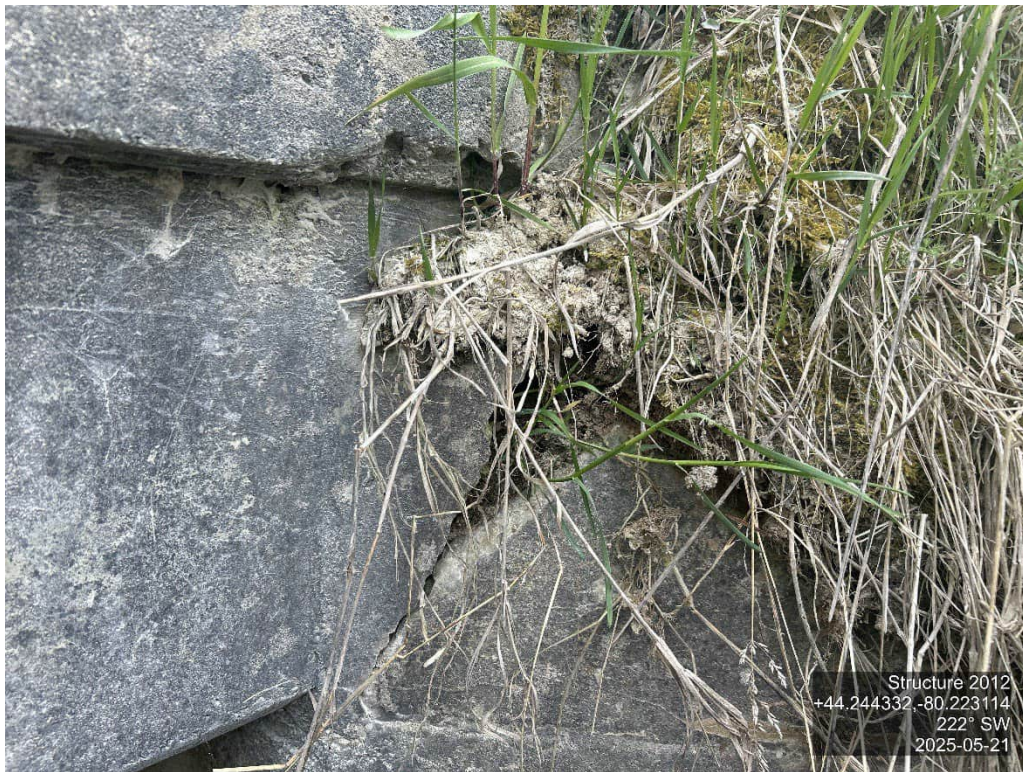
WINGWALL – SOUTHWEST – WIDE CRACK AT CONNECTION
