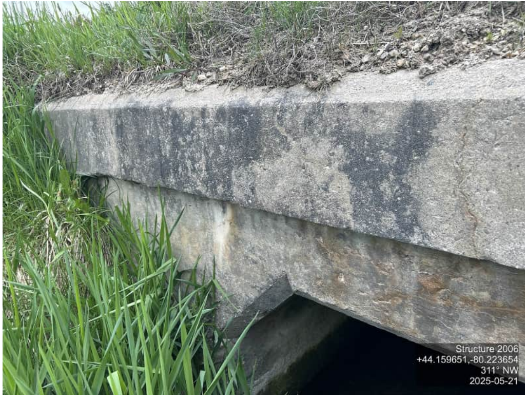
CURB – WEST – IMPACT DAMAGE SPALLS ON ENDS
