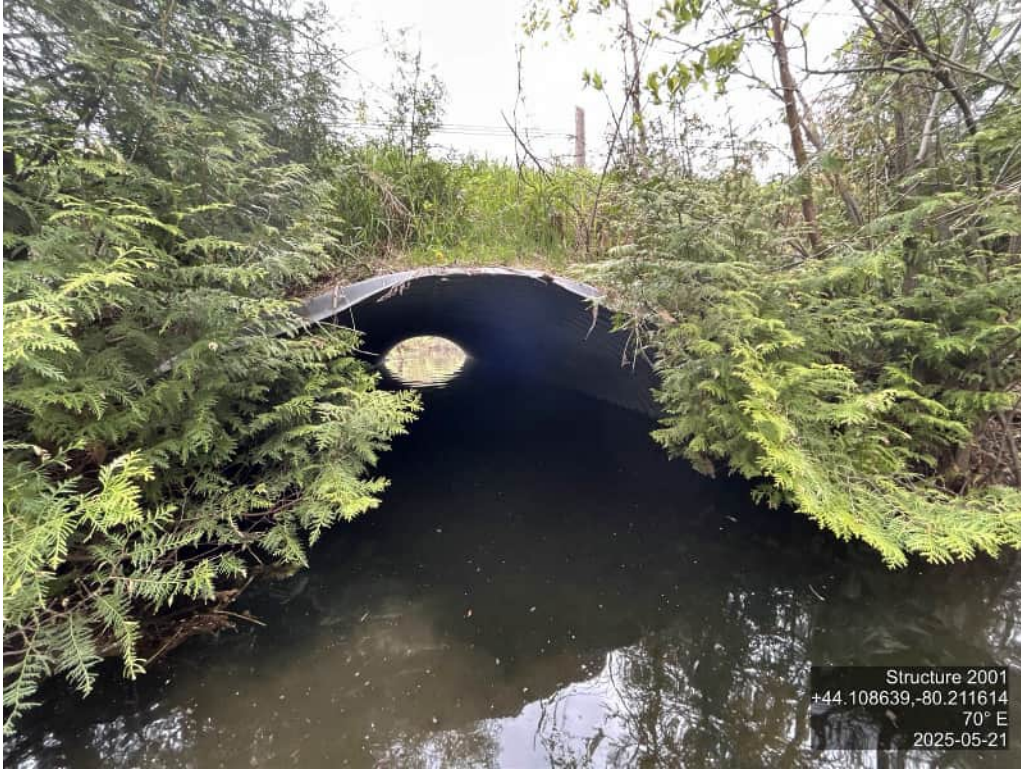
EMBANKMENT – EAST – OVERGROWN VEGETATION
