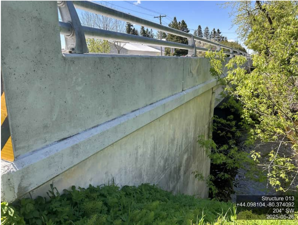
WINGWALL – SOUTHEAST – NARROW CRACKS THROUGHOUT
