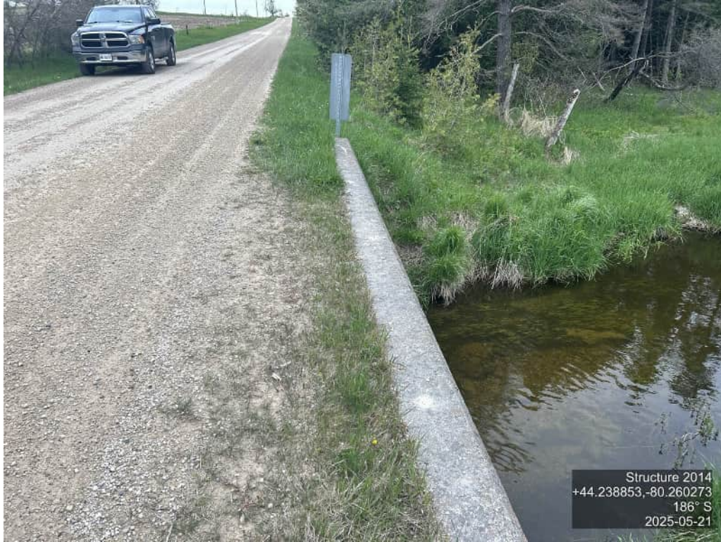
CURB – SOUTHEAST – MEDIUM CRACKS THROUGHOUT
