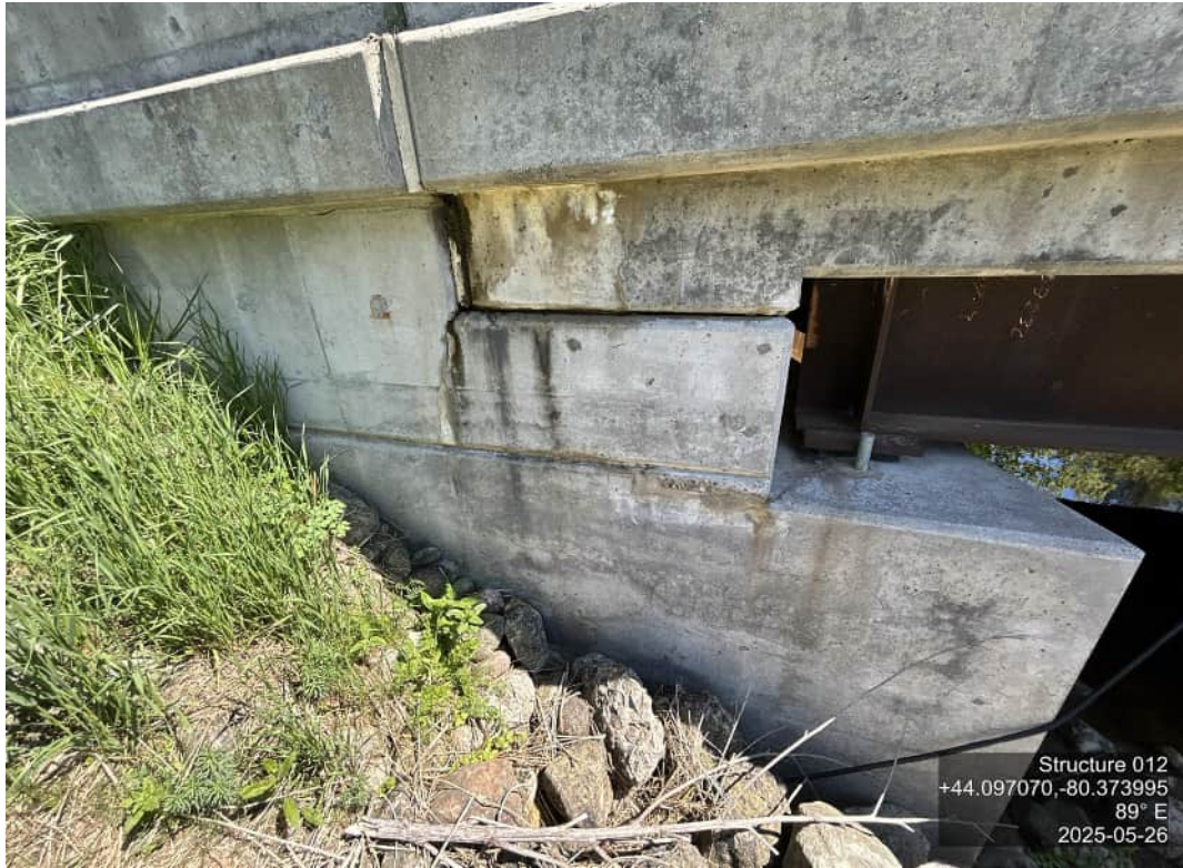
WINGWALLS – WEST – EFFLORESCENCE STAINED CRACK BELOW JOINT
