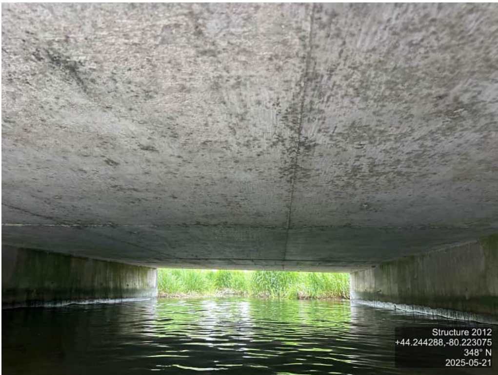
SOFFIT- INTERIOR – LIGHT TO MODERATE HONEYCOMBING
