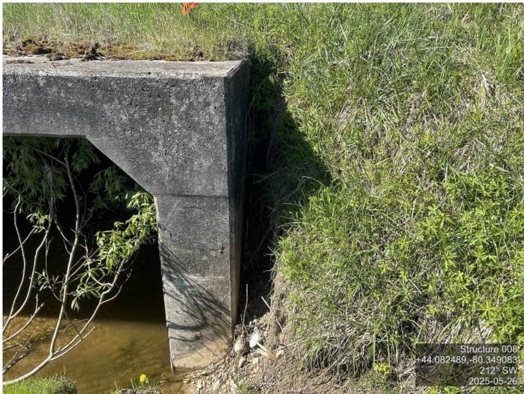
EMBANKMENT – NORTHWEST – LIGHT WASHOUTS ON ALL QUADRANTS
