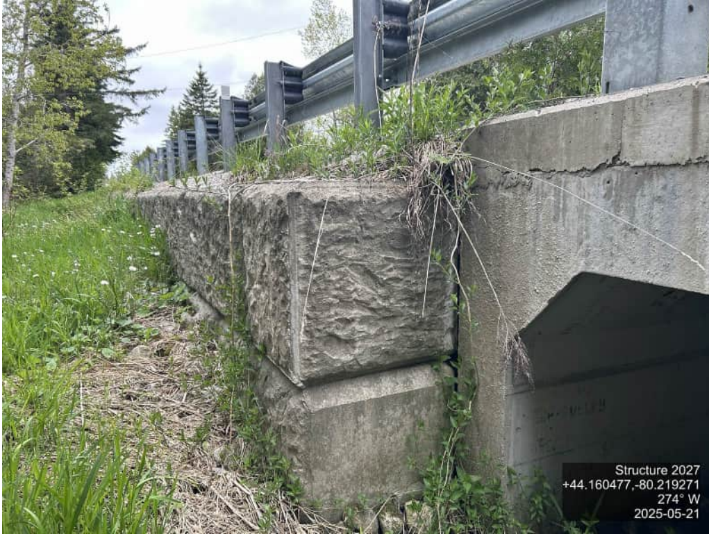
OUTLET – NORTH – HAIRLINE STAINED CRACKS
