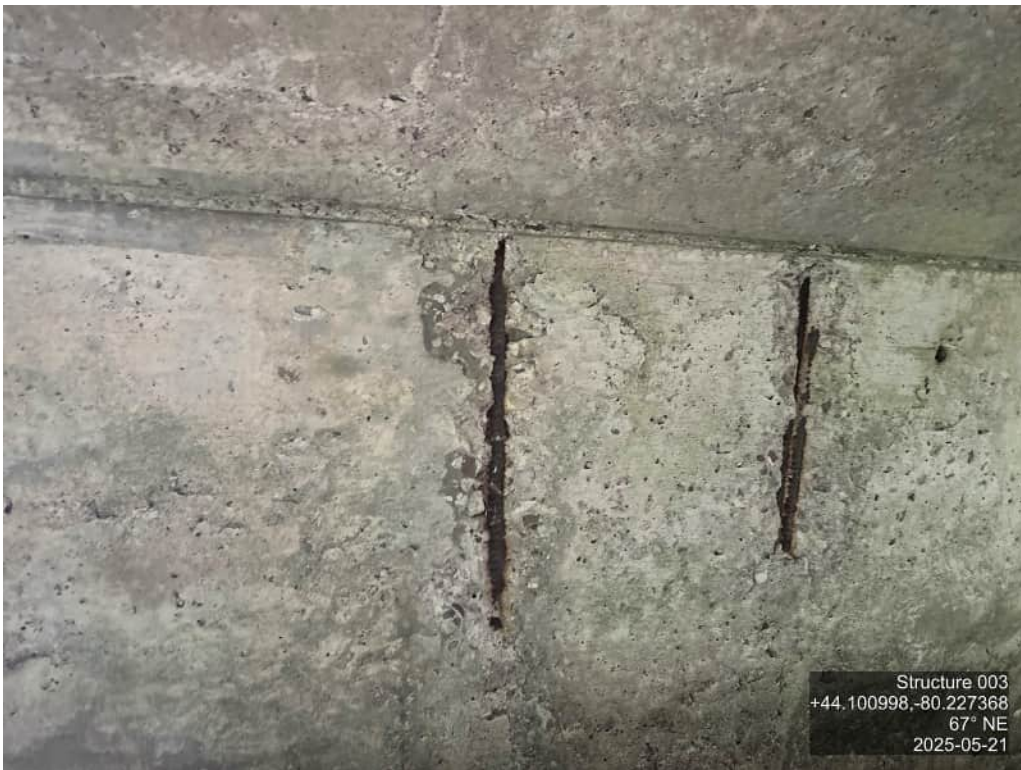
ABUTMENT WALLS –WITH EXPOSED CORRODED REBAR
