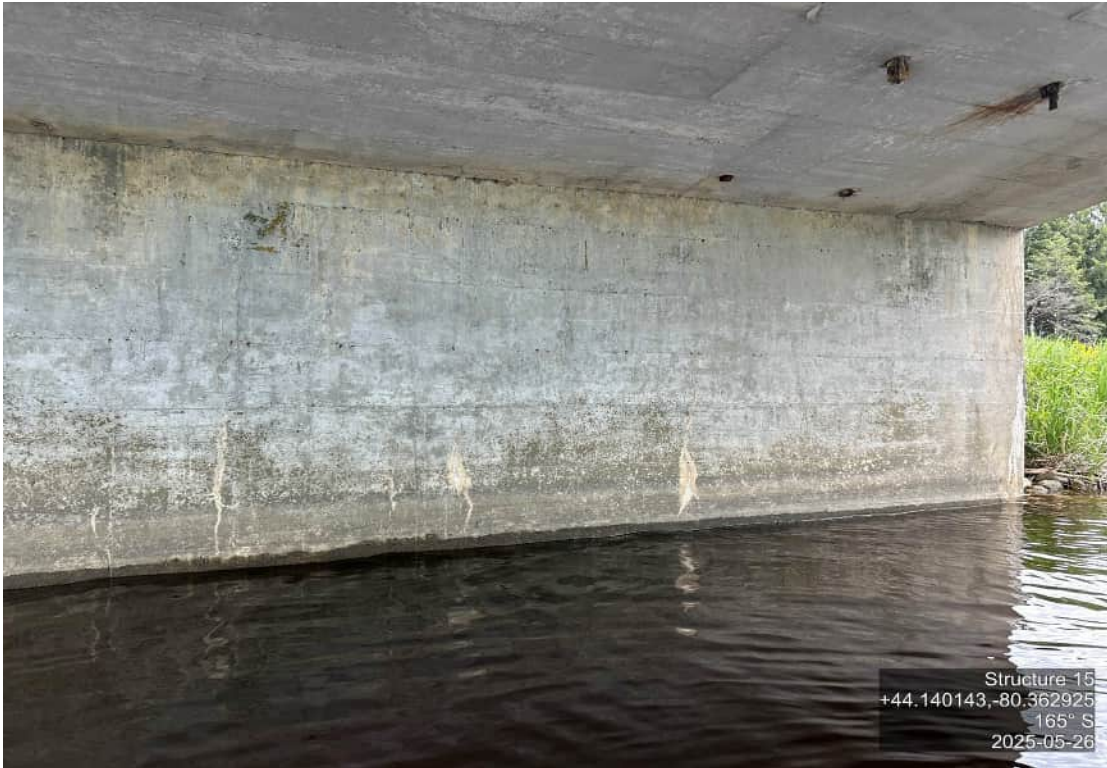
ABUTMENT WALLS – SOUTHWEST – DELAMINATIONS AND STAINED CRACKING
