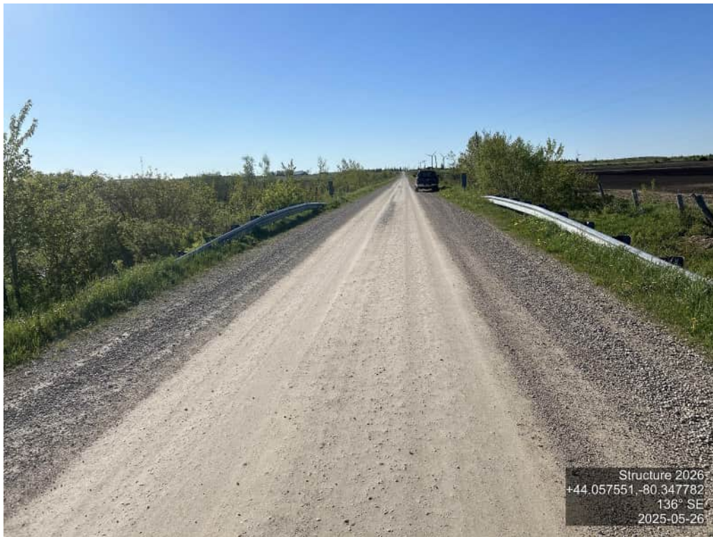
DECK WEARING SURFACE – SOUTHEAST – LOOSE GRAVEL ON SHOULDERS
