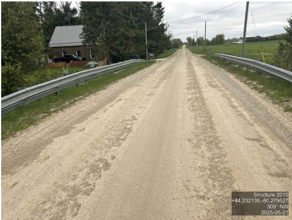
DECK WEARING SURFACE – NORTH – VEGETATION ALONG SHOULDERS
