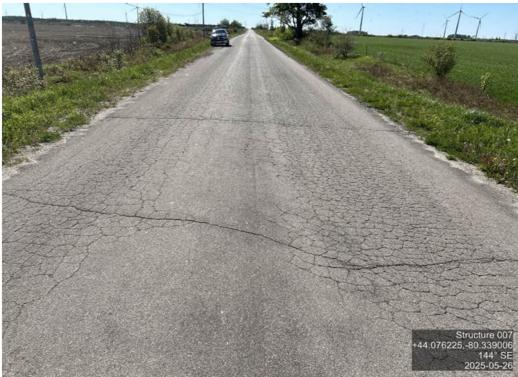
APPROACH WEARING SURFACE – SOUTH – SEVERE ALLIGATOR CRACKING
