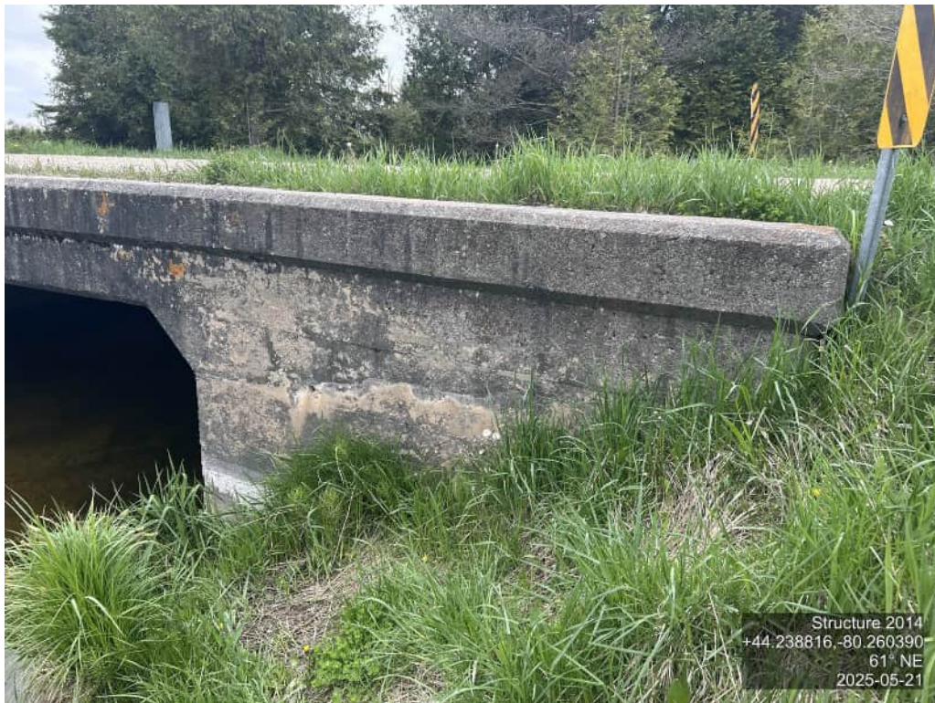
WINGWALL – NORTHWEST – SCALING AND STAINING PRESENT
