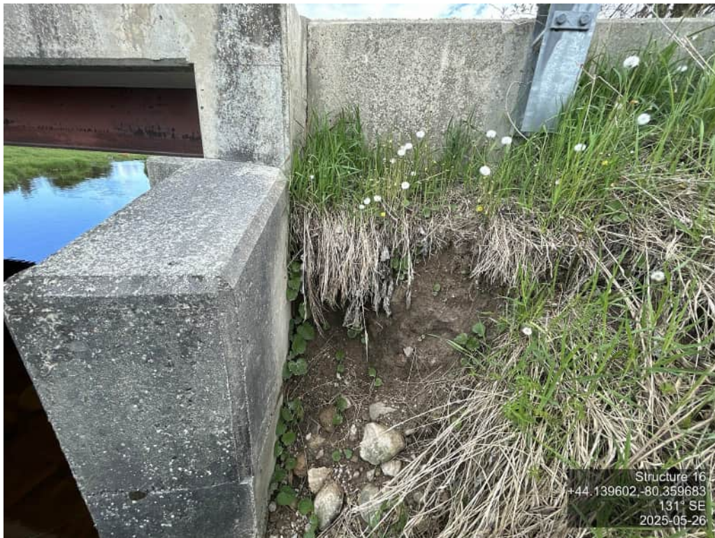
EMBANKMENT – SOUTHWEST – SEVERE ERROSION
