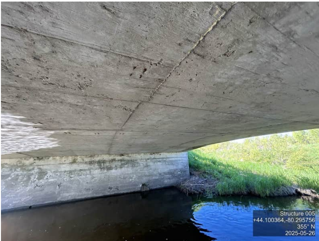
ABUTMENT WALLS – SOUTHEAST – COLD JOINT, DELAMINATIONS AND SEVERE HONEYCOMBING WITH EXPOSED CORRODED REBAR
