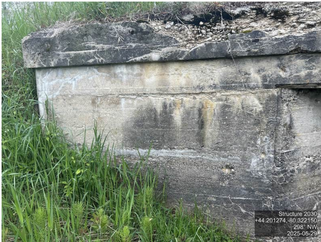
WINGWALL – NORTHWEST – DELAMINATIONS AND COLD JOINTS
