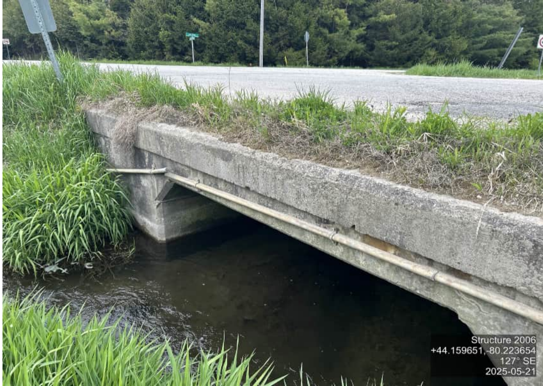
STREAM – SOUTH FOOTING EXPOSED
