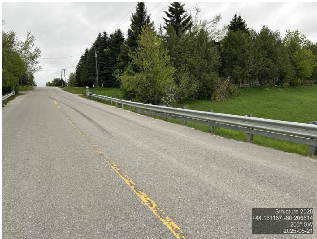
DECK WEARING SURFACE – OVER DECK TOP
