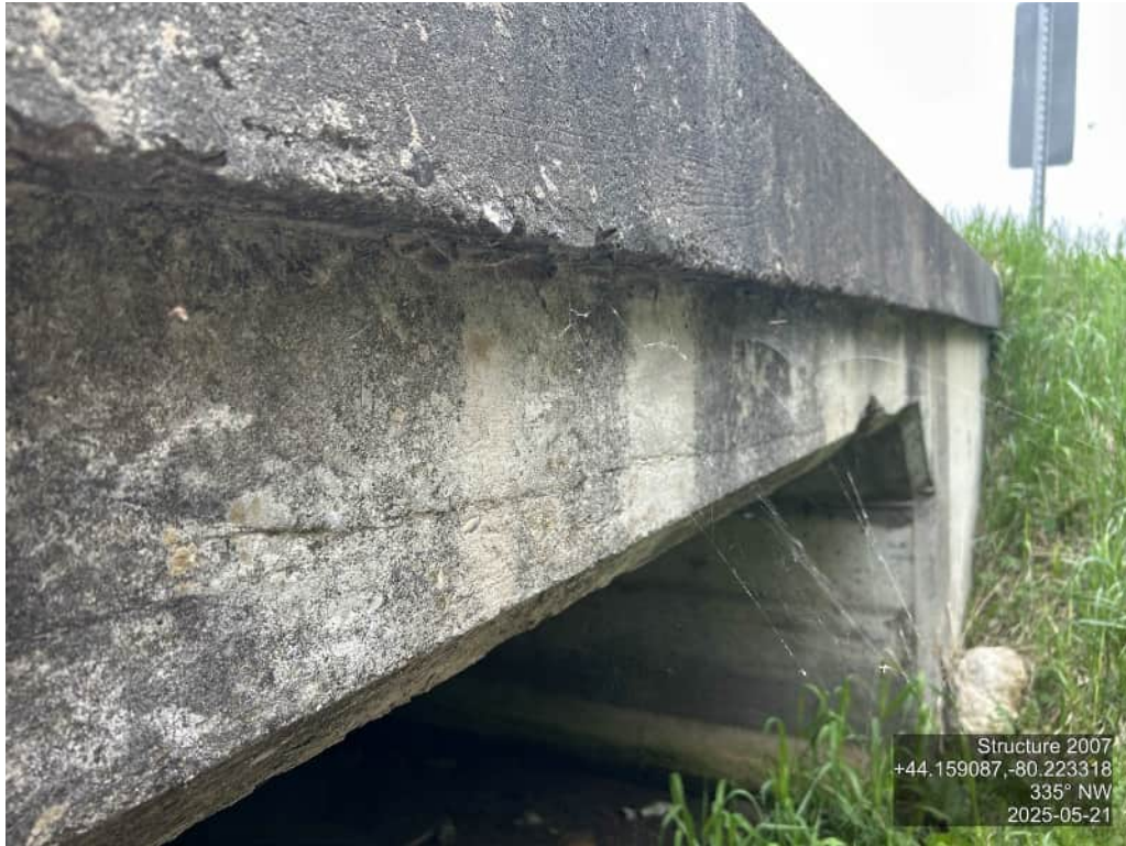
SOFFIT EXTERIOR – SOUTH - DELAMINATIONS
