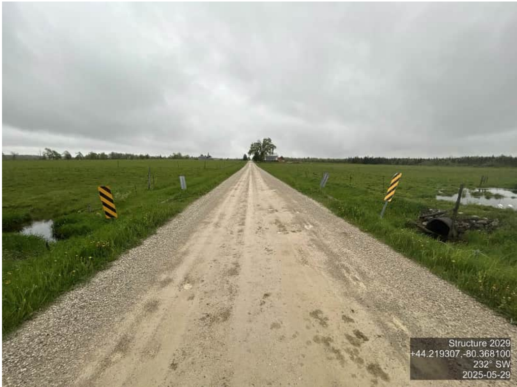
DECK WEARING SURFACE – OVER DECK TOP – SMALL TO MEDIUM POTHOLES
