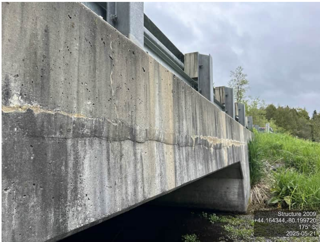
INLET – NORTH – EFFLORESCENCE STAINED CRACKS
