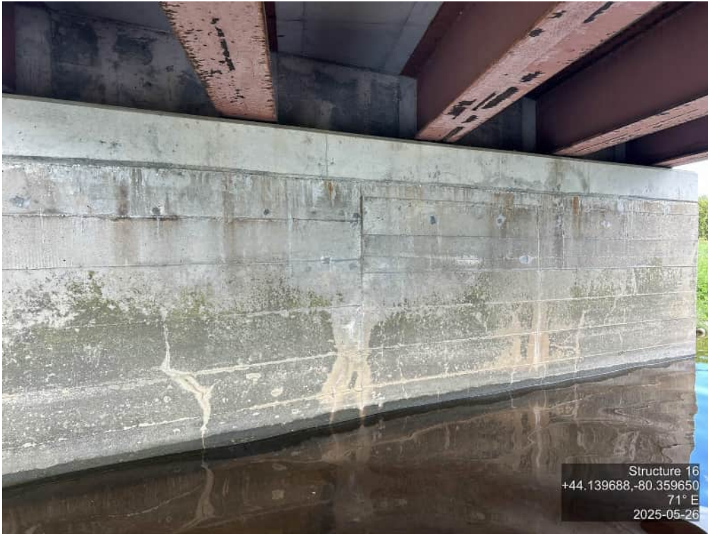
ABUTMENT WALLS – EAST – WIDE VERTICAL CRACKS AND LIGHT HONEYCOMBING
