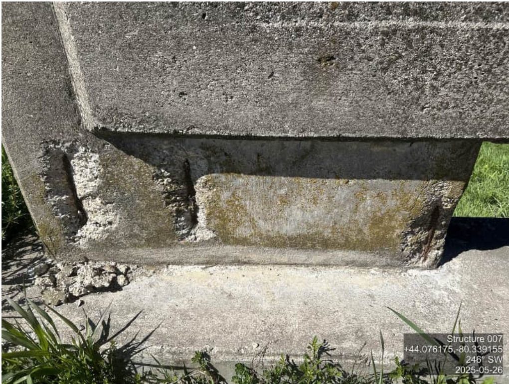
BARRIER POSTS – WEST – SPALLING WITH EXPOSED CORRODED REBAR
