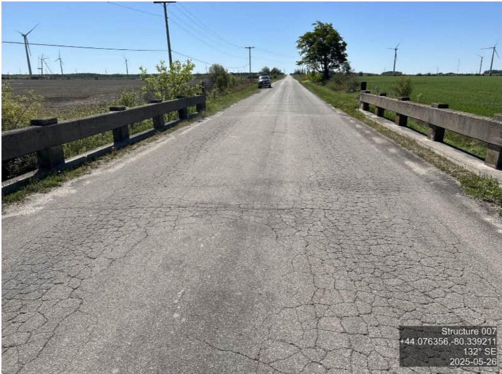
DECK WEARING SURFACE – SOUTH – SEVERE ALLIGATOR CRACKING
