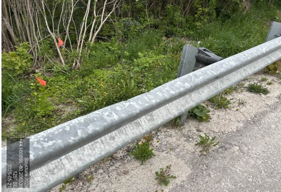
GUIDERAIL – SOUTHEAST – LIGHT IMPACT DAMAGE AND FALLEN POST
