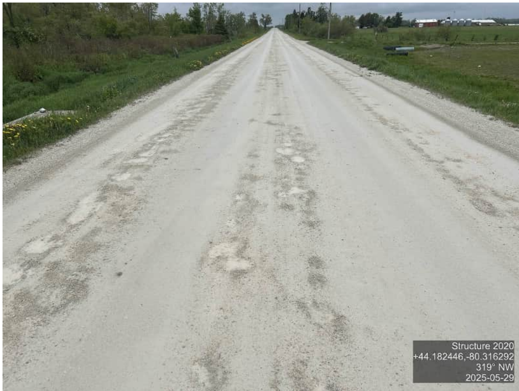
DECK WEARING SURFACE – OVER DECK TOP – SMALL POTHoles
