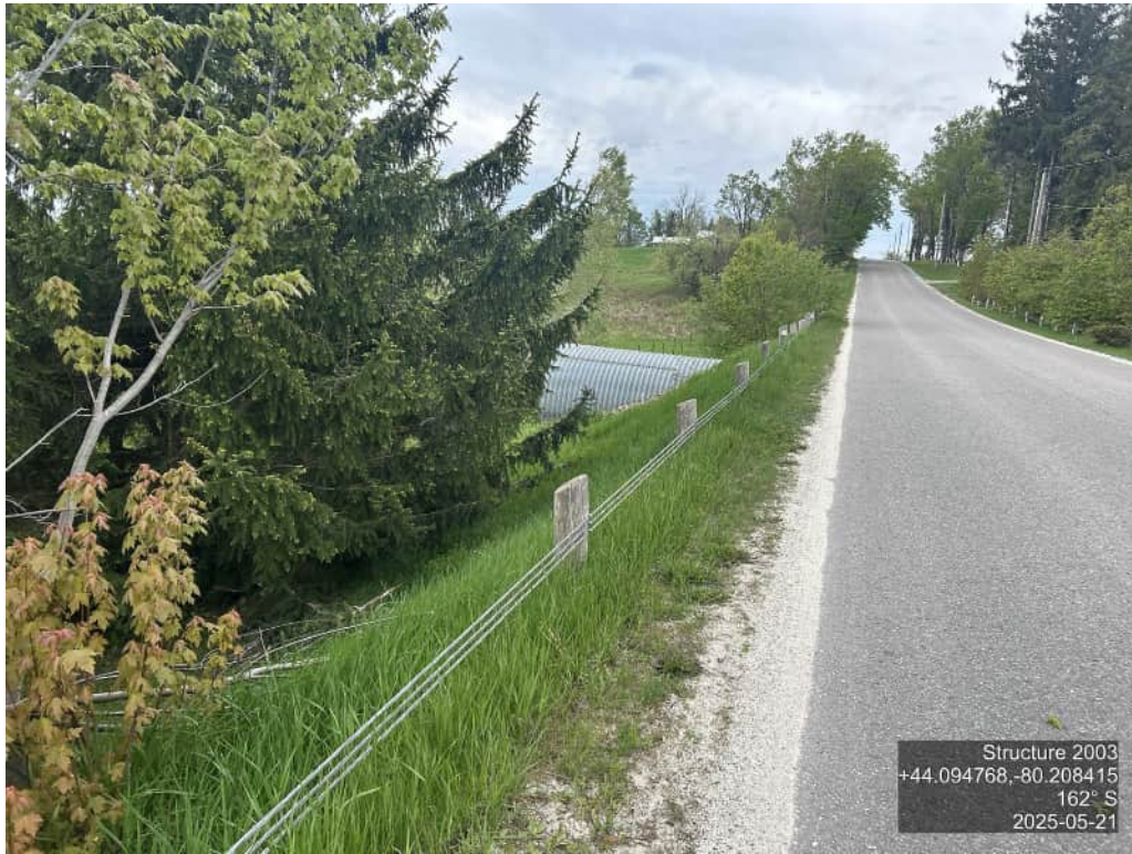
GUIDE RAIL – WEST – ROTTED POSTS
