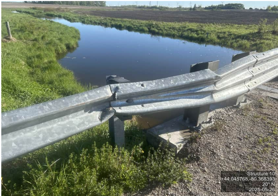
APPROACH GUIDERAIL – NORTH – IMPACT DAMAGE THROUGHOUT
