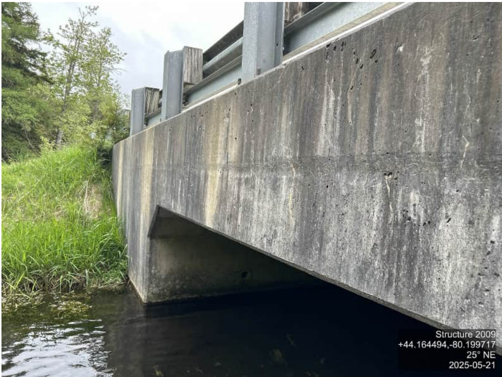
OUTLET – SOUTH – EFFLORESCENCE STAINED CRACKS THROUGHOUT
