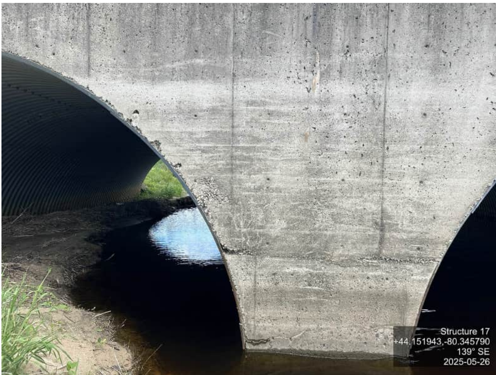
INLET – WEST – HONEYCOMBING AND POPOUTS
