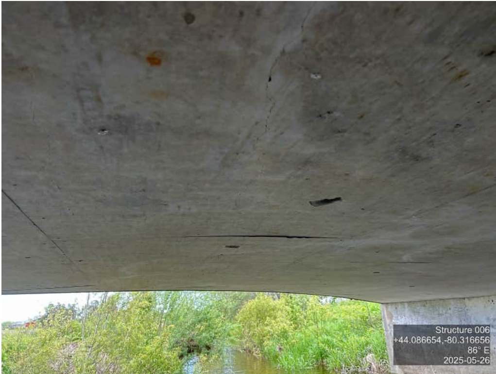
SOFFIT INTERIOR – MIDSPAN – TRANSVERSE CRACK FULL WIDTH
