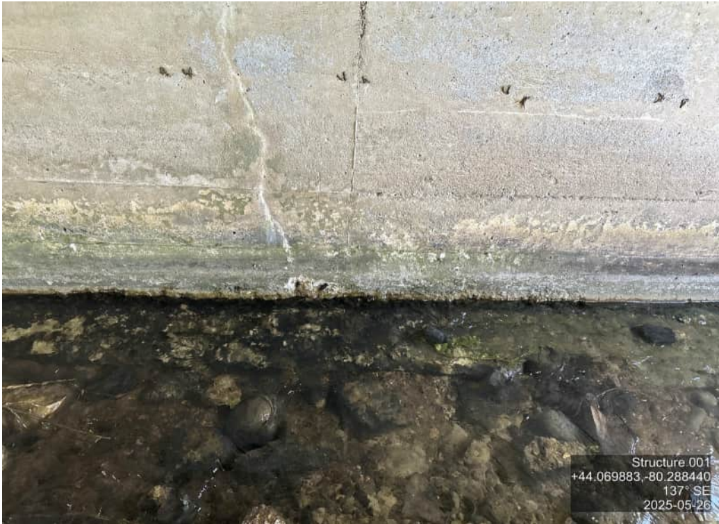
FOUNDATION – SOUTH – TOP OF FOOTING EXPOSED AND SEVERELY ERODED
