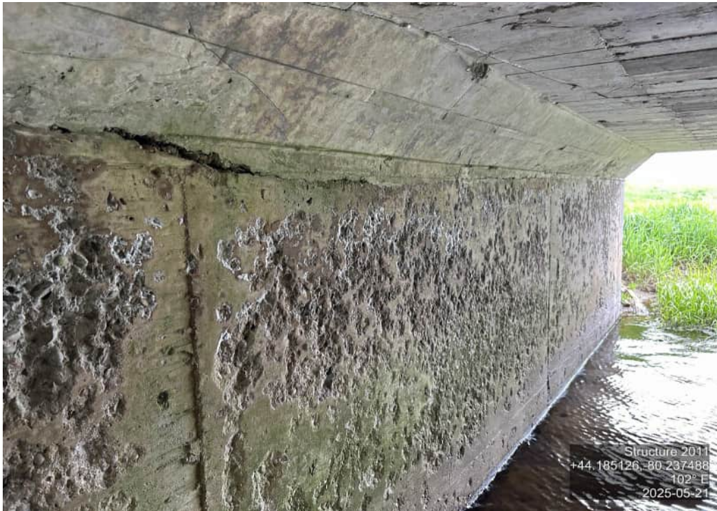
ABUTMENT WALLS – EAST – SEVERE SCALING WITH HONEYCOMBING AND DELAMINATIONS
