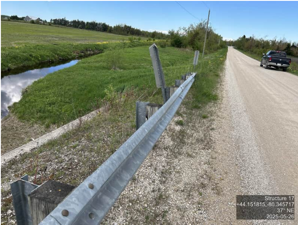
GUIDE RAIL – WEST – ROTTING OFFSET BLOCKS
