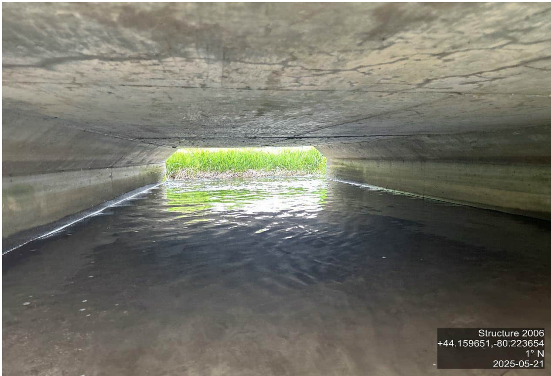
SOFFIT – INTERIOR – SPALLS WITH EXPOSED CORRODED REBAR
