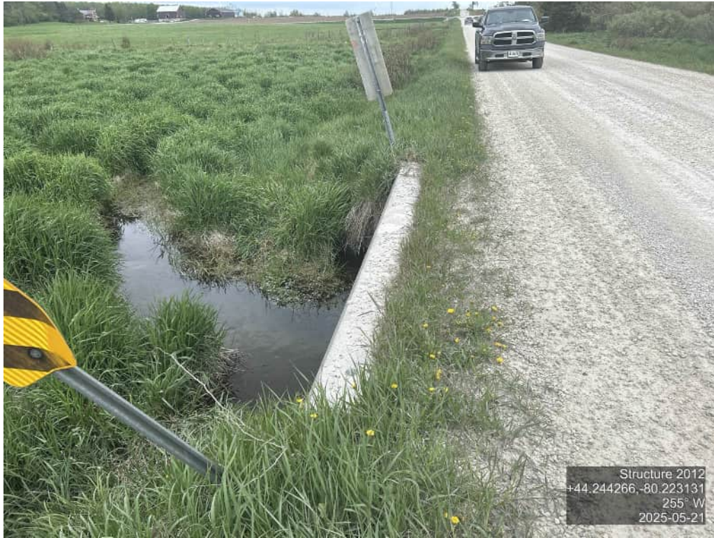
CURB – SOUTH – IMPACT DAMAGE ON SW SIDE
