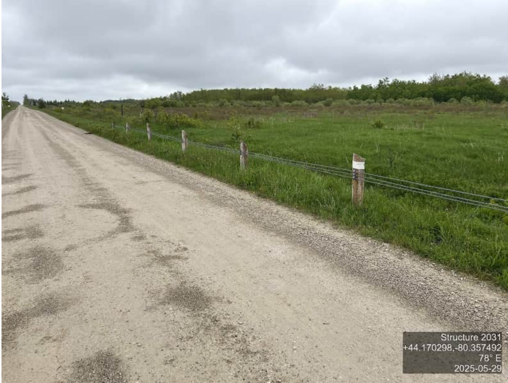
GUIDERAIL – SOUTH – FEW ROTTEN POSTS AND CABLE IS LOOSE
