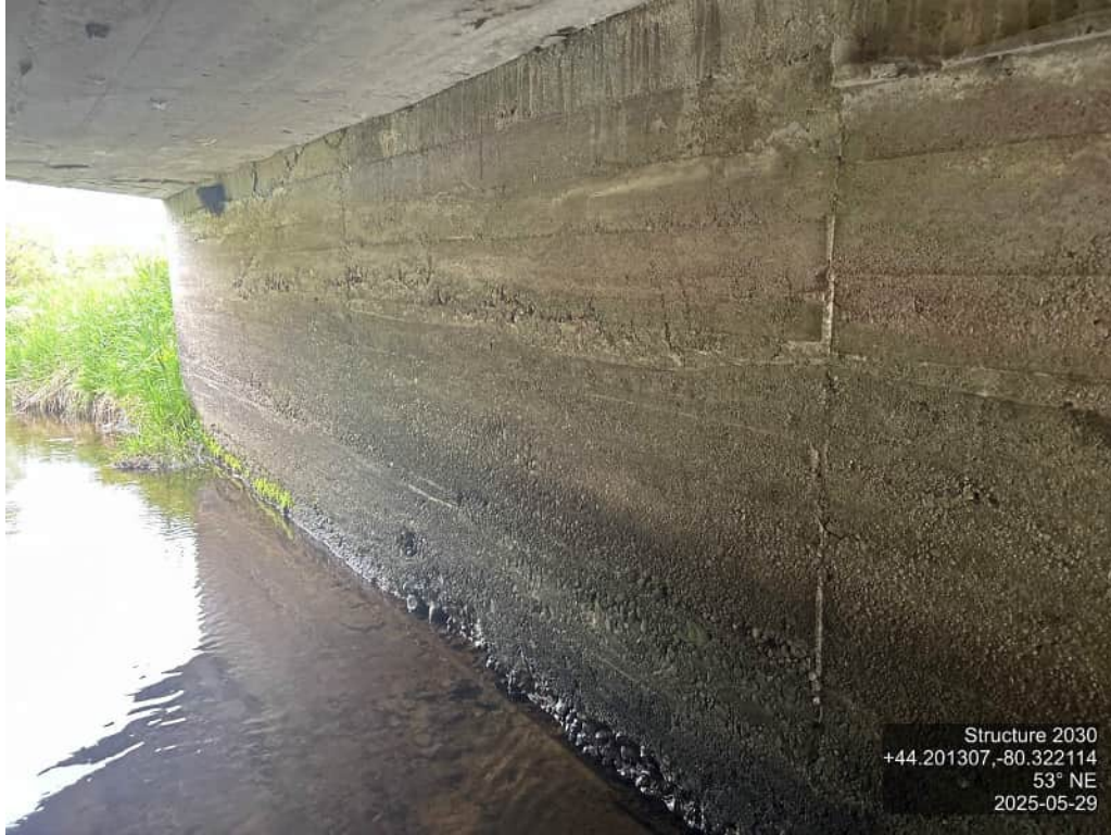
ABUTMENT WALL – EAST – EROSION AND SCOUR ON BOTH WALLS
