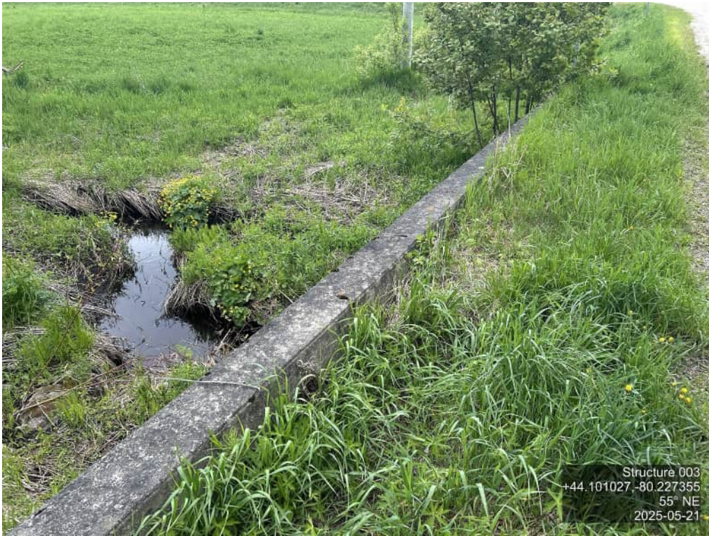
CURB – NORTH – SPALLS WITH EXPOSED CORRODED REBAR
