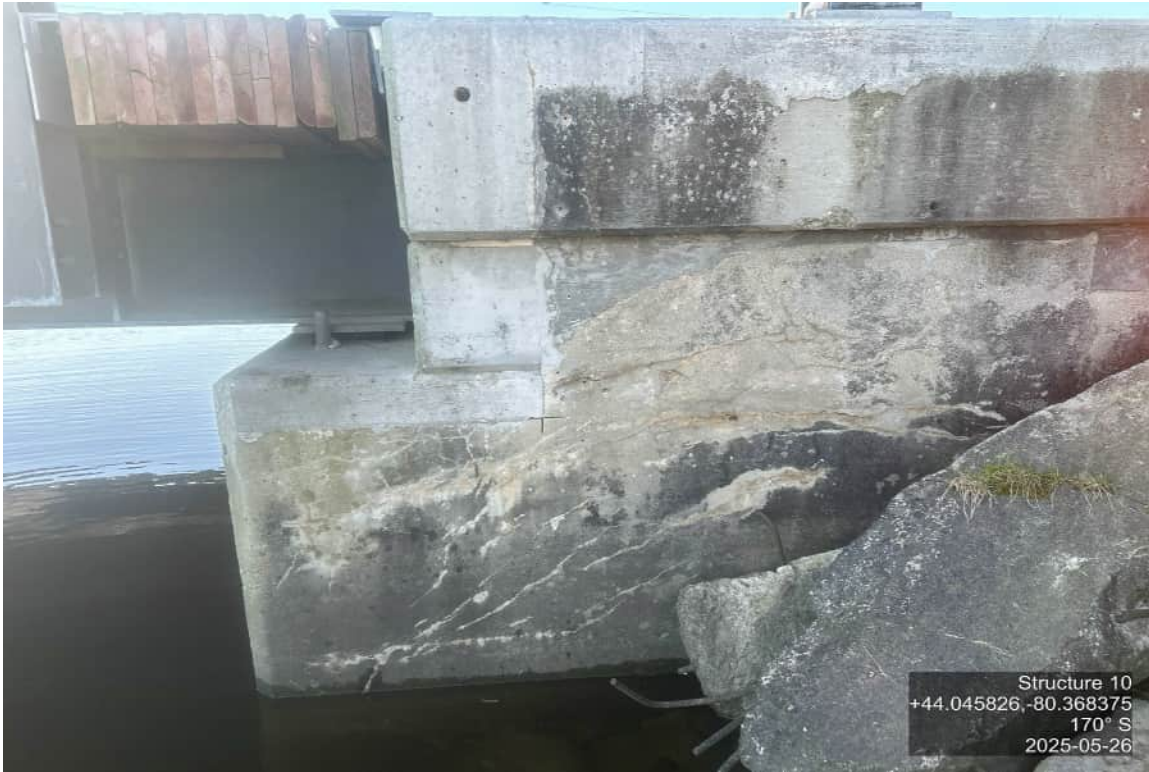
EMBANKMENTS – NORTHWEST – OLD CONCRETE ON EMBANKMENT
