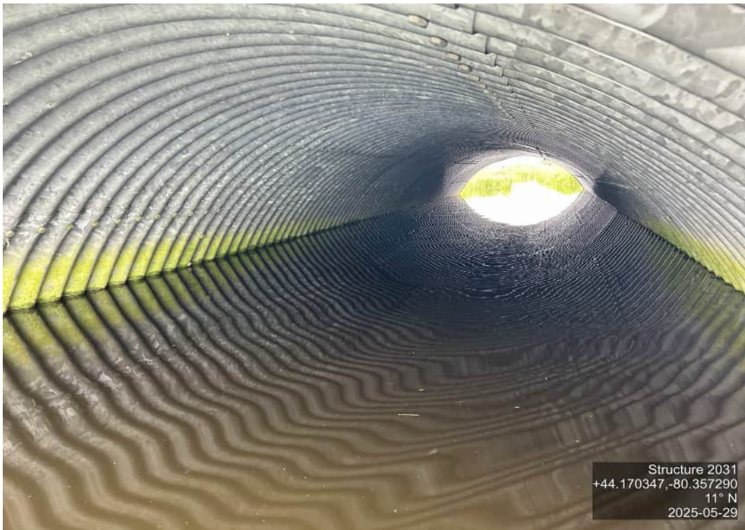
BARREL – NORTH – DEFORMATION IN MIDDLE AND MISSING BOLTS
