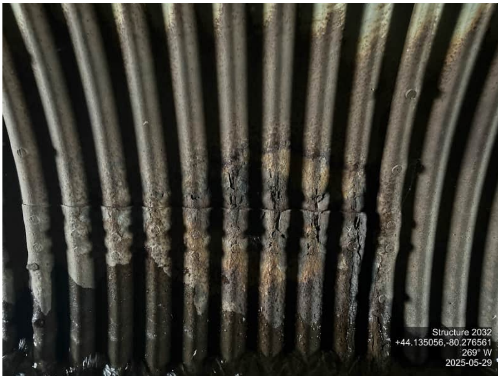
BARREL – SOUTH – MODERATE SURFACE CORROSION, FLAKING AND SECTION LOSS
