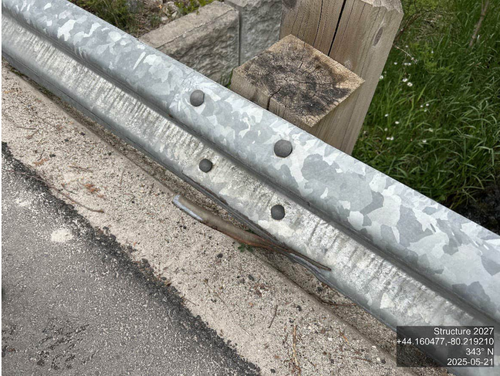
GUIDERAIL – NORTH – LIGHT IMPACT DAMAGE
