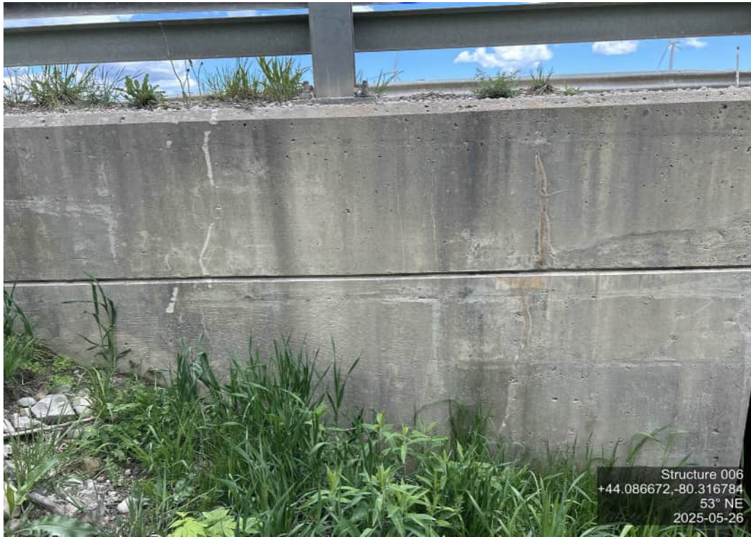
WINGWALL – SOUTHEAST – NARROW STAINED CRACKS
