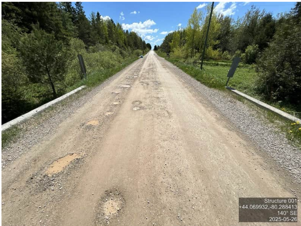
APPROACH WEARING SURFACE – SOUTHEAST – MEDIUM SIZED POTHOLE
