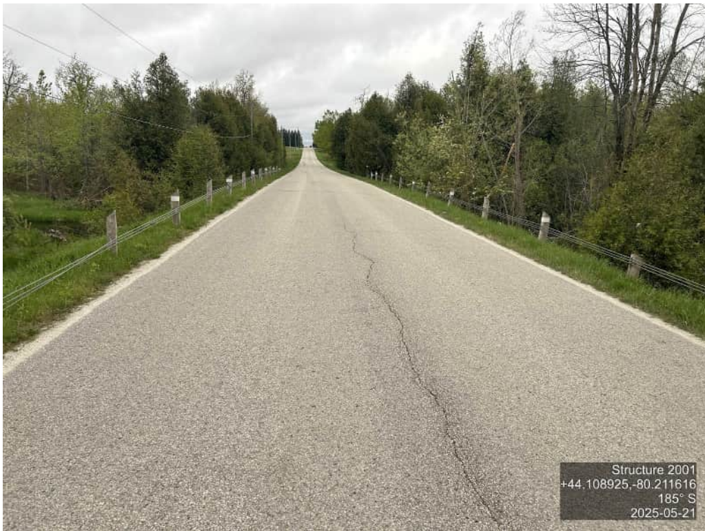
DECK WEARING SURFACE – SOUTH – WIDE TRANSVERSE CRACKS
