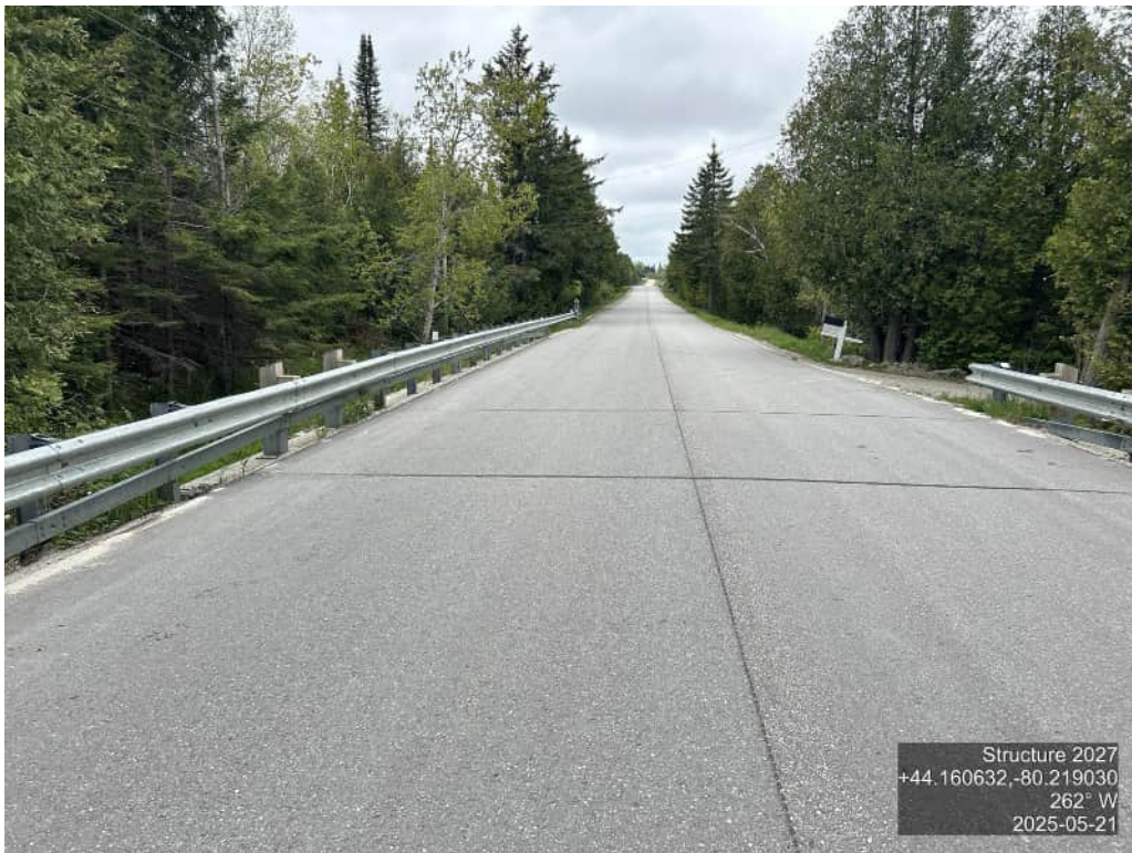
WEARING SURFACE – WEST – LIGHT EDGE CRACKING
