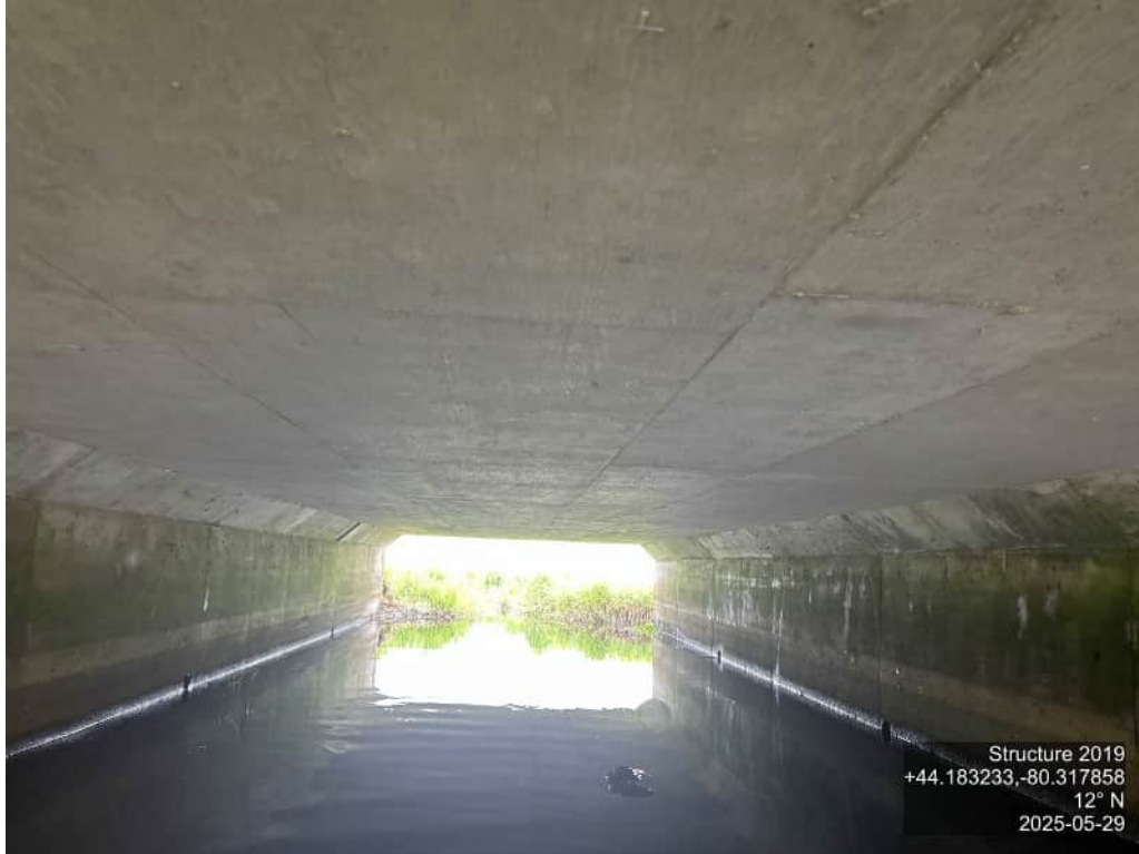
STREAM – NORTH – VEGETATION PARTIALLY OBSTRUCTING WATECOURSE
