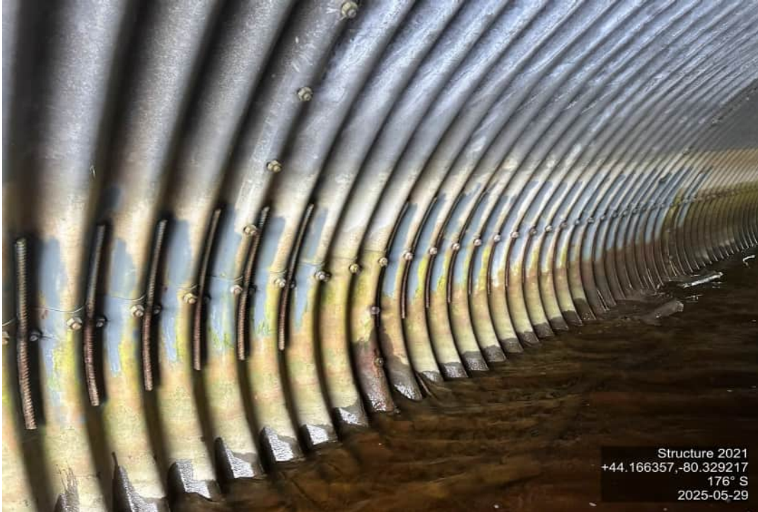
BARREL – SOUTH – FLAKING AND PERFORATIONS UP TO SPRING LINE
