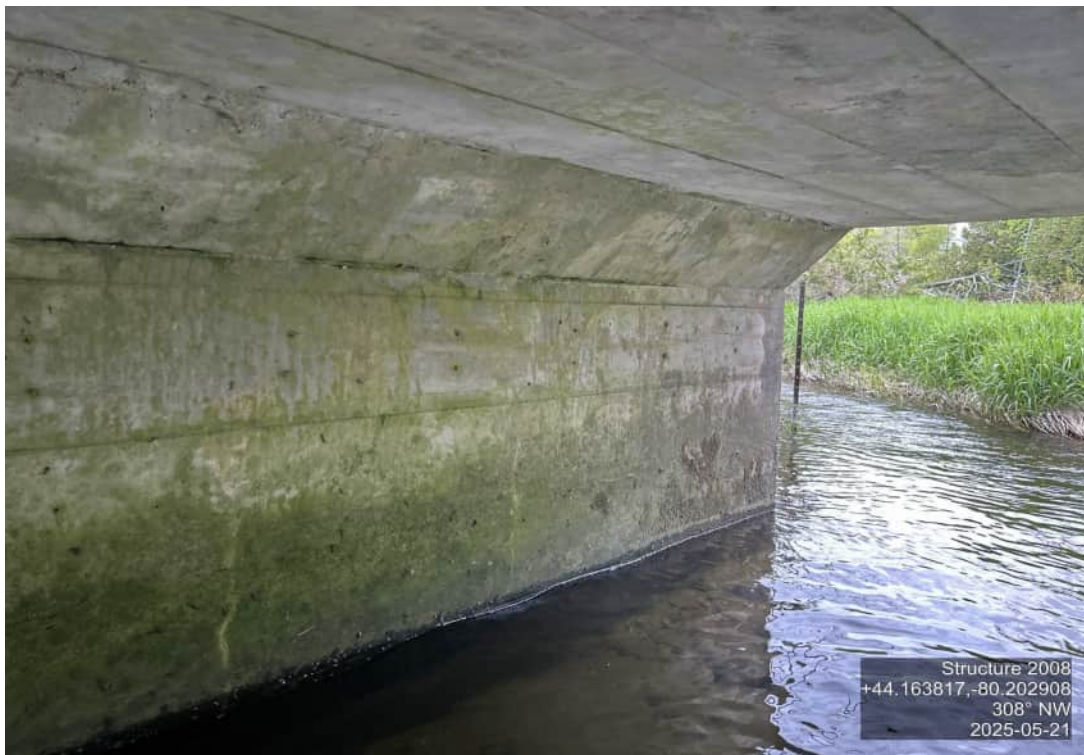
ABUTMENT WALLS – NORTHWEST – VERTICAL CRACKS
