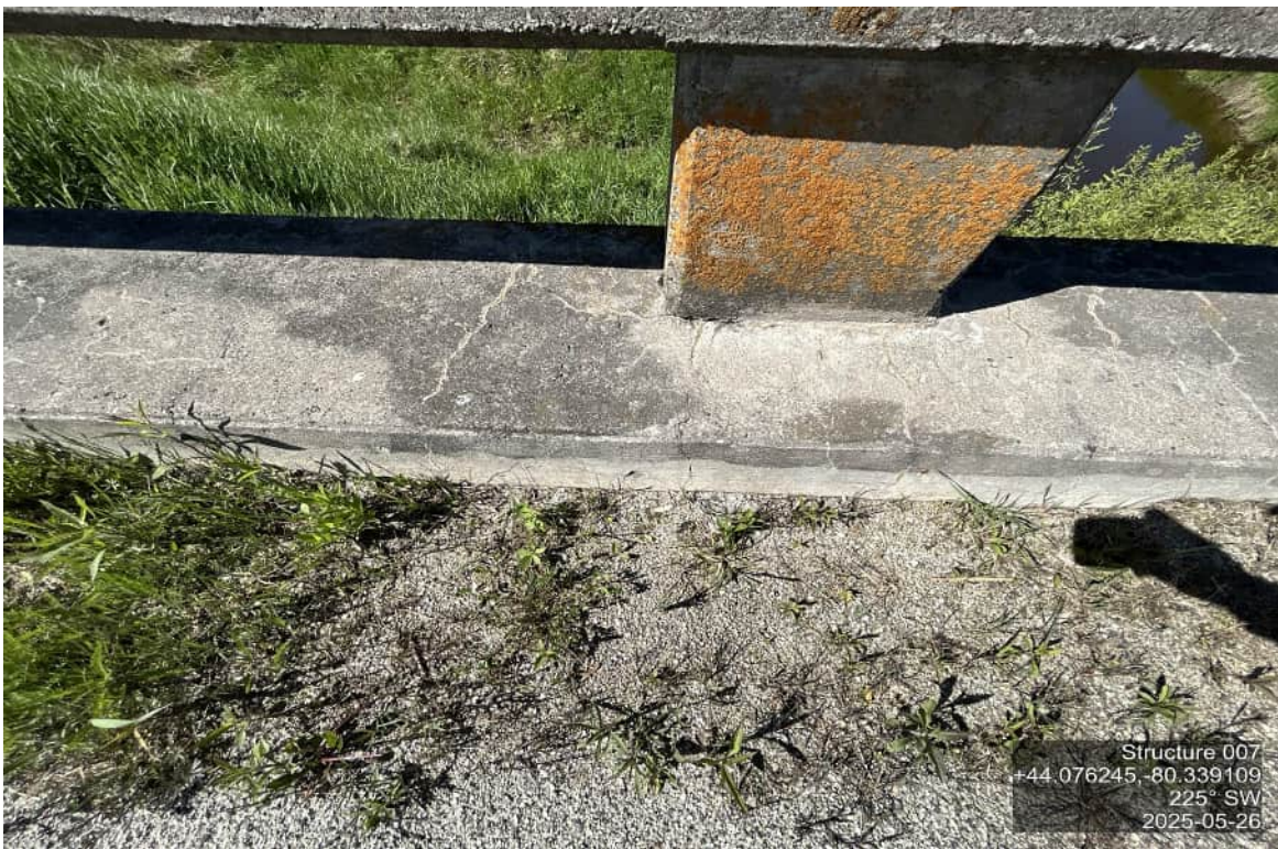
CURB– WEST - NARROW STAINED CRACKS, DELAMINATIONS AND ABRASIONS
