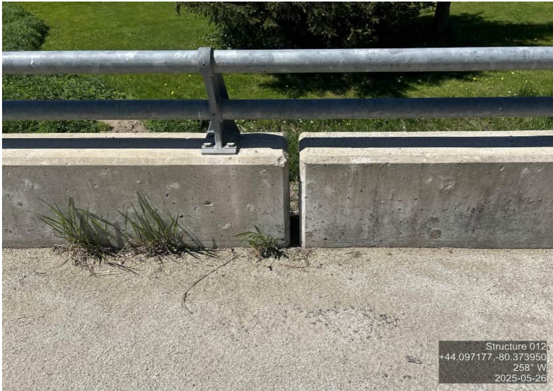
BARRIER WALLS INTERIOR – NORTH – MISSING JOINT SEAL
