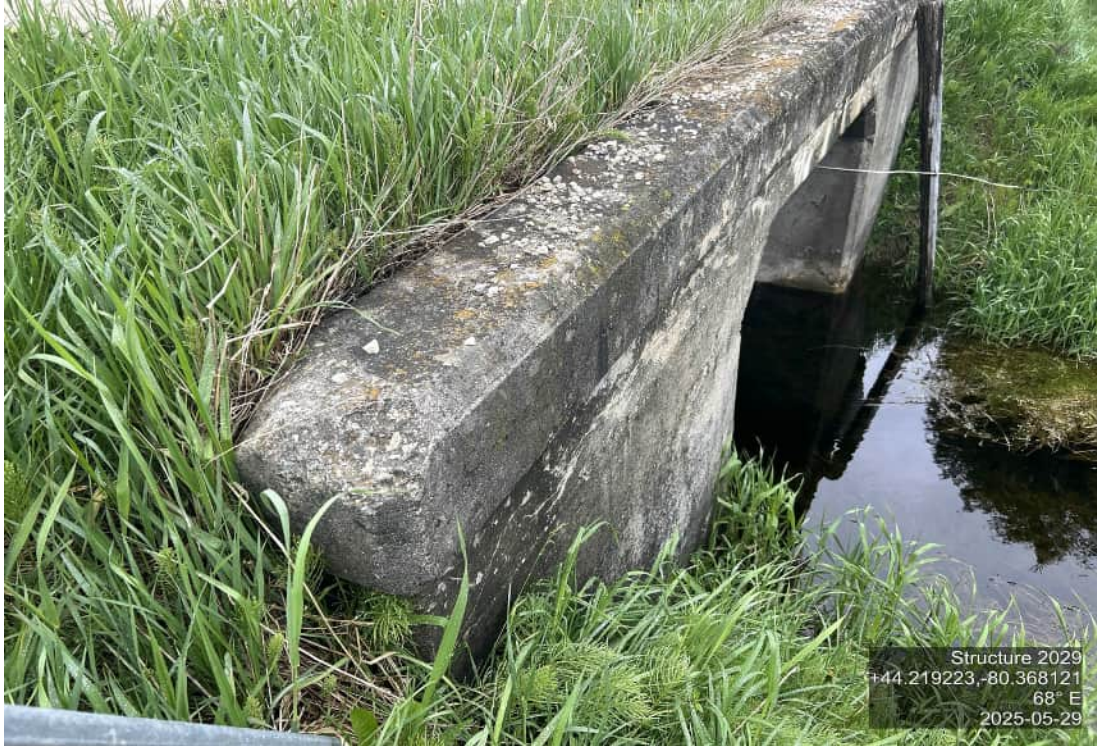
CURB – SOUTH – IMPACT DAMAGE ON CORNERS AND WIDE CRACK AT CENTERLINE
