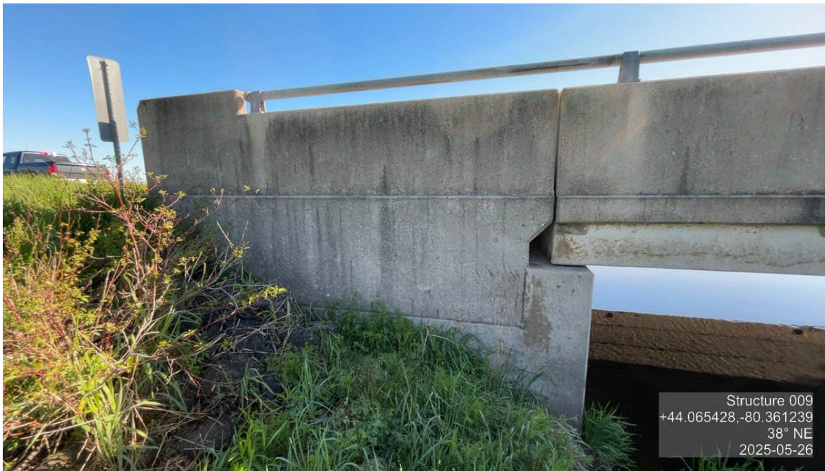
WINGWALL – NORTHEAST – NARROW STAINED CRACKS
