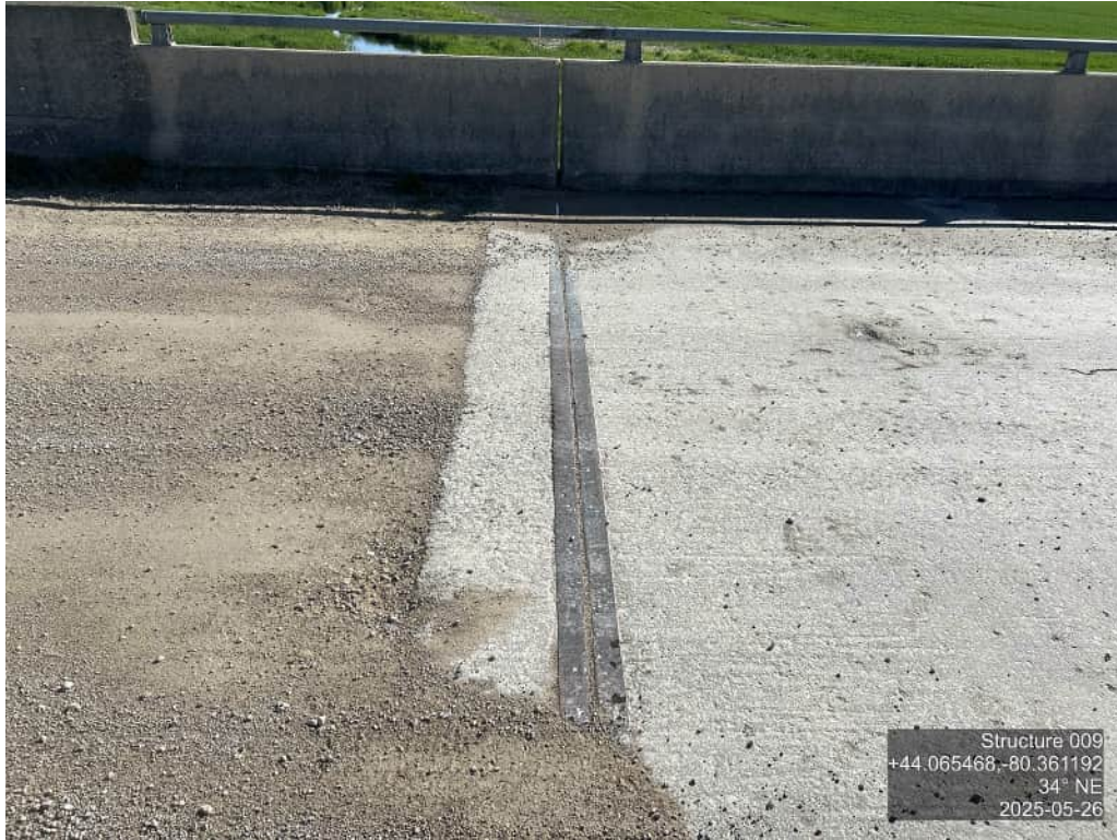
ARMOURING – NORTH – APPEARS TO BE SEIZED
