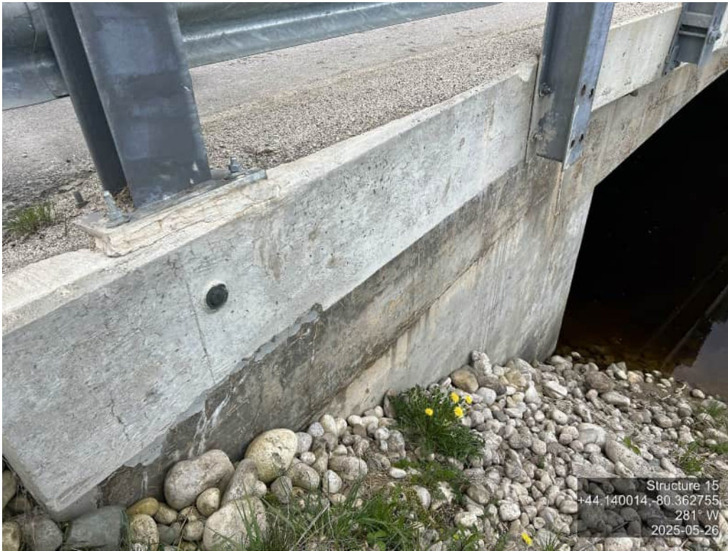
CURB – NORTHEAST – LIGHT SCALING
