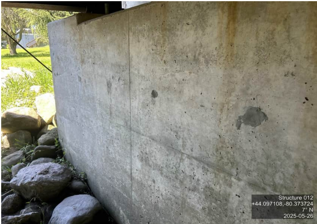
ABUTMENT WALLS – LOCATION – MEDIUM VERTICAL CRACK ON EACH WALL
