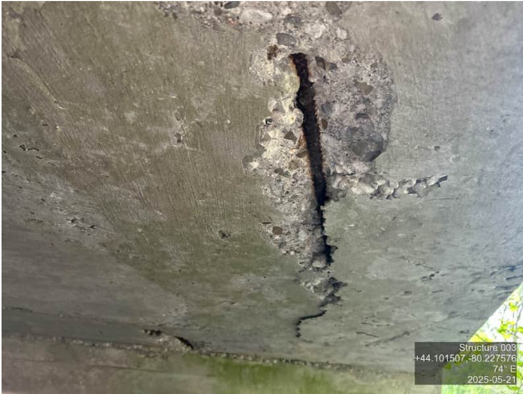
SOFFIT INTERIOR – UNDERSIDE – SPALLS WITH EXPOSED CORRODED REBAR
