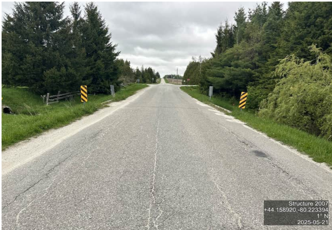
DECK WEARING SURFACE – NORTH – SEVERE ALLIGATOR CRACKING
