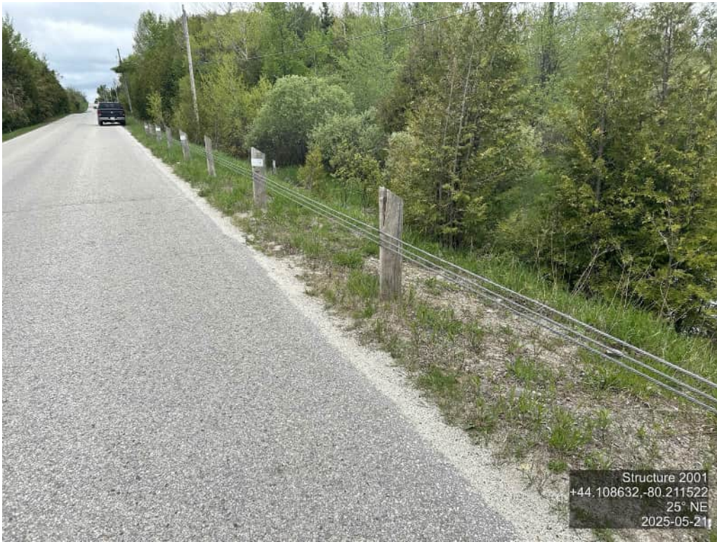
GUIDE RAIL – WEST – ROTTED POSTS AND LOW CABLES
