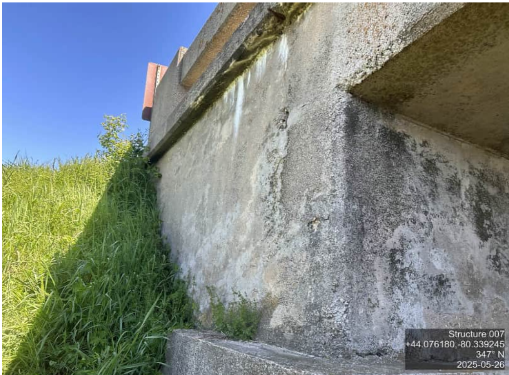
WINGWALLS – NORTHWEST – LIGHT HONEYCOMBING, DISSINTEGRATION AND EFFLORESCENCE STAINING
