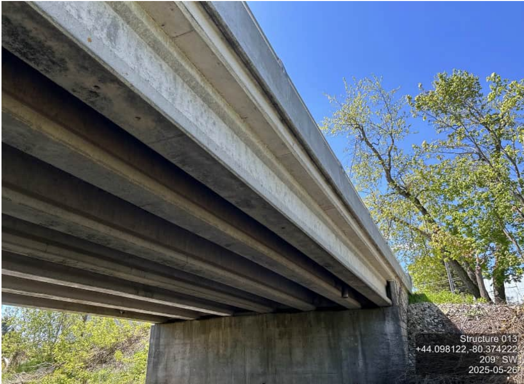
GIRDERS – MIDDLE – NARROW CRACKS THROUGHOUT
