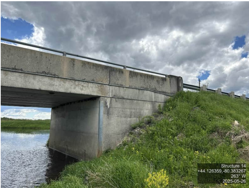
WINGWALL – EAST – NARROW STAINED CRACKS
