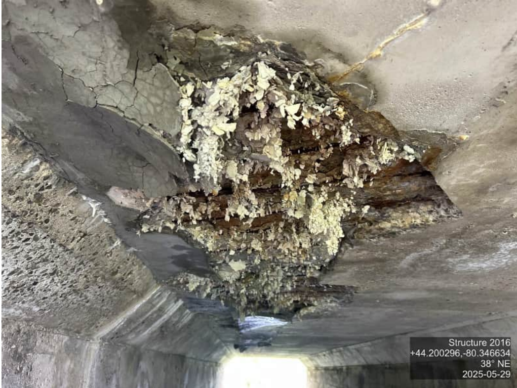
SOFFIT – INTERIOR – SEVERE SPALLING AND DELAMINATIONS THROUGHOUT
