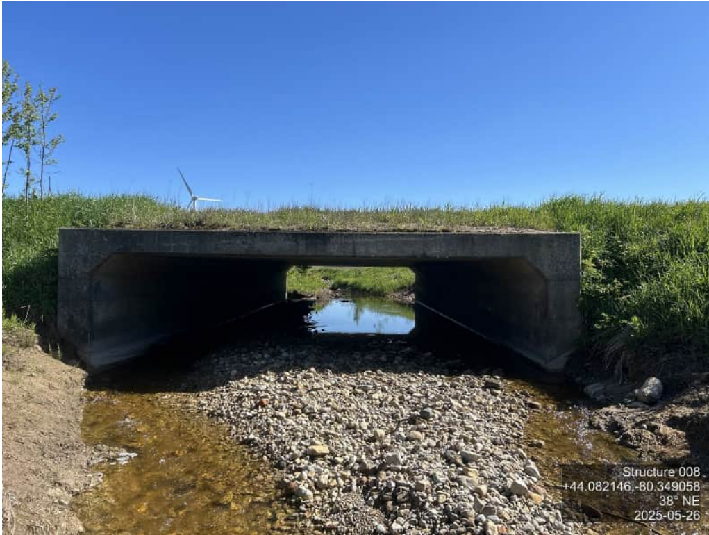
STREAM – FLOWS EAST TO WEST – HEAVY AGGRADATION AT INLET AND OUTLET
