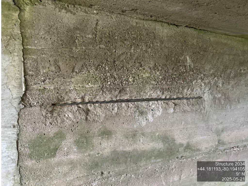
ABUTMENT – NORTH – SPALL WITH EXPOSED REBAR
