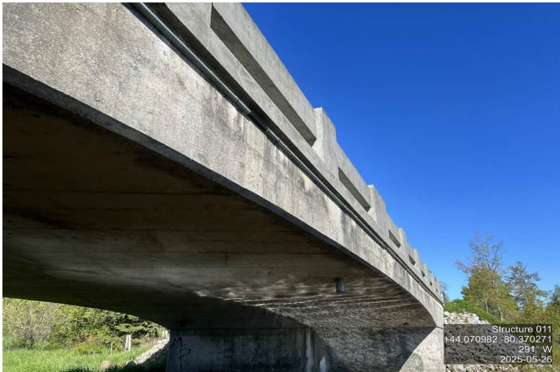
SOFFIT EXTERIOR – WEST – DAMPNESS NOTED
