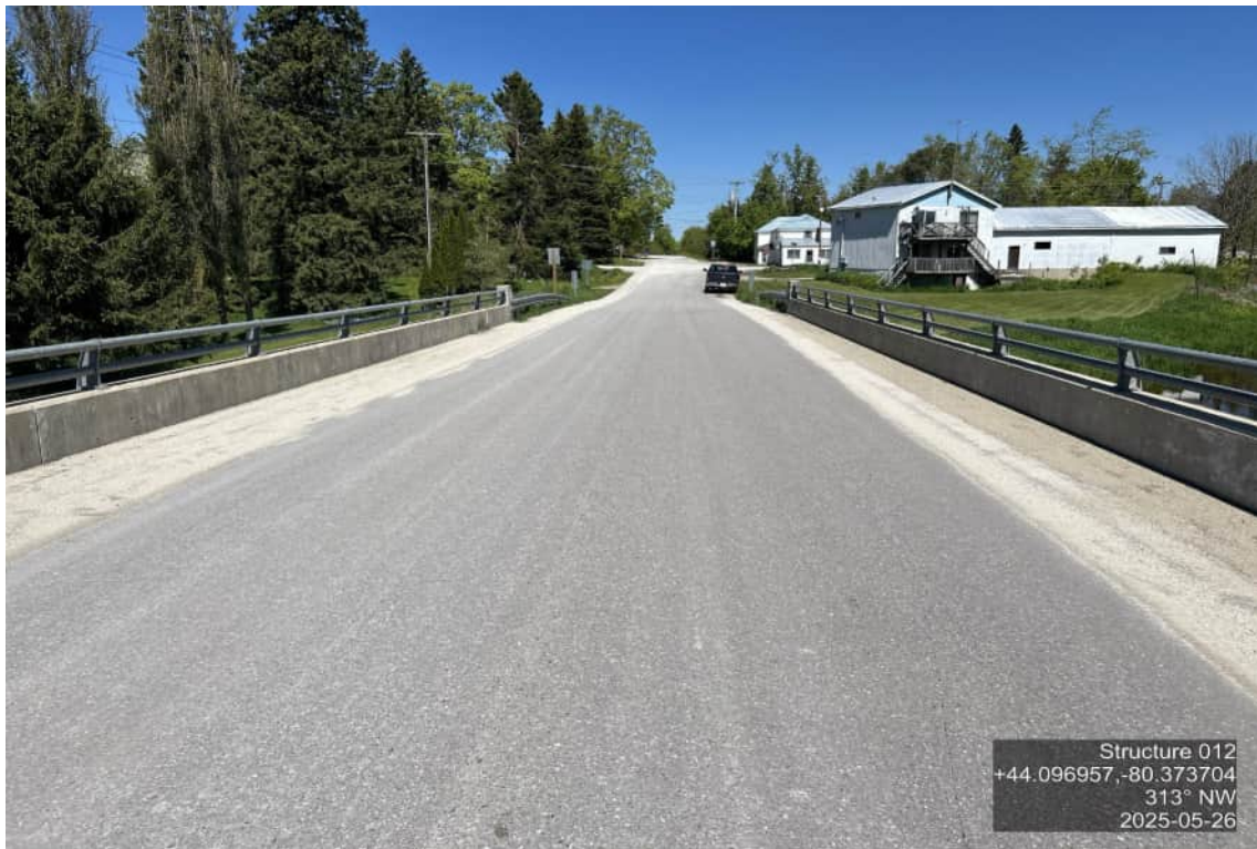
DECK WEARING SURFACE – WEST – GRANULAR ON SHOULDERS
