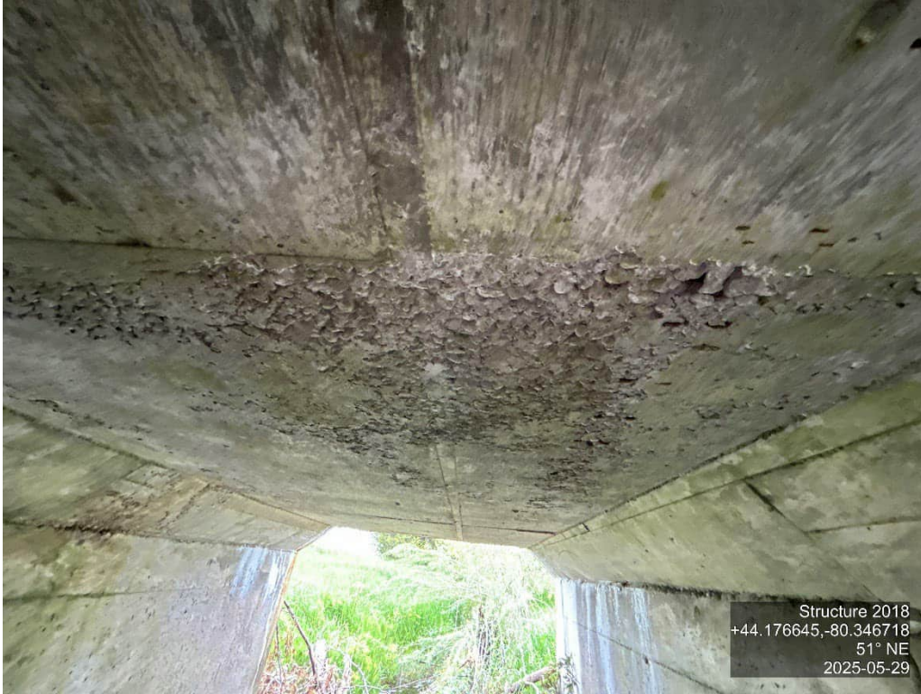
SOFFIT – NORTH – HONEYCOMBING
