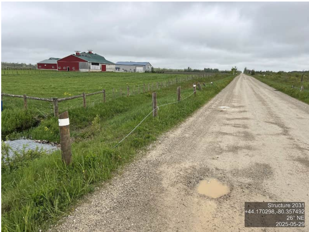
DECK WEARING SURFACE – NORTHEAST – MEDIUM TO LARGE POTHoles
