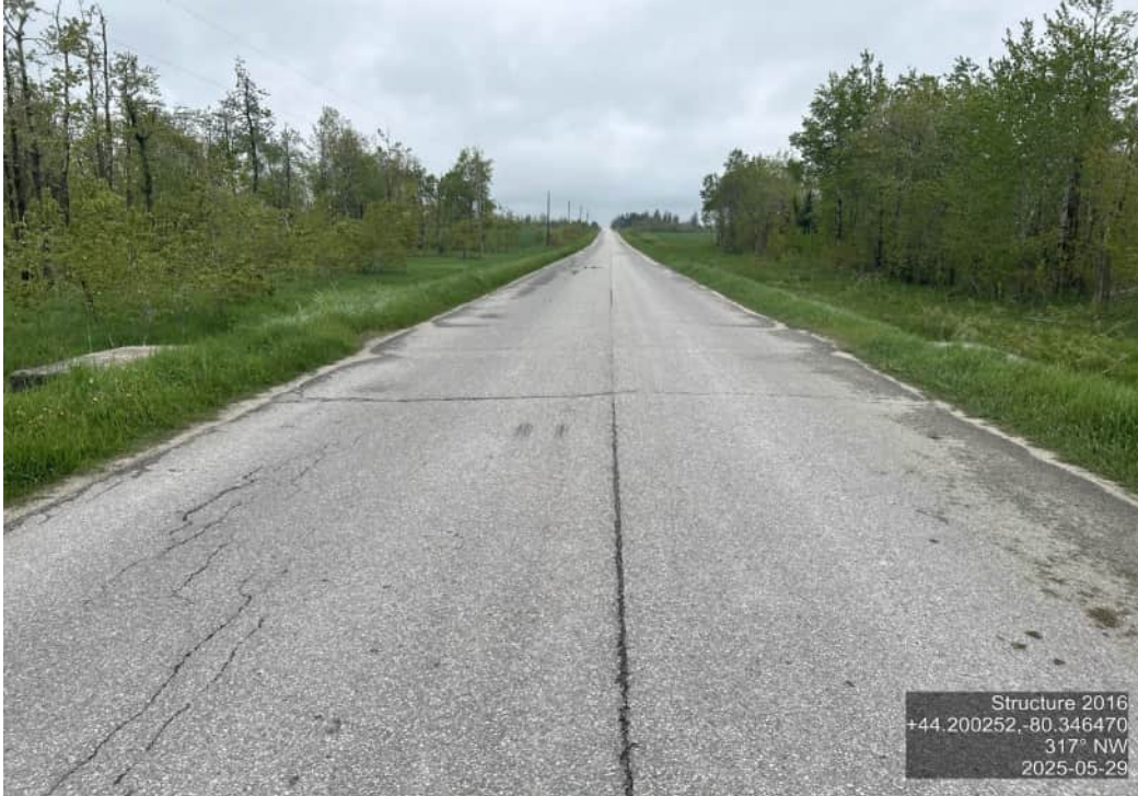
DECK WEARING SURFACE – NORTH – MODERATE SETTLEMENT AT DECK ENDS AND WIDE TRANSVERSE CRACKS
