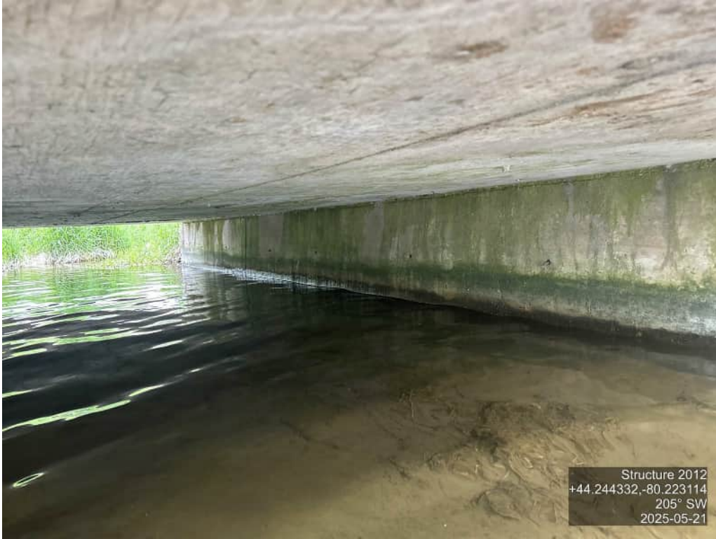
ABUTMENT WALLS – INTERIOR – STAINING AT WATERLINE
