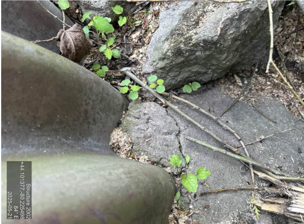
INLET – SOUTHEAST – SPALL
