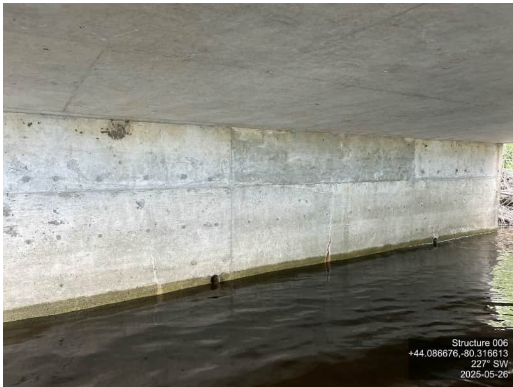
ABUTMENT WALLS – SOUTH – FULL HEIGHT MEDIUM VERTICAL CRACK
