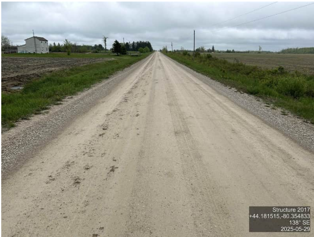
DECK WEARING SURFACE – SOUTHWEST – GRAVEL ON SHOULDERS
