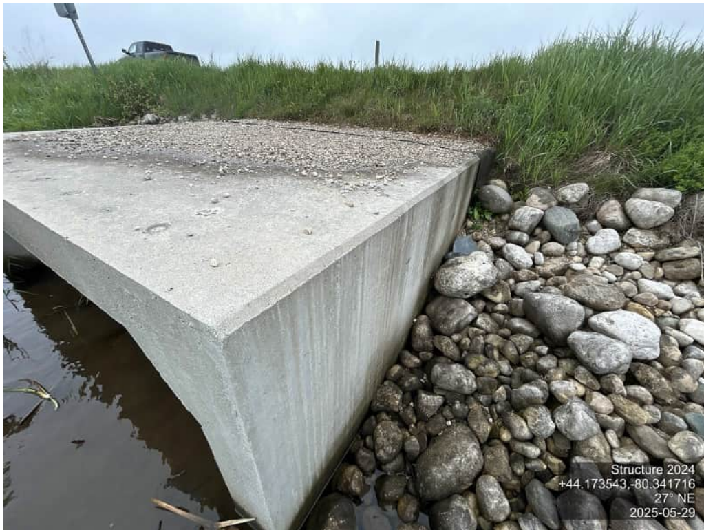
OUTLET – WEST – HAIRLINE STAINED CRACKS
