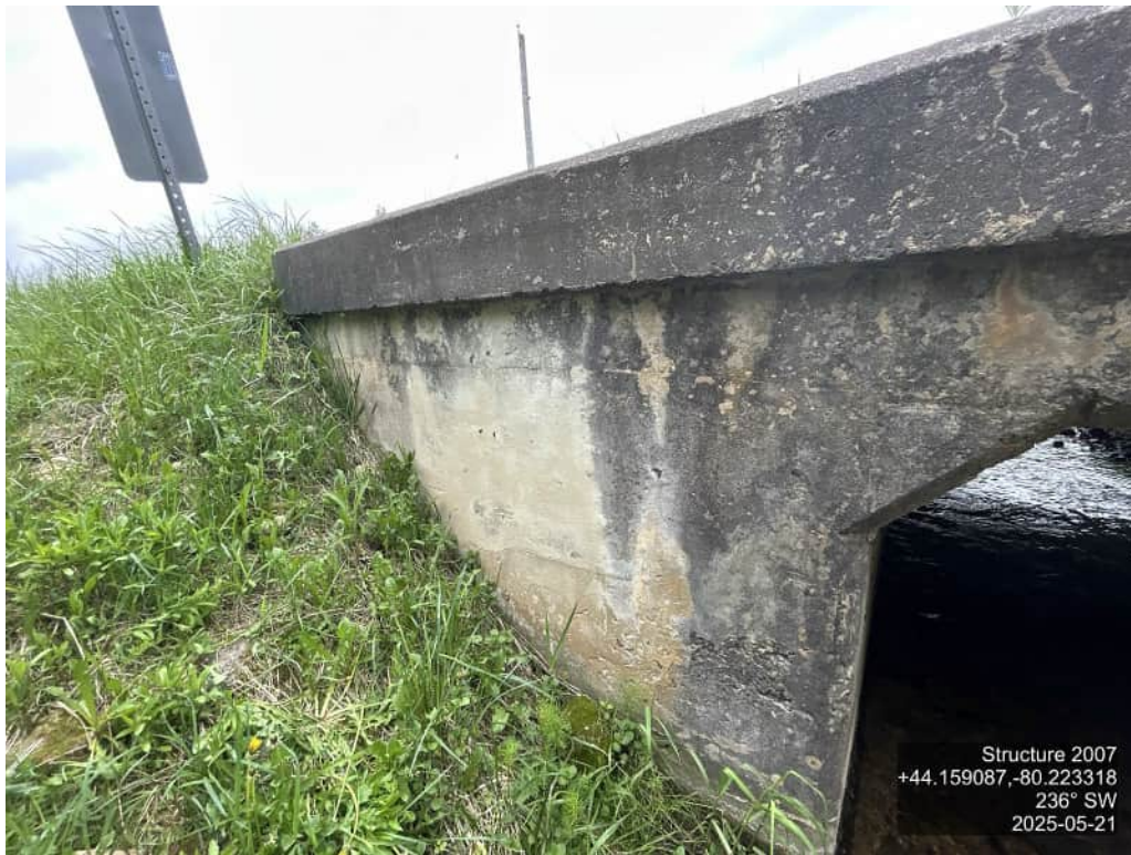
WINGWALL – NORTHWEST – NARROW STAINED CRACKS
