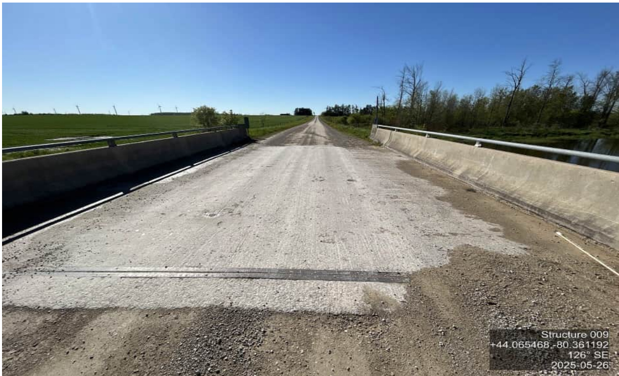
DECK TOP – NORTH – MEDIUM LONGITUDINAL CRACK IN CENTER WITH DELAMINATIONS PRESENT
