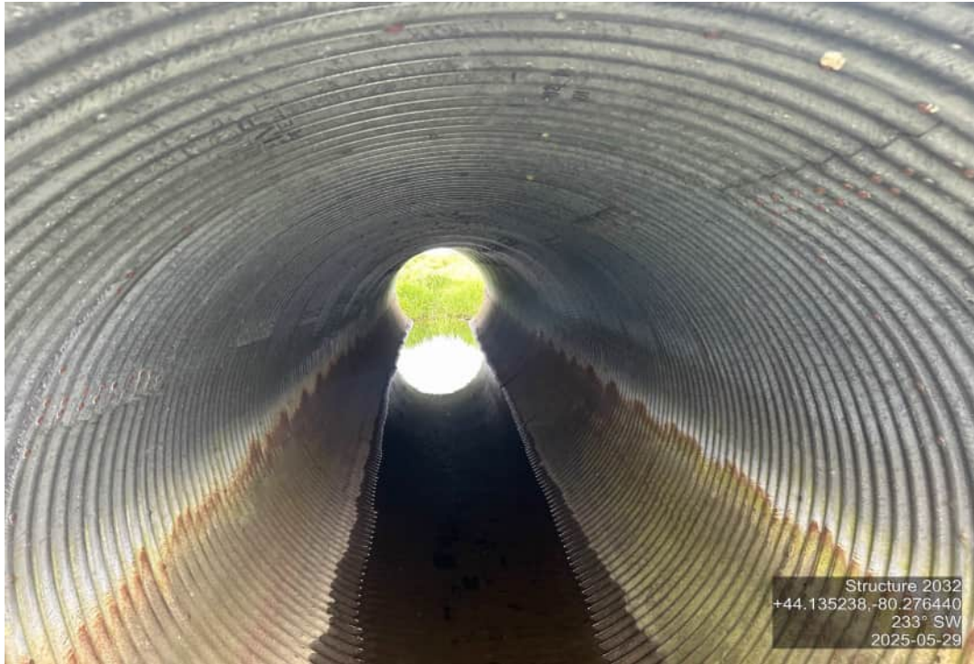
BARREL – NORTH – MODERATE CORROSION, FLAKING AND SECTION LOSS ON FLOOR
