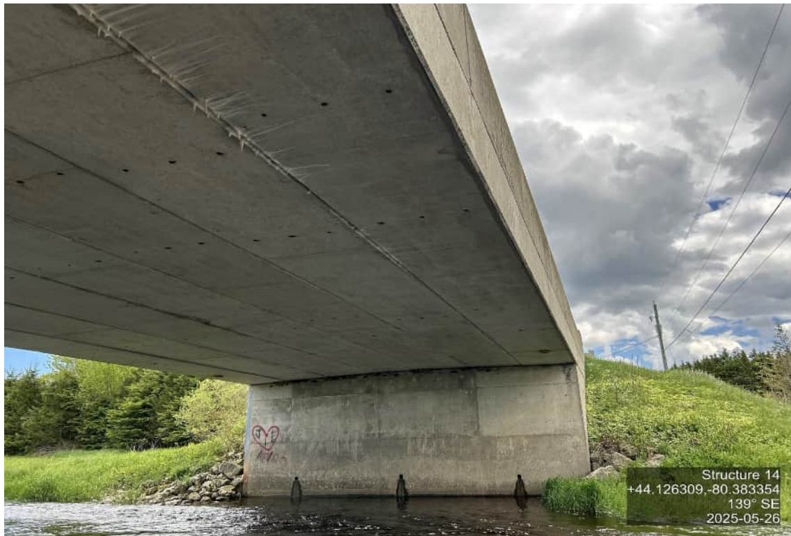
GIRDERS – MIDDLE – STALACTITES AND SIGNS OF WATER PENETRATION
