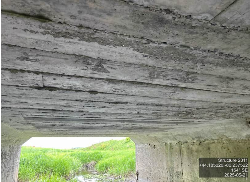
SOFFIT – INTERIOR – SECTIONS OF HONEYCOMBING
