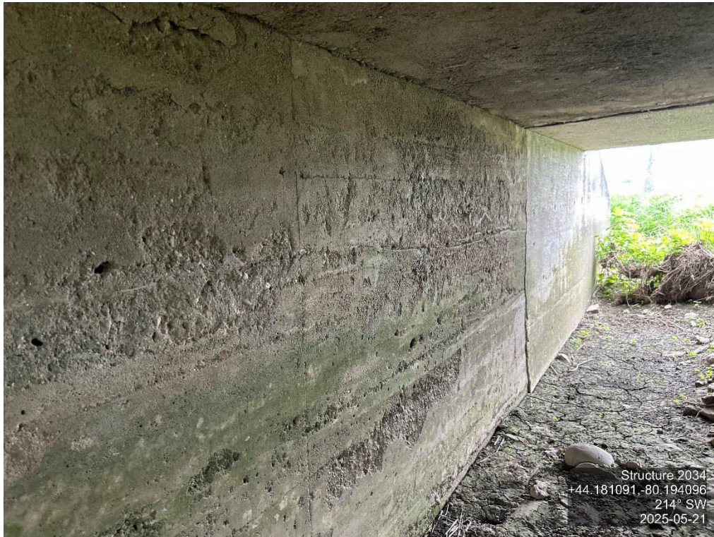
ABUTMENT - SOUTH - MEDIUM SCALING
