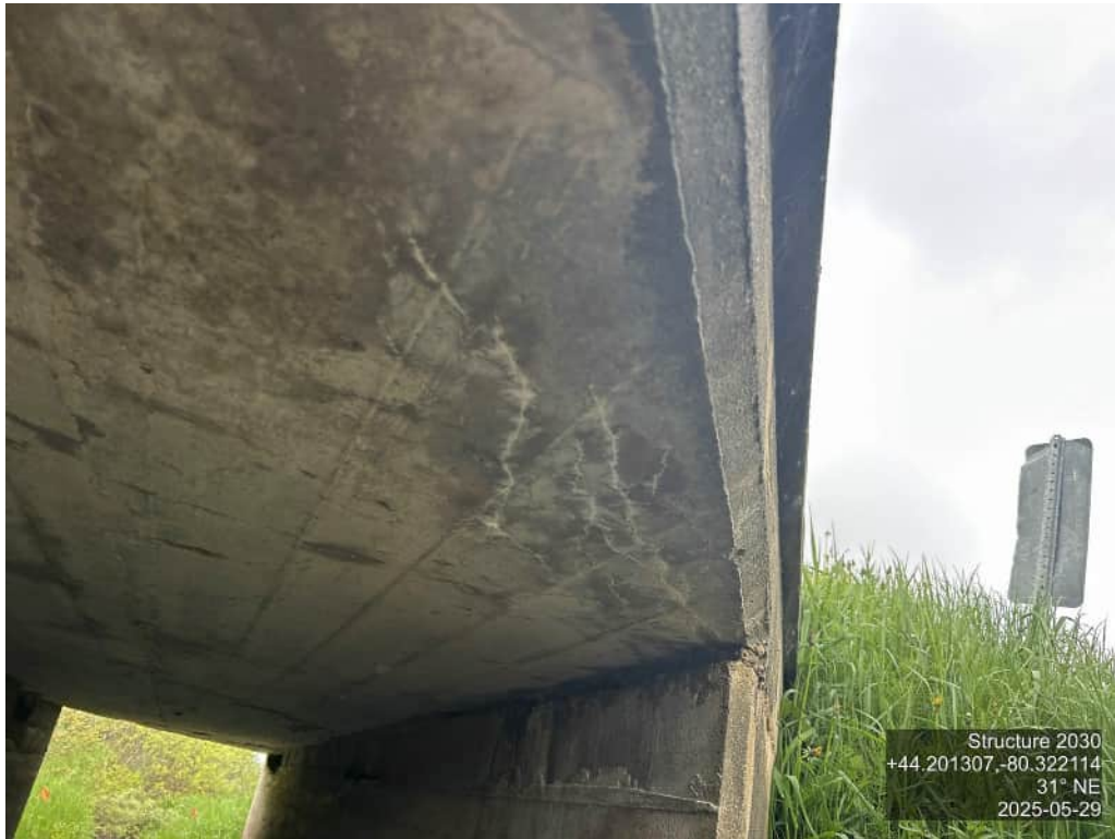
SOFFIT INTERIOR – NORTH – SIGNS OF WATER PENETRATION
