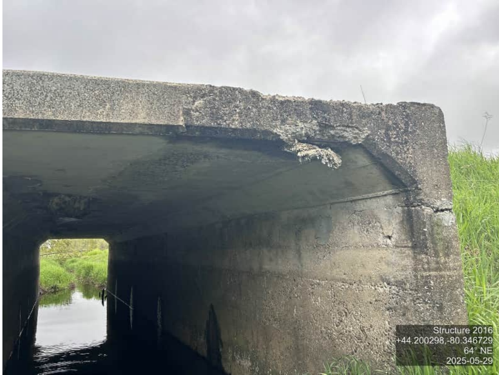
SOFFIT EXTERIOR – EAST – CRACKS AND SPALLING
