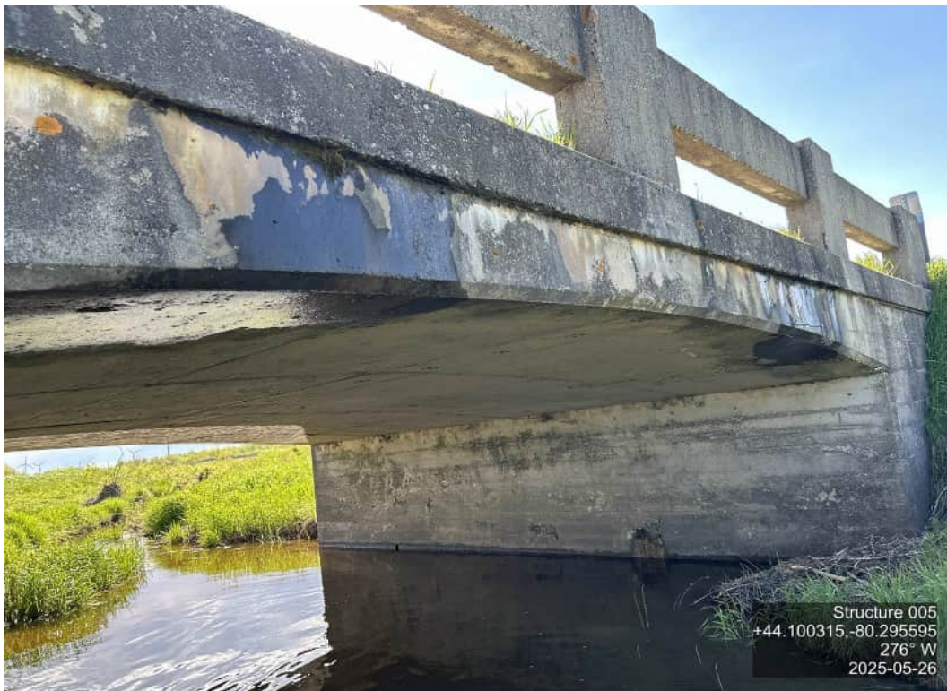
SOFFIT EXTERIOR – WEST – STAINING WITH DELAMINATIONS AND SECTIONS OF MODERATE HONEYCOMBING
