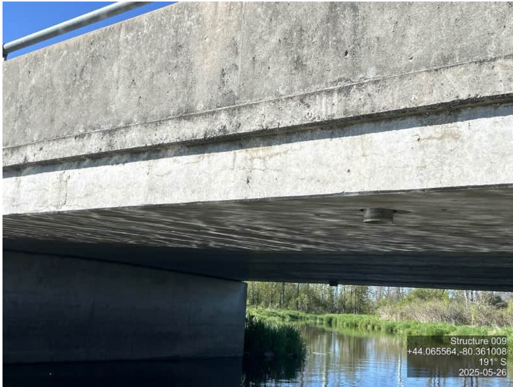
BARRIER WALL EXTERIOR – WEST – NARROW STAINED CRACKS
