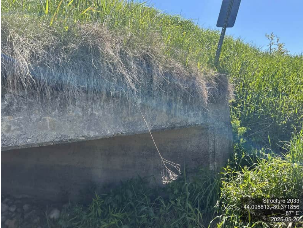
EMBANKMENT – SOUTHEAST – STEEP WITH WASHOUTS ON ALL EMBANKMENTS
