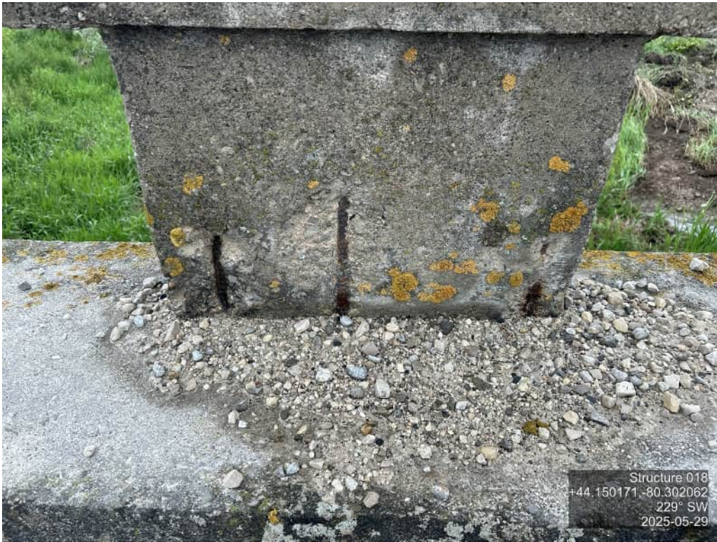
POSTS – INTERIOR – SPALLS WITH EXPOSED CORRODED REBAR
