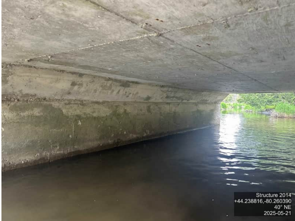
ABUTMENT WALLS – INTERIOR – SEVERE SCALING AND HONEYCOMBING
