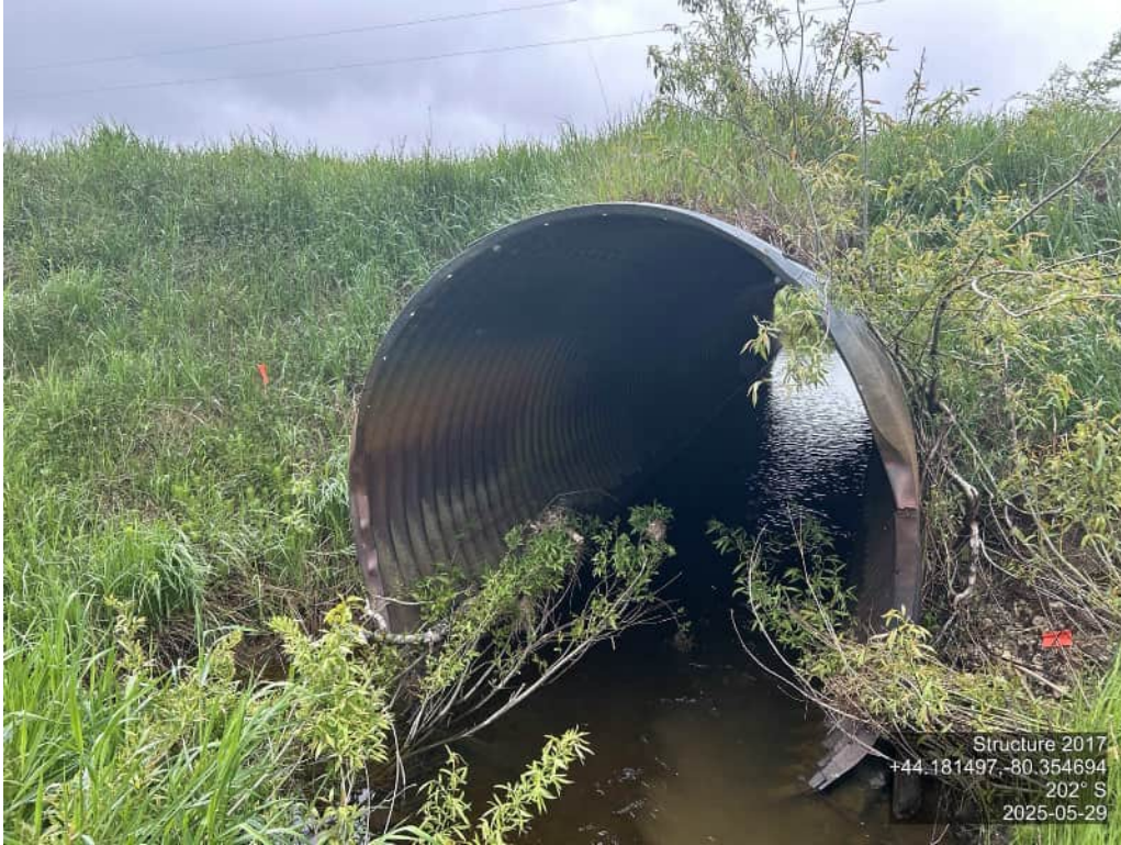
EMBANKMENT – EAST – SEVERE WASHOUTS
