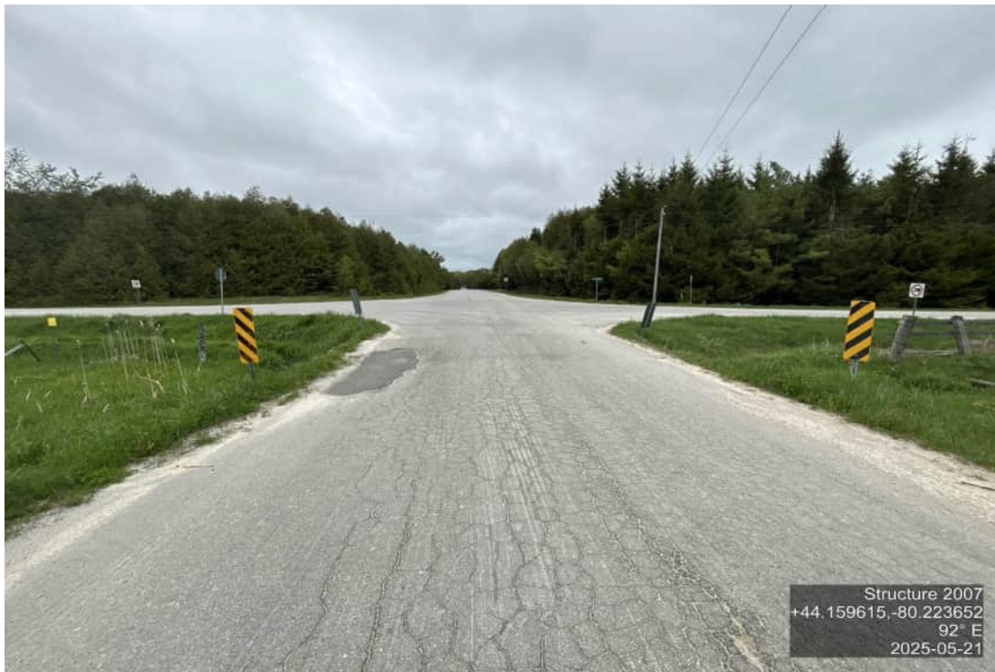
DECK WEARING SURFACE– NORTH – LONGITUDINAL CRACKING THROUGHOUT
