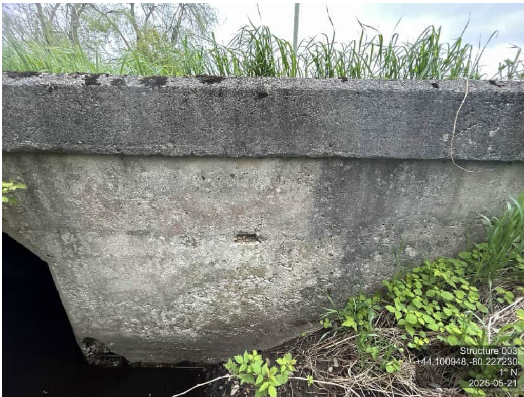
WINGWALL – NORTHEAST – SEVERE SPALL WITH EXPOSED CORRODED REBAR
