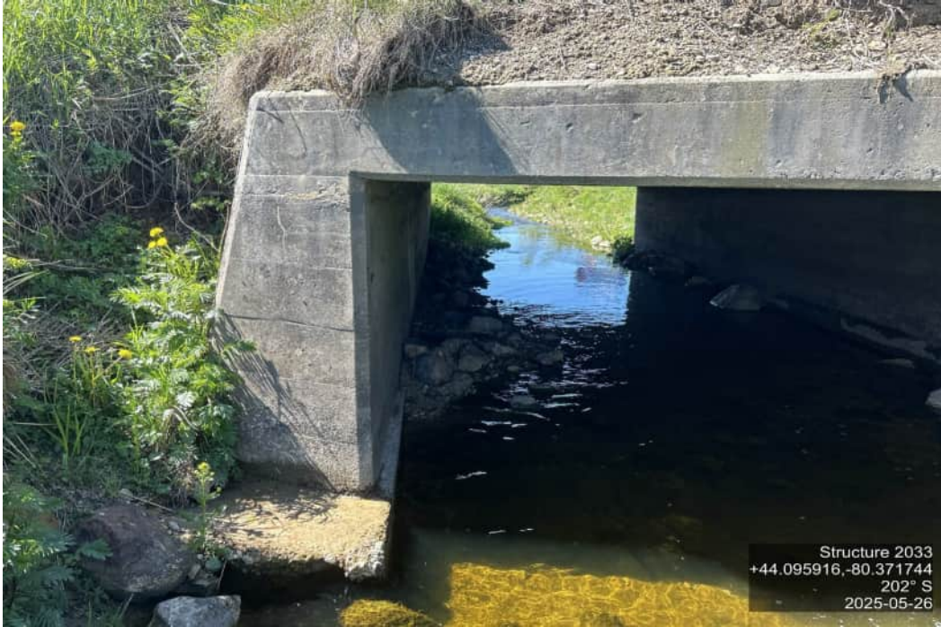
INLET – SOUTHEAST – EXPOSED FOOTING, LARGE AMOUNT OF FILL ON CULVERT ENDS
