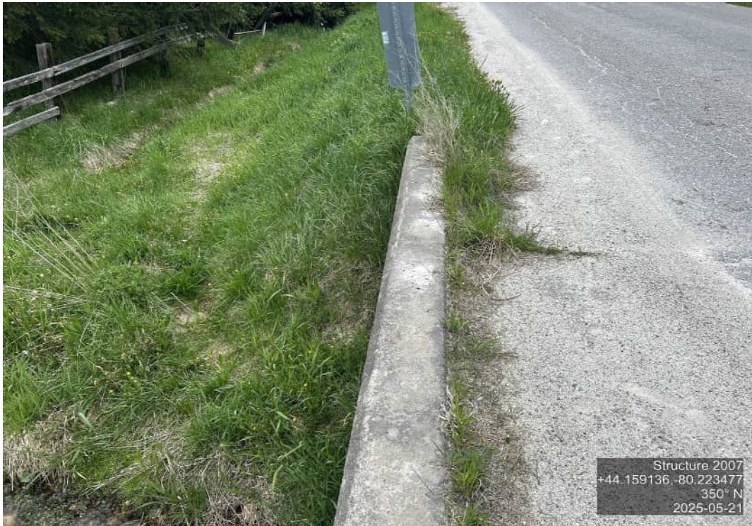
CURB – WEST – SMALL SPALLS
