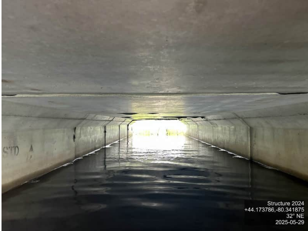
BARREL – INTERIOR – GAP BETWEEN JOINTS
