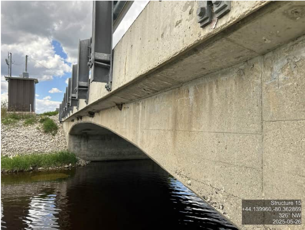
SOFFIT EXTERIOR – WEST – LIGHT DELAMINATIONS
