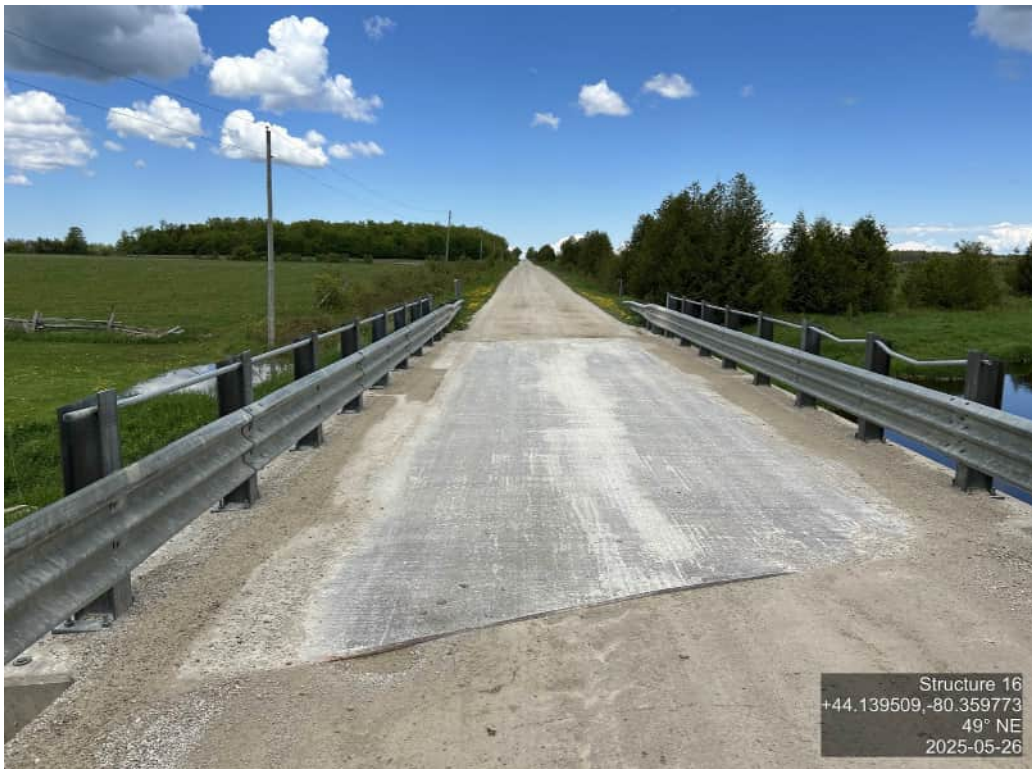
DECK TOP – NORTHEAST – GRAVEL TRACKED ONTO DECK ENDS
