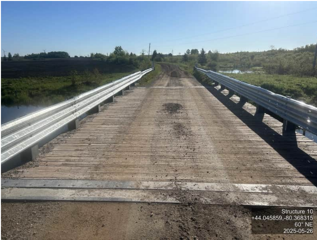
DECK TOP – EAST – LIGHT SPLITS AND WEATHERING
