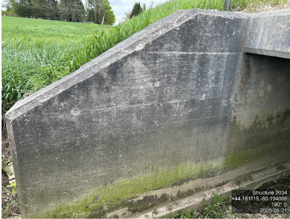
WINGWALL- SOUTHWEST - MOISTURE STAINING
