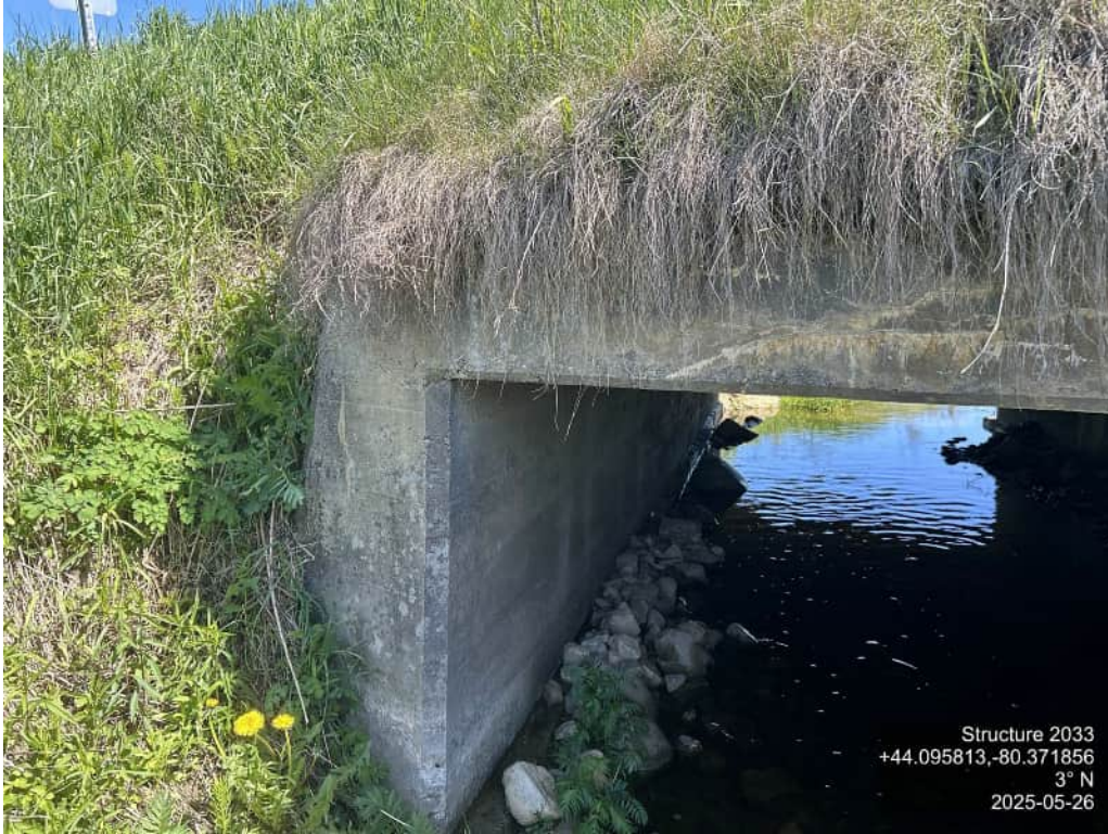
OUTLET – WEST – MEDIUM SIZED EFFLORESCENCE STAINED CRACKS
