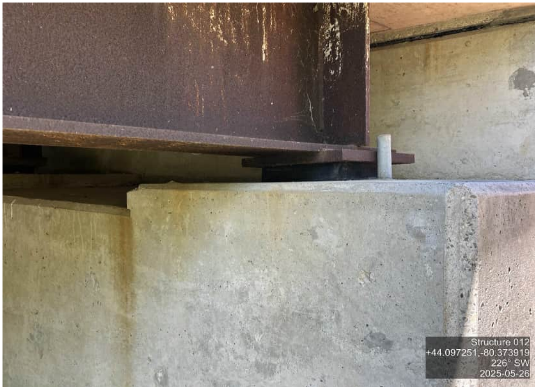
BEARING PADS – SOUTHEAST – LIGHT BULGING
