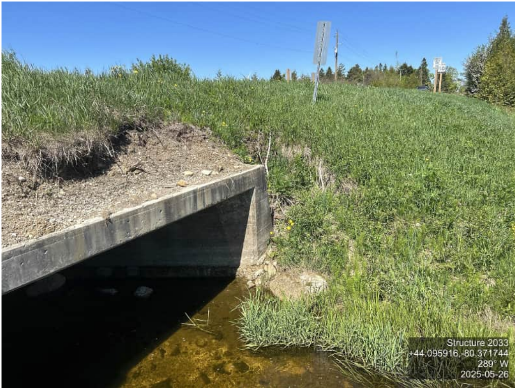
STREAM – NORTHWEST – ERROSION AT CORNERS OF STRUCTURE
