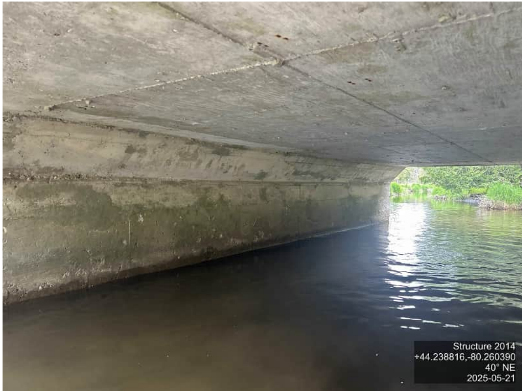
SOFFIT – INTERIOR – LIGHT HONEYCOMBING
