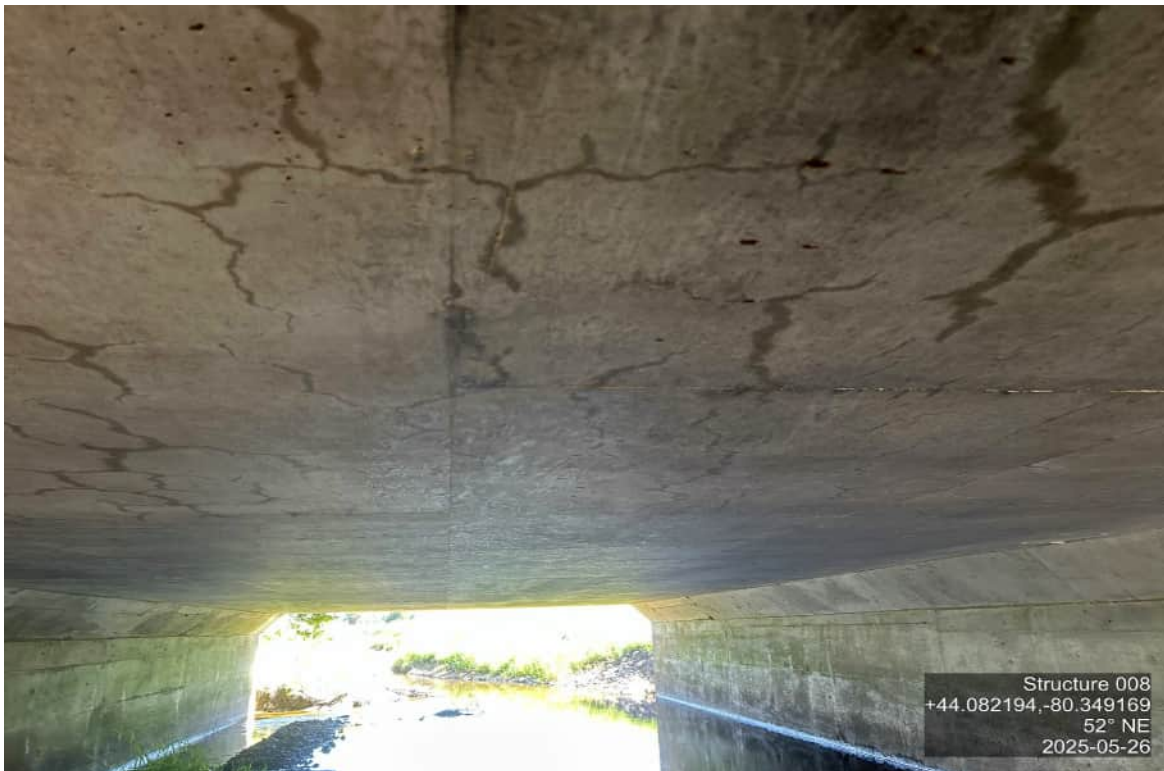
BARREL – INTERIOR – MOISTURE PENETRATION CRACKING
