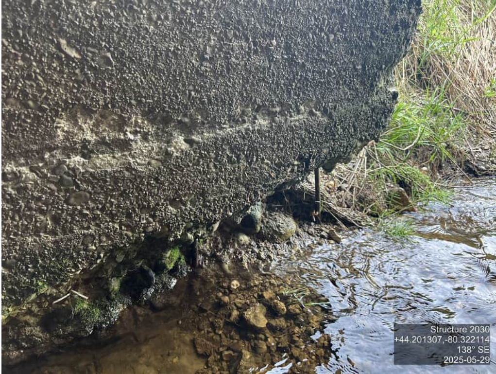
EMBANKMENT – NORTHWEST – SEVERE EROSION AT WATERLINE
