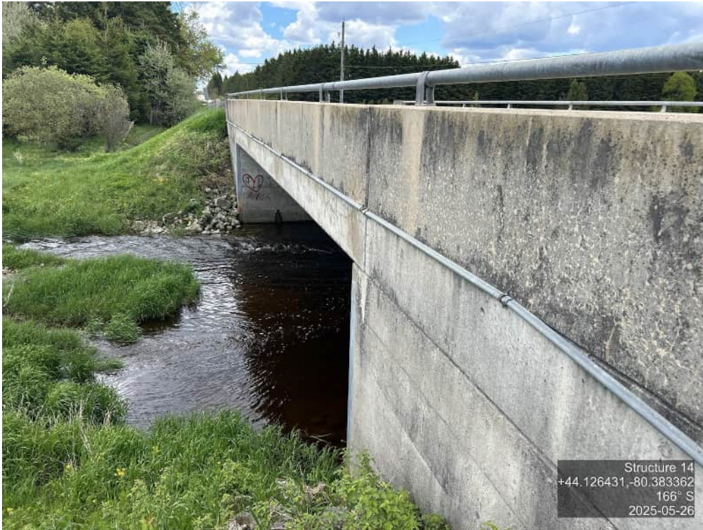
BARRIER WALLS EXTERIOR – EAST – NARROW STAINED CRACKS
