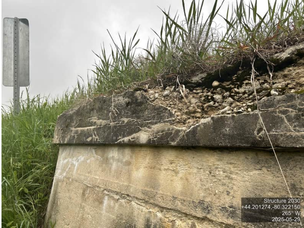
CURB – NORTHEAST – SPALLING AND DELAMINATIONS
