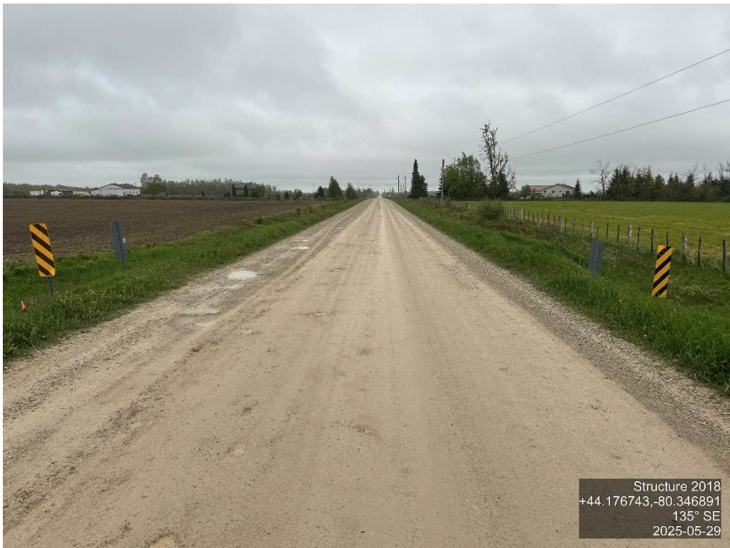
DECK WEARING SURFACE – WEST – SMALL POTHOLES
