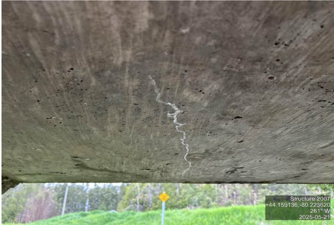
SOFFIT INTERIOR – WEST – HONEYCOMBING AND SCALING
