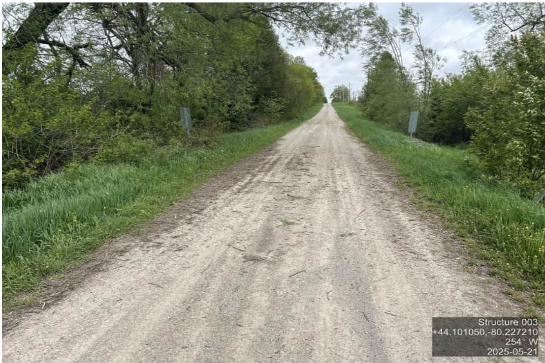
DECK WEARING SURFACE – EAST – SMALL POTHoles
