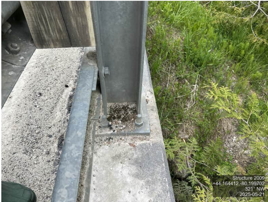
CURB – NORTHWEST – POUR VIBRATION AROUND BASE PLATES
