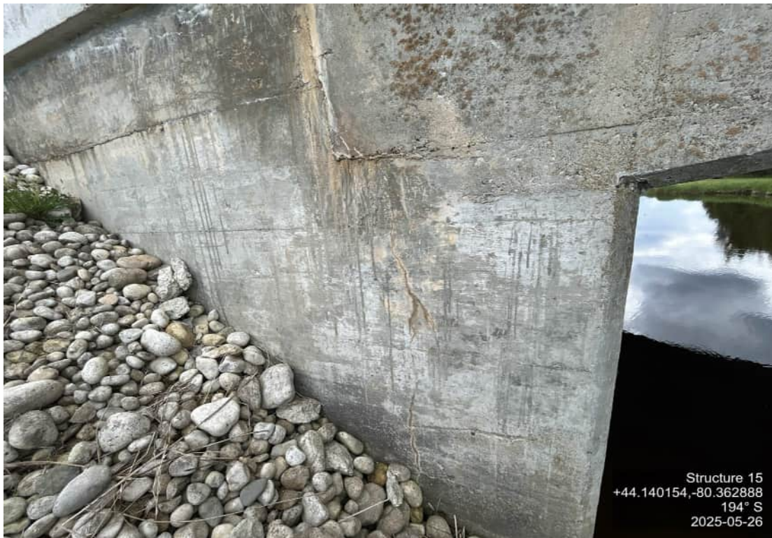
WINGWALL – SOUTHWEST – DELAMINATIONS AND STAINED CRACKS
