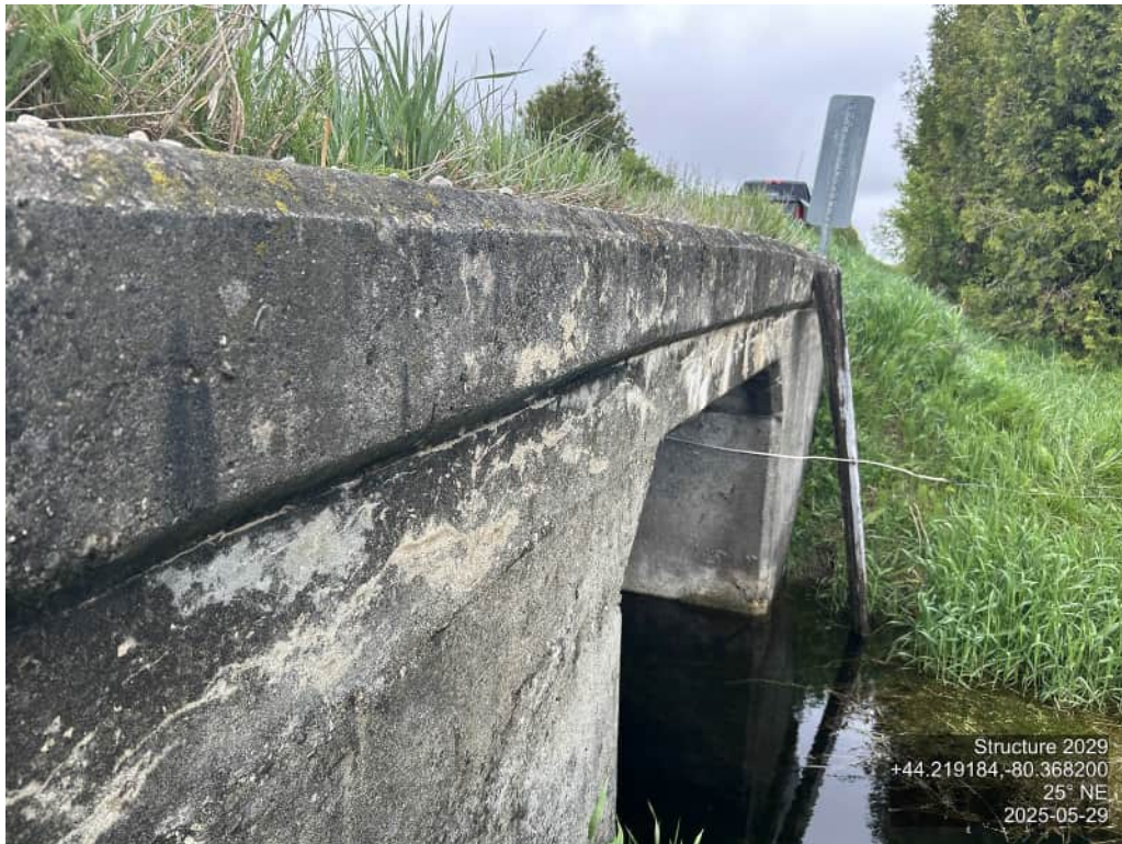
WINGWALLS – NORTHEAST – HONEYCOMBING AND CRACKS THROUGHOUT
