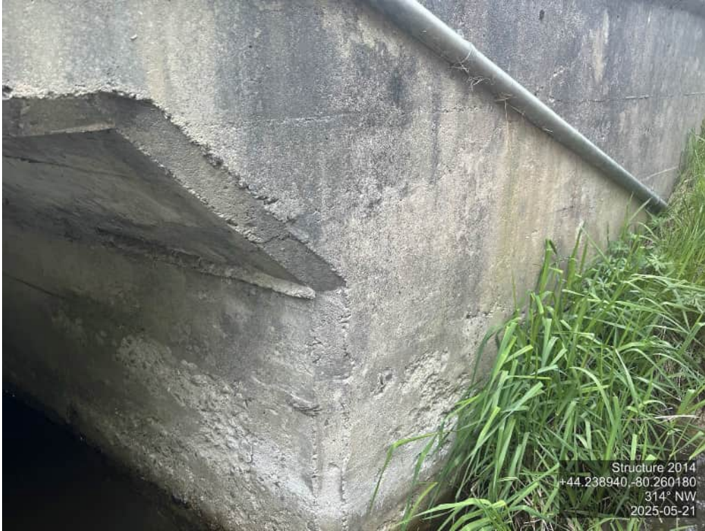
EMBANKMENT – SOUTHWEST - EROSION
