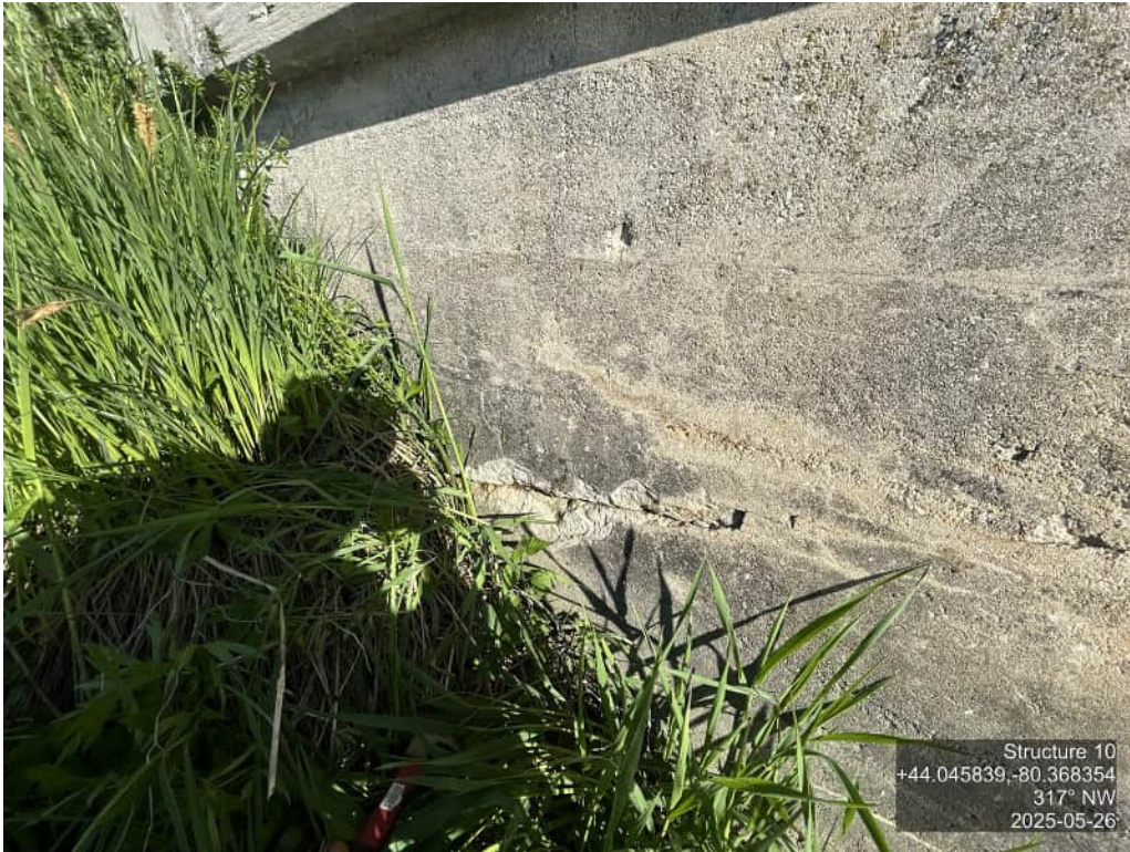
WINGWALL – SOUTHEAST – MEDIUM CRACK
