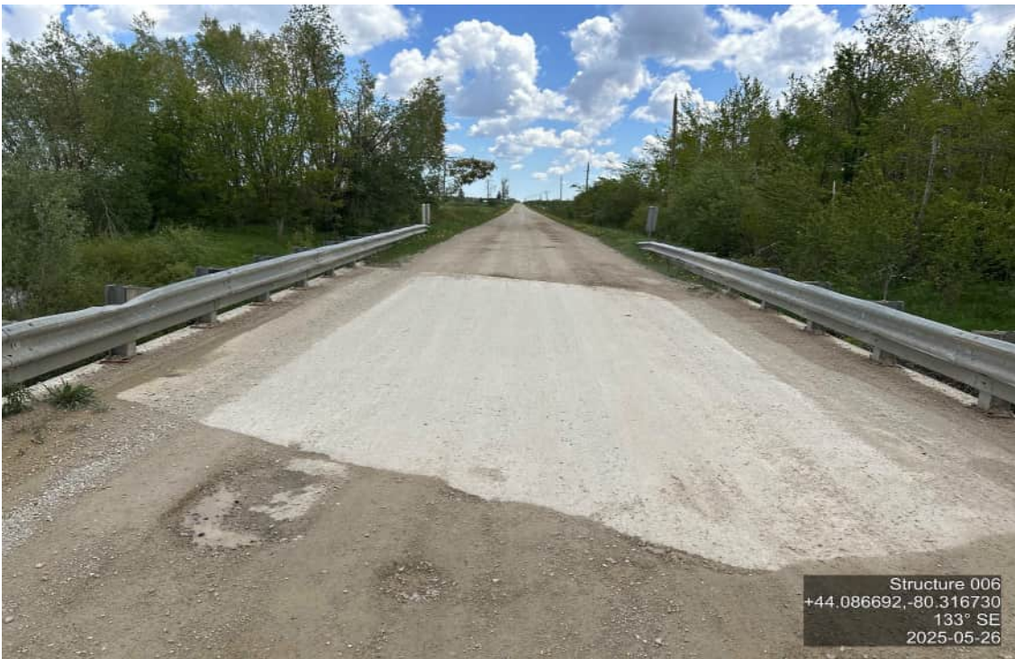
APPROACH WEARING SURFACE – NORTH APPROACH – SEVERAL LARGE POTHLES
