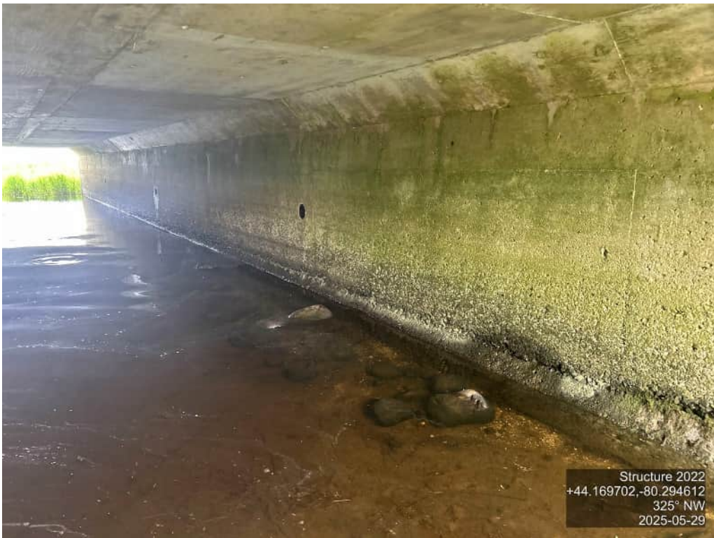
BARREL – EAST – HONEYCOMBING, SCALING AND WIDE CRACKS AT HAUNCH
