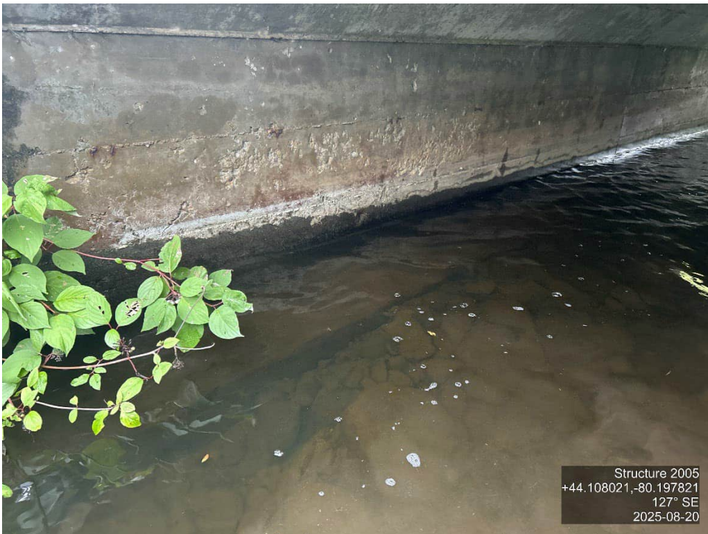
ABUTMENT- EAST – EXPOSED FOOTING
