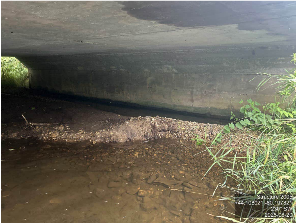
WATERCOURSE – SEDIMENT BUILDUP
