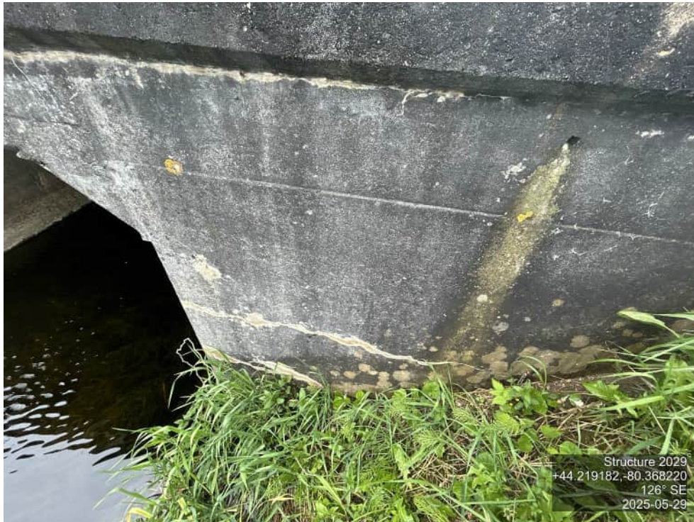
SOFFIT EXTERIOR – LOCATION – HAIRLINE CRACKING AND STAINING WITH EFFLORESCENCE
