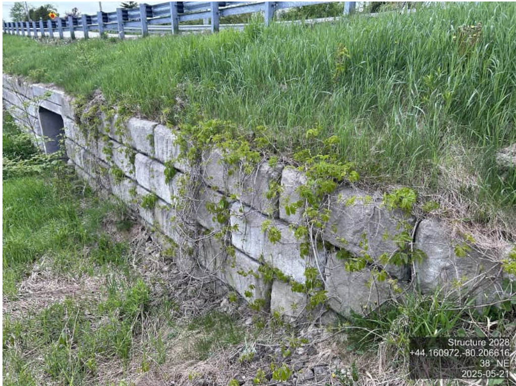
RETAINING WALLS – NORTHWEST – VEGETATION GROWING OVER WALL
