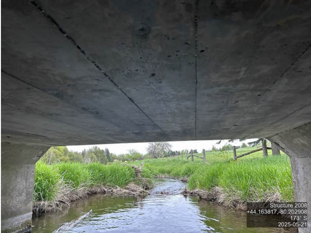
SOFFIT INTERIOR – SOUTH – LIGHT HONEYCOMBING AND DELAMINATIONS
