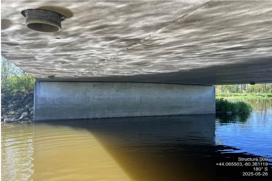
ABUTMENT WALLS – SOUTH – LIGHT HONEYCOMBING
