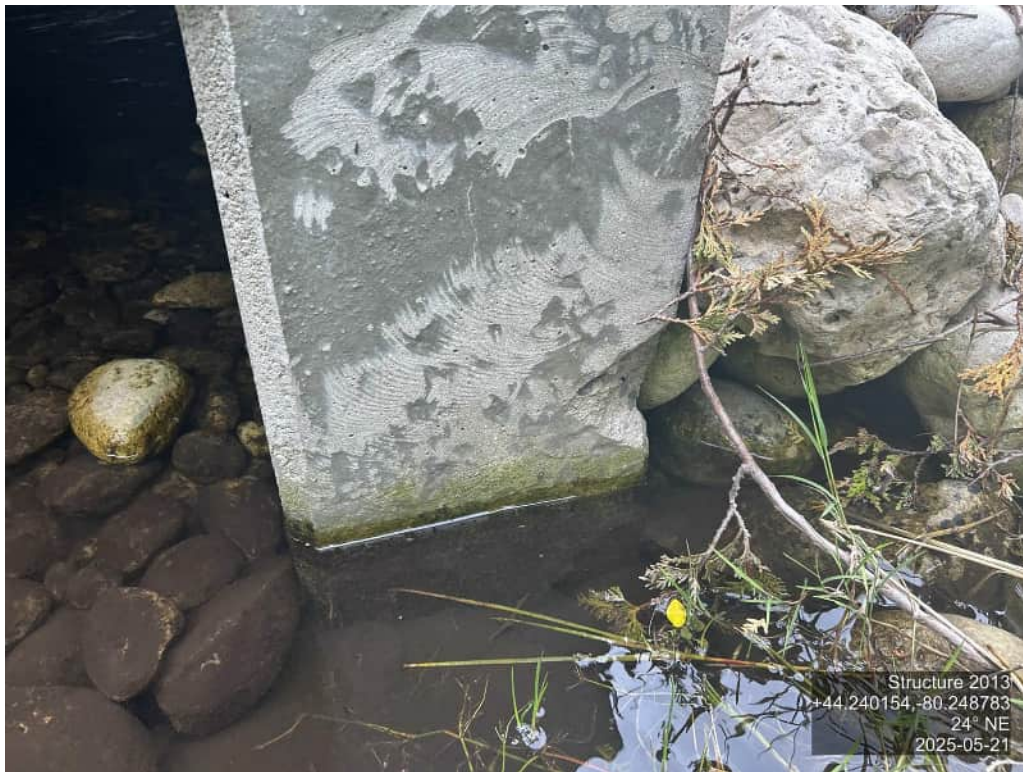
OUTLET – NORTH – SMALL SPALL
