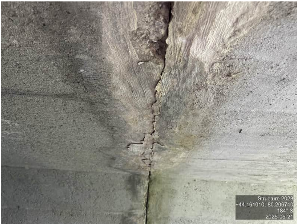
BARREL – INSIDE WALLS – FAILED PARING AT JOINT WITH WATER PENETRATION
